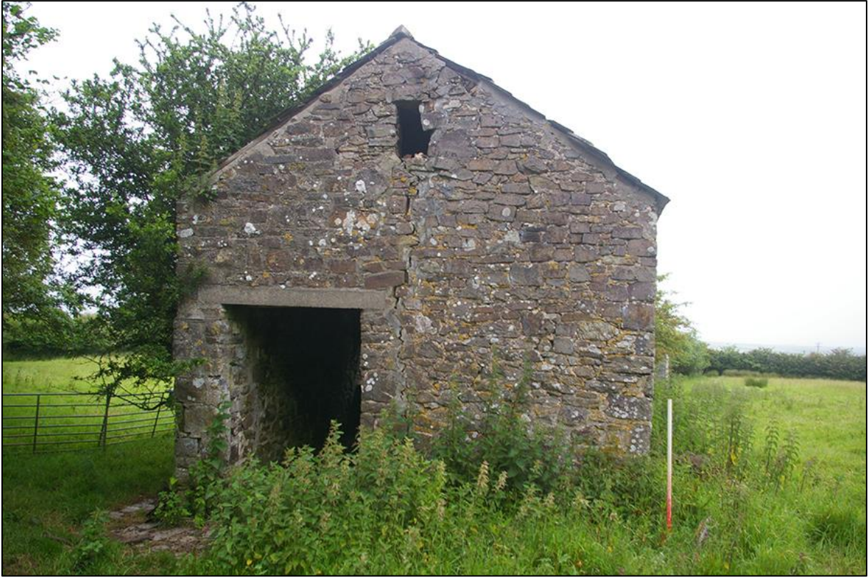
5. SOUTH ELEVATION OF THE STONE-BUILT STRUCTURE IN THE SOUTH-WESTERN CORNER OF F1; VIEWED FROM THE SOUTH (1M SCALE).
