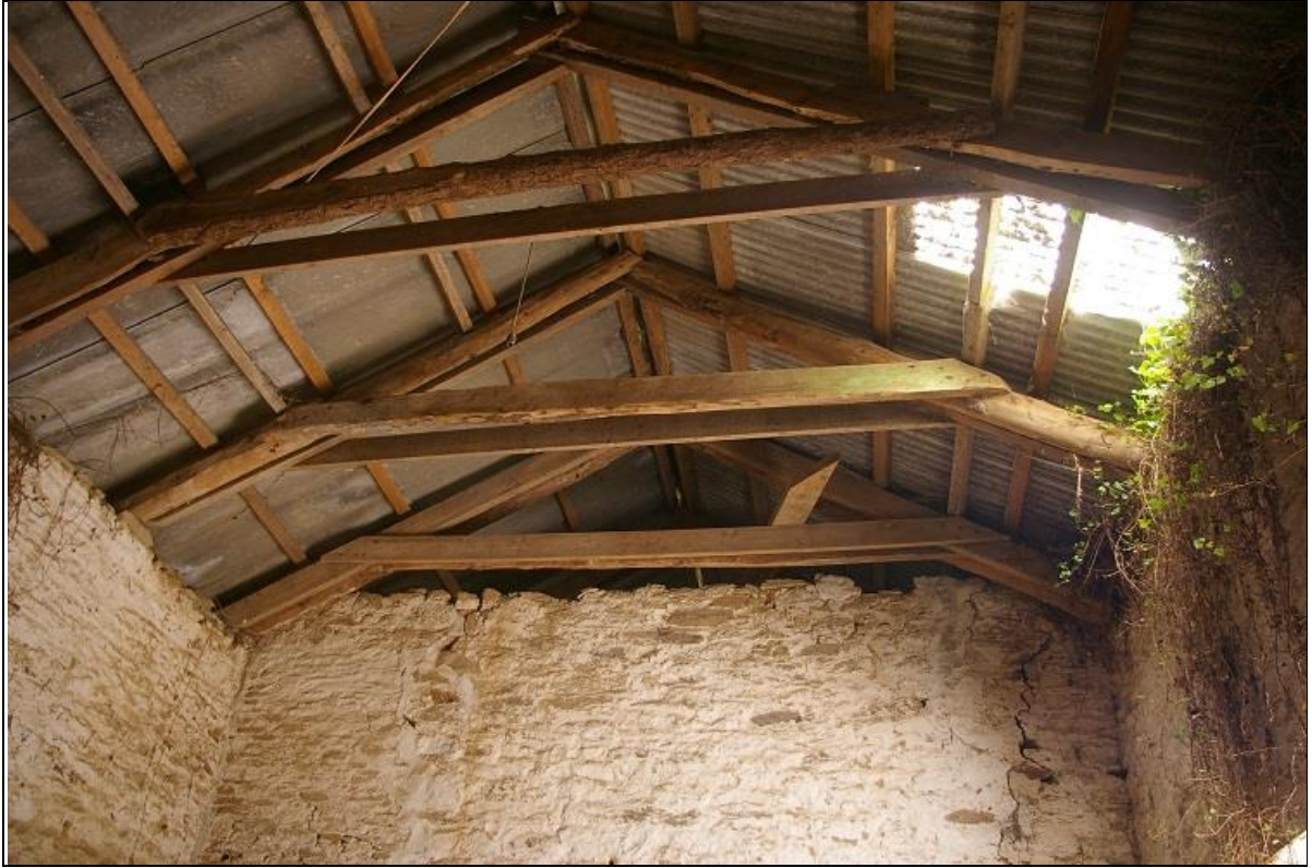
23. THE ROUGH EMBARKED TRUSSES OVER INFILL STRUCTURE BUILDING C, OF BARN RANGE 2, CLEARLY OF A POORER QUALITY THAN SOME OF THE OTHER 18 TH CENTURY BUILDINGS; FROM THE SOUTH-EAST.
