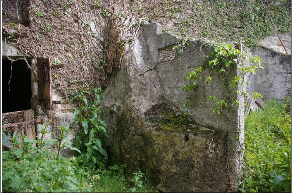
15. PROJECTING WALL STUB ON THE FRONT OF BARN RANGE 4; FROM THE SOUTH-WEST.
