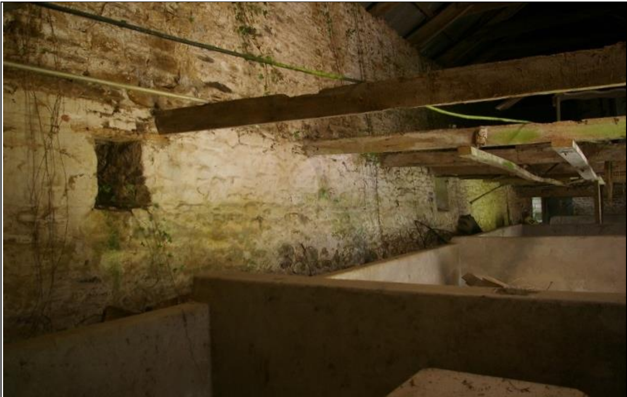
18. THE BACK WALL OF BARN RANGE 3, SHOWING DIFFERENT BATTERED BUILD TO THE LOWER PART OF THE WALL, WITH MODERN CONCRETE PENS; FROM THE SOUTH-EAST.
