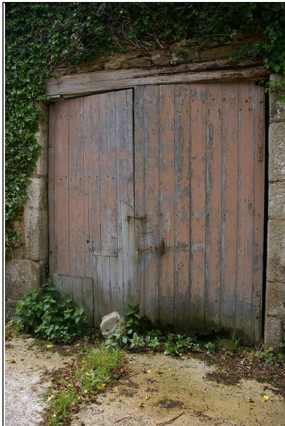
20. THE LARGE PLANK BOARDED DOORS TO BUILDING C, BARN RANGE 2; FROM THE NORTH-EAST.
