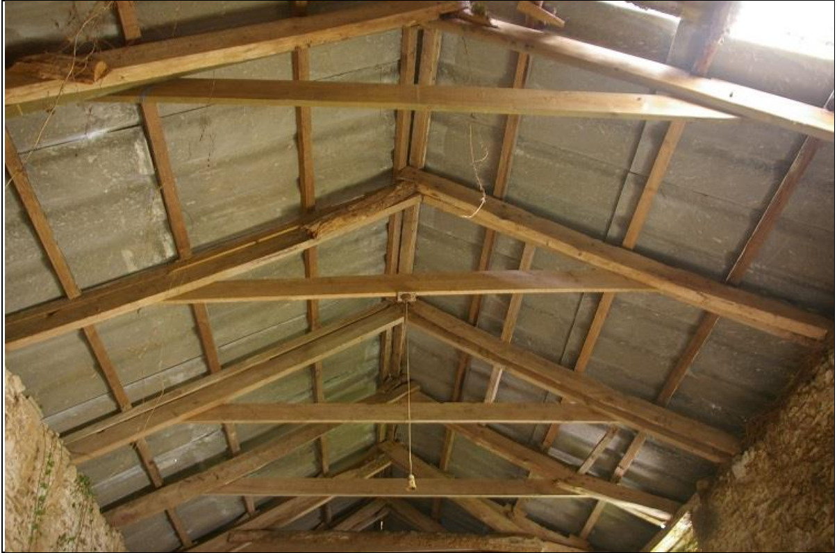
19. THE ROOF OVER BARN RANGE 3, THE ELM TRUSSES HAVE LARGELY FAILED, REPLACED WITH 20 TH CENTURY PINE AND CORRUGATED SHEETING; FROM THE SOUTH.
