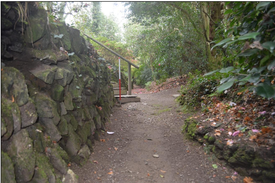
FIGURE 145: STEPS HAVE BEEN INSERTED INTO THE VERTICAL FACE OF THE HA-HA TO PERMIT ACCESS. FROM THE WEST
