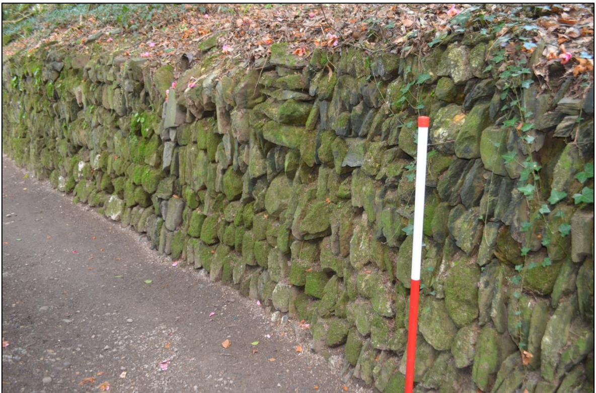
FIGURE 149: THE BUILD FORM OF THE CURVED SECTION OF THE HA-HA APPEARS TO BE CONTIGUOUS WITH THE STRAIGHT SECTION ALTHOUGH IT SEEMS LIKELY THAT REPAIRS HAVE BEEN MADE TO THE UPPER SECTIONS OF THE WALL.
