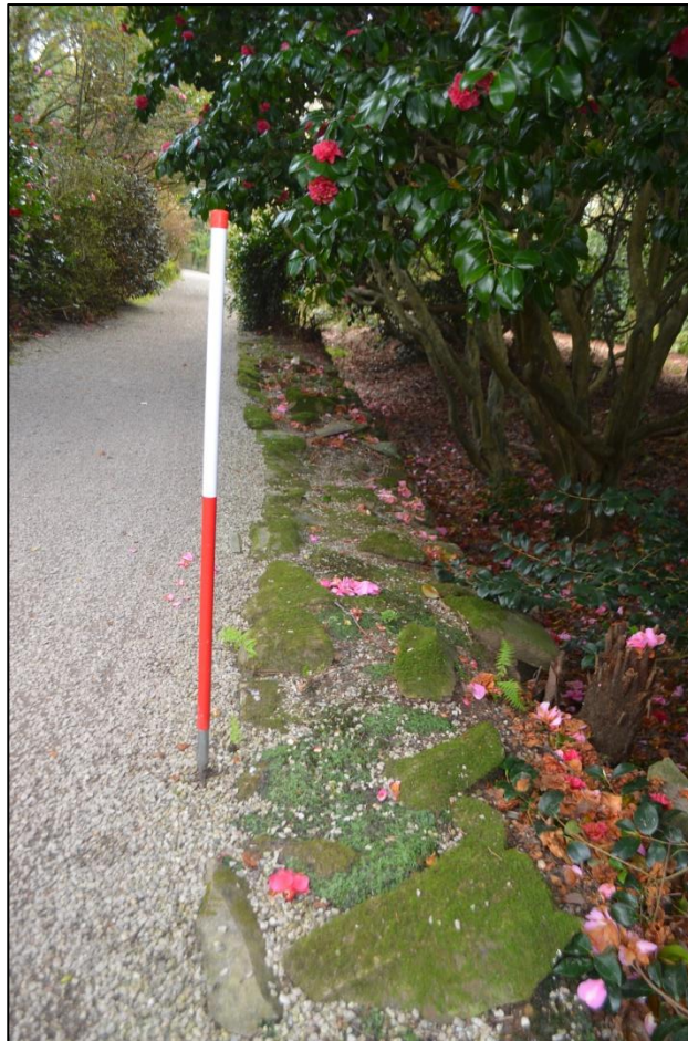
FIGURE 60: EXPOSED STONE SECTION AT THE TOP OF A HA-HA IN THE SOUTH EAST OF THE PLEASURE GARDENS. FROM THE NORTH
