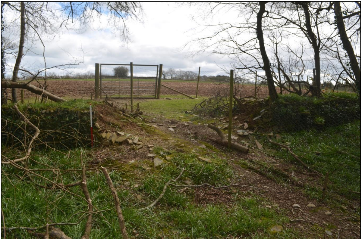
FIGURE 102: RECENT BREACH IN BOUNDARY 11 AT ITS SOUTHERN END.
