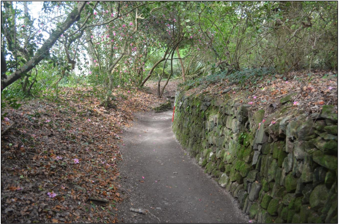
FIGURE 146: THE HA-HA CURVES AROUND AT ITS WESTERN END, THIS ALIGNS WITH THE BOUNDARY SHOWN ON THE 1747 PLAN. FROM THE EAST
