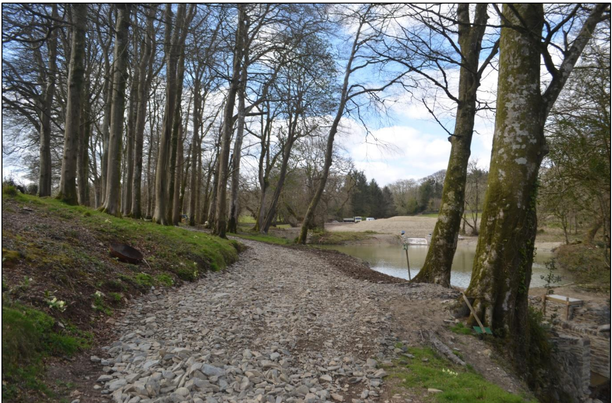
FIGURE 38: RENOVATION WORKS TAKING PLACE IN THE WEST OF THE EAGLE PONDS VALLEY. FROM THE EAST
