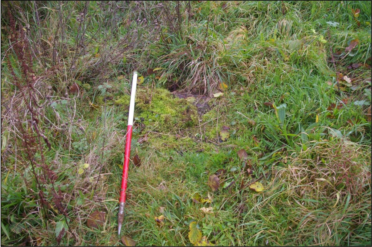
9. DETAIL OF MAN-HOLE COVER IN F2; VIEWED FROM THE WEST-NORTH-WEST (1M SCALE).
