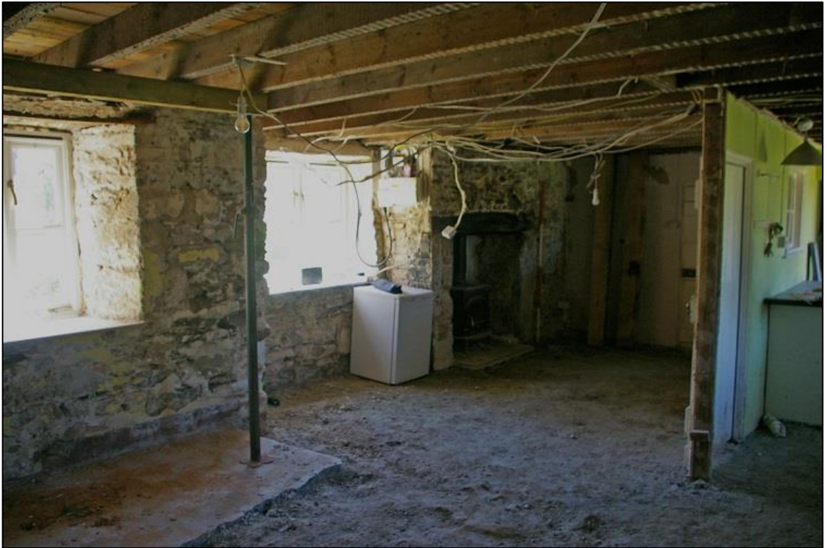
3. THE FRONT WALL OF THE COTTAGE, FORMERLY KNOWN AS NO.2, WITH LATERAL STACK (2M SCALE); FROM THE NORTH-WEST.
