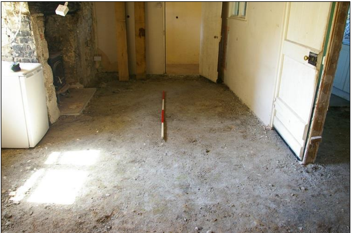
FIGURE 4: THE SOUTH END OF THE ROOM, WITH LATERAL STACK TO THE FRONT WALL AND MODERN PARTITION WALL FORMING THE KITCHEN; FROM THE NORTH-NORTH-WEST (2M SCALE).
