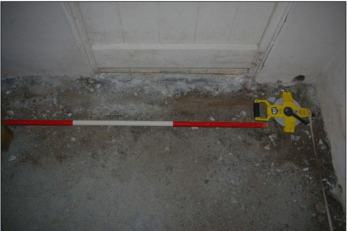
FIGURE 8: BROWN LIMECRETE FLOOR AND A FEW SPLIT SLATE LINEAR COBBLES IN THE DOORWAY TO THE HALL, ALONGSIDE THE PLANK PARTITION, AS WELL AS THE CONCRETE FLOOR IN THE HALLWAY VISIBLE ABOVE; FROM THE NORTH (2M SCALE).
