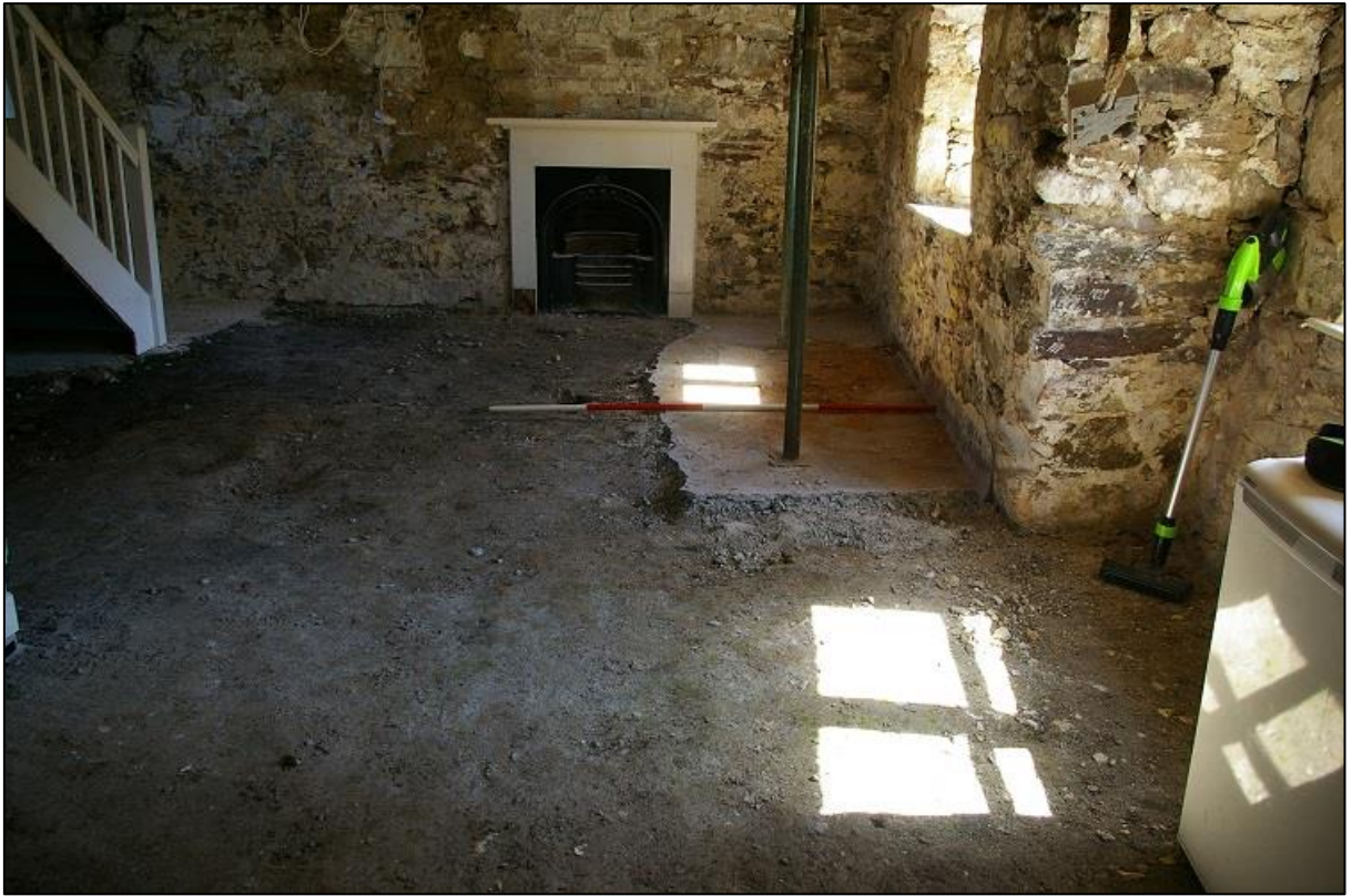
FIGURE 3: THE NORTH END OF THE ROOM, WITH PARTIAL CONCRETE FLOOR REMAINING AND POST MEDIEVAL FIREPLACE, LIKELY POST 1800; FROM THE SOUTH-SOUTH-EAST (2M SCALE).
