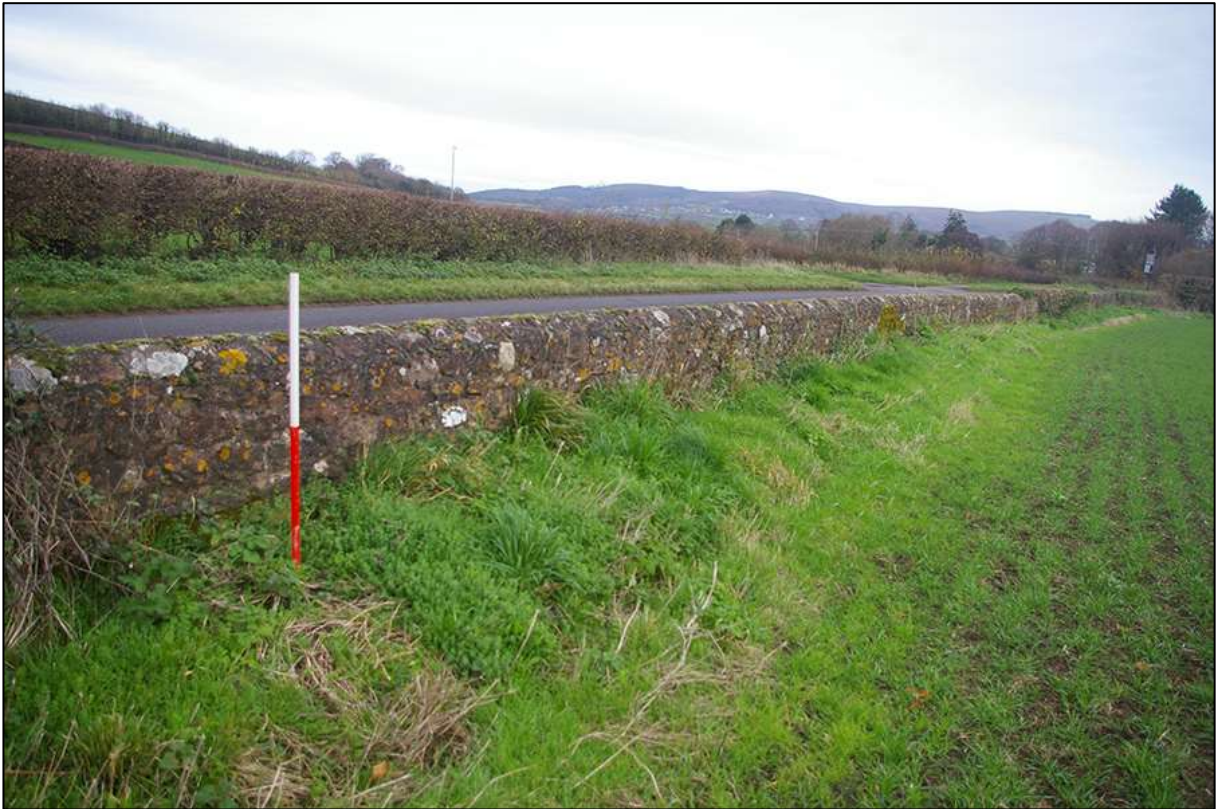
5. DETAIL OF THE NORTHERN ROADSIDE WALL BOUNDARY TO FIELD F1; VIEWED FROM THE WEST-NORTH-WEST (1M SCALE).
