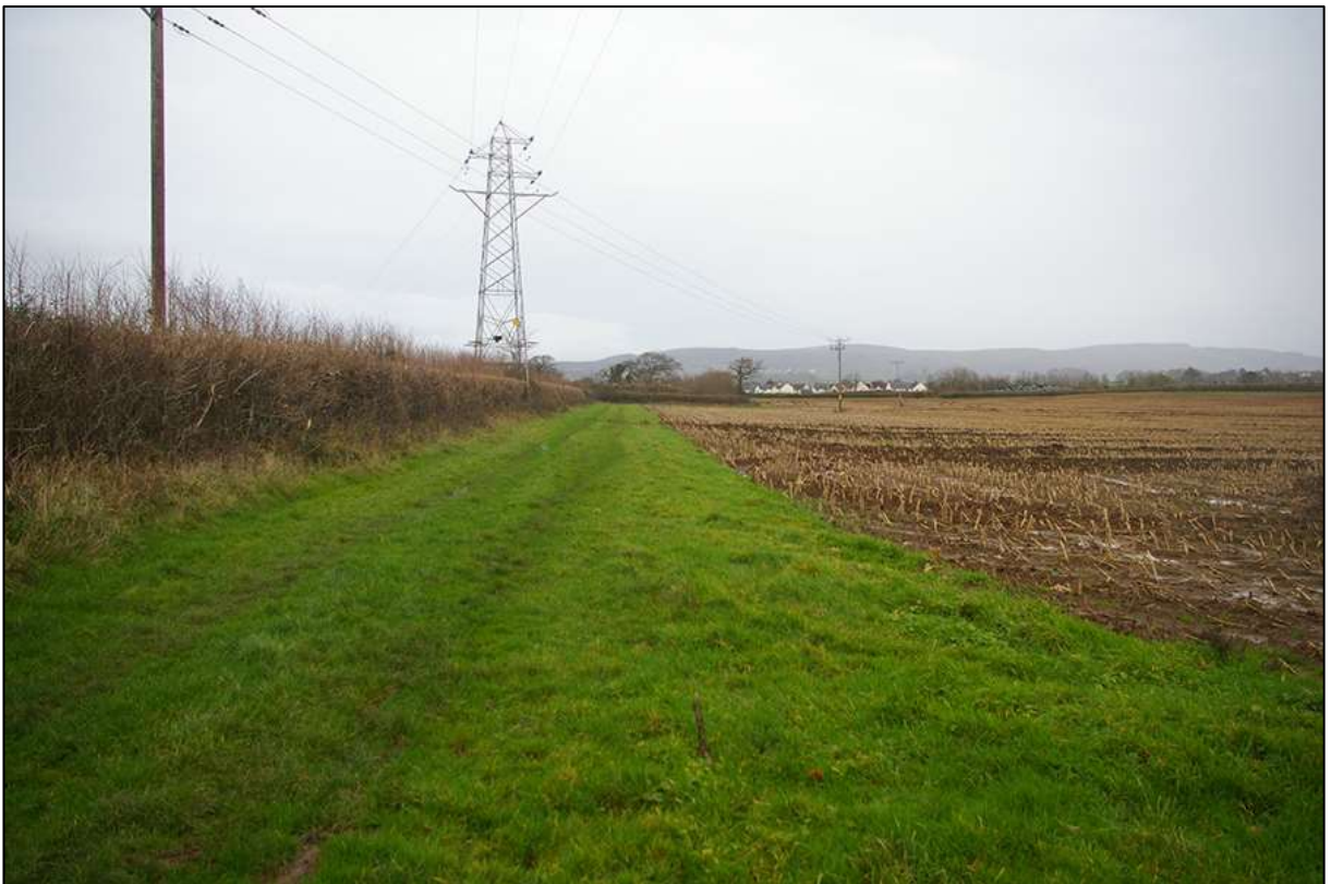
64. VIEW ALONG THE NORTHERN EDGE OF FIELD F10 SHOWING DETAIL OF THE PYLONS AND OVERHEAD CABLES; VIEWED FROM THE WEST (NO SCALE).
