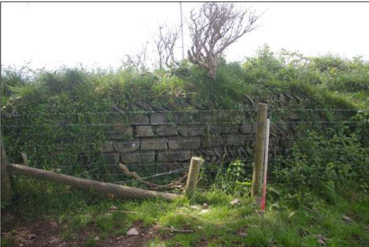
6. DETAIL OF MODERN REPAIRS TO THE SOUTHERN BOUNDARY; VIEWED FROM THE NORTH (1M SCALE).
