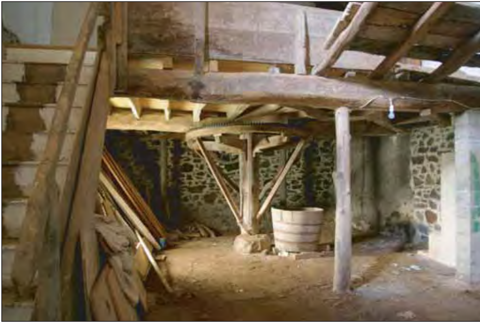
Plate 3: The interior of the Cider Barn viewed from the north, after clearance of debris.
