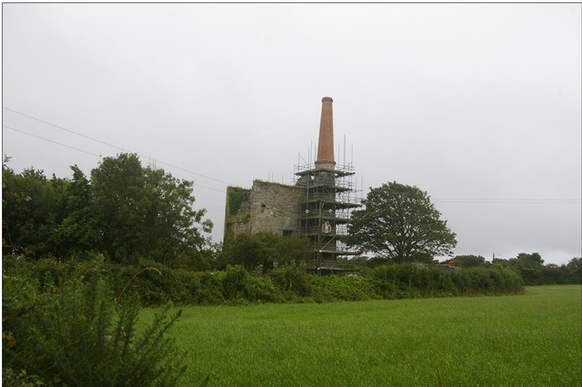
FIGURE 15: THE ENGINE HOUSE AND CHIMNEY AT IVEY'S SHAFT; VIEWED FROM THE NORTH.
