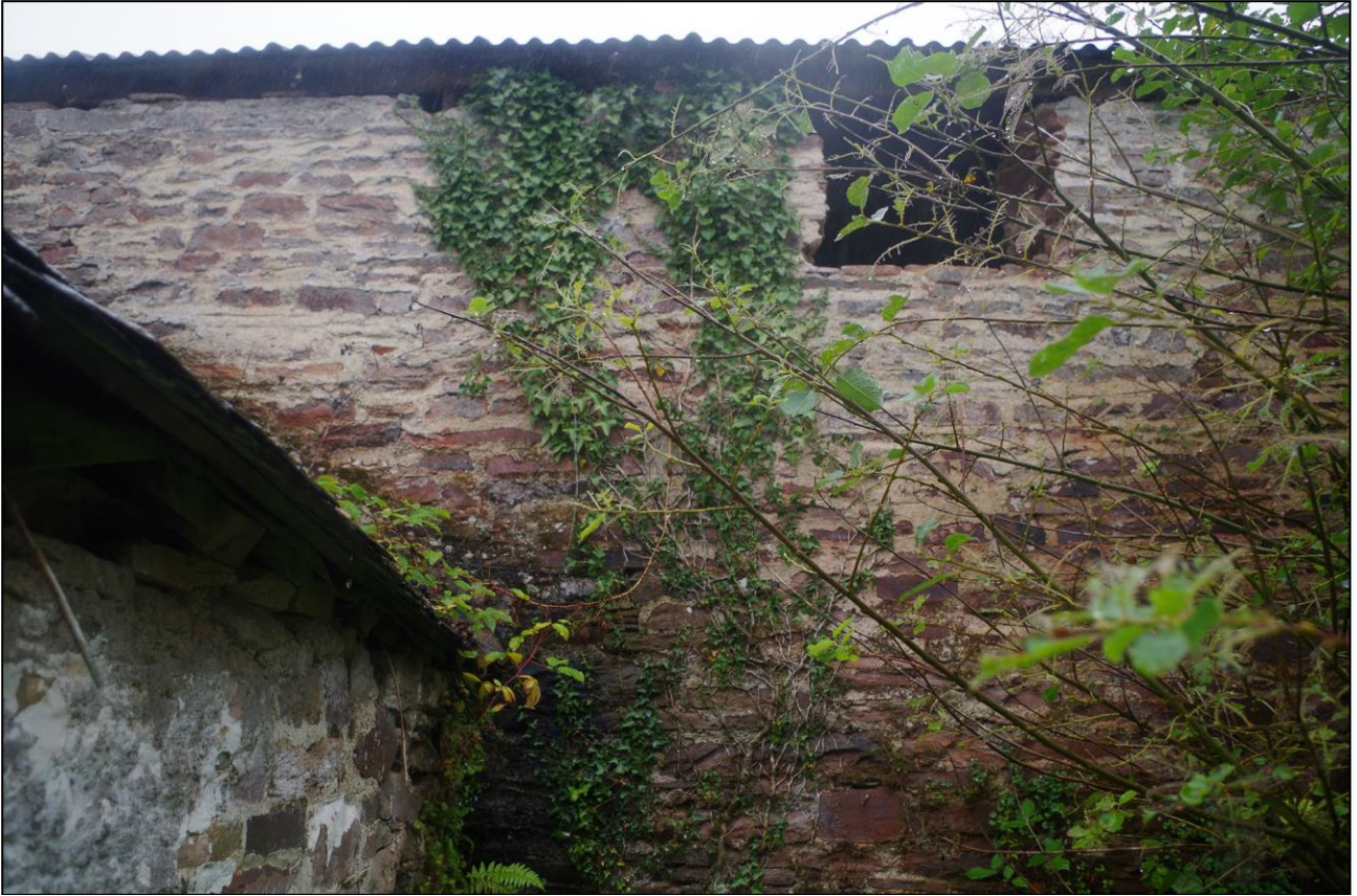
11. OPENING AT EAVES IN NORTHERN EDGE OF B1 AND NORTH ELEVATION OF B2; VIEWED FROM THE E.
