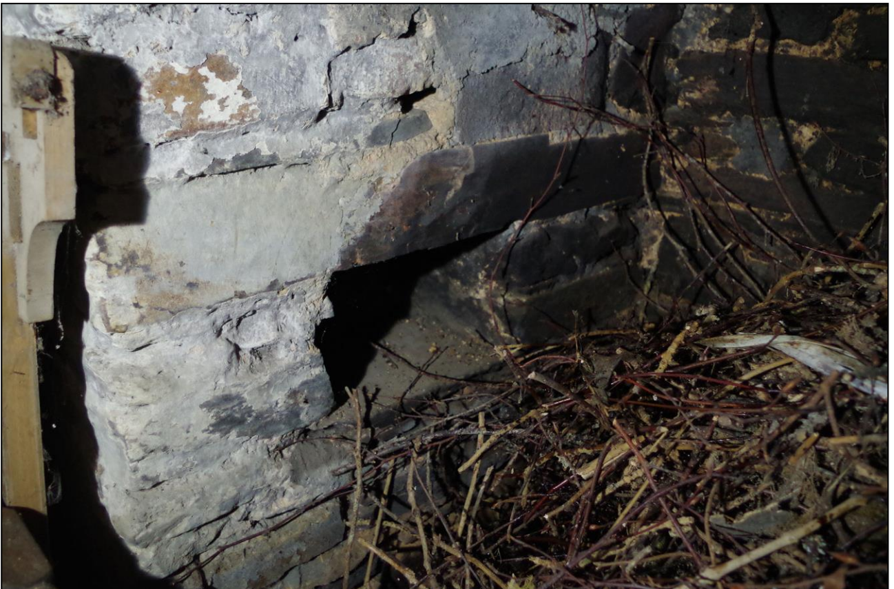
28. THE SMOKING BOX TO THE LEFT OF THE FIREPLACE; VIEWED FROM THE NW.
