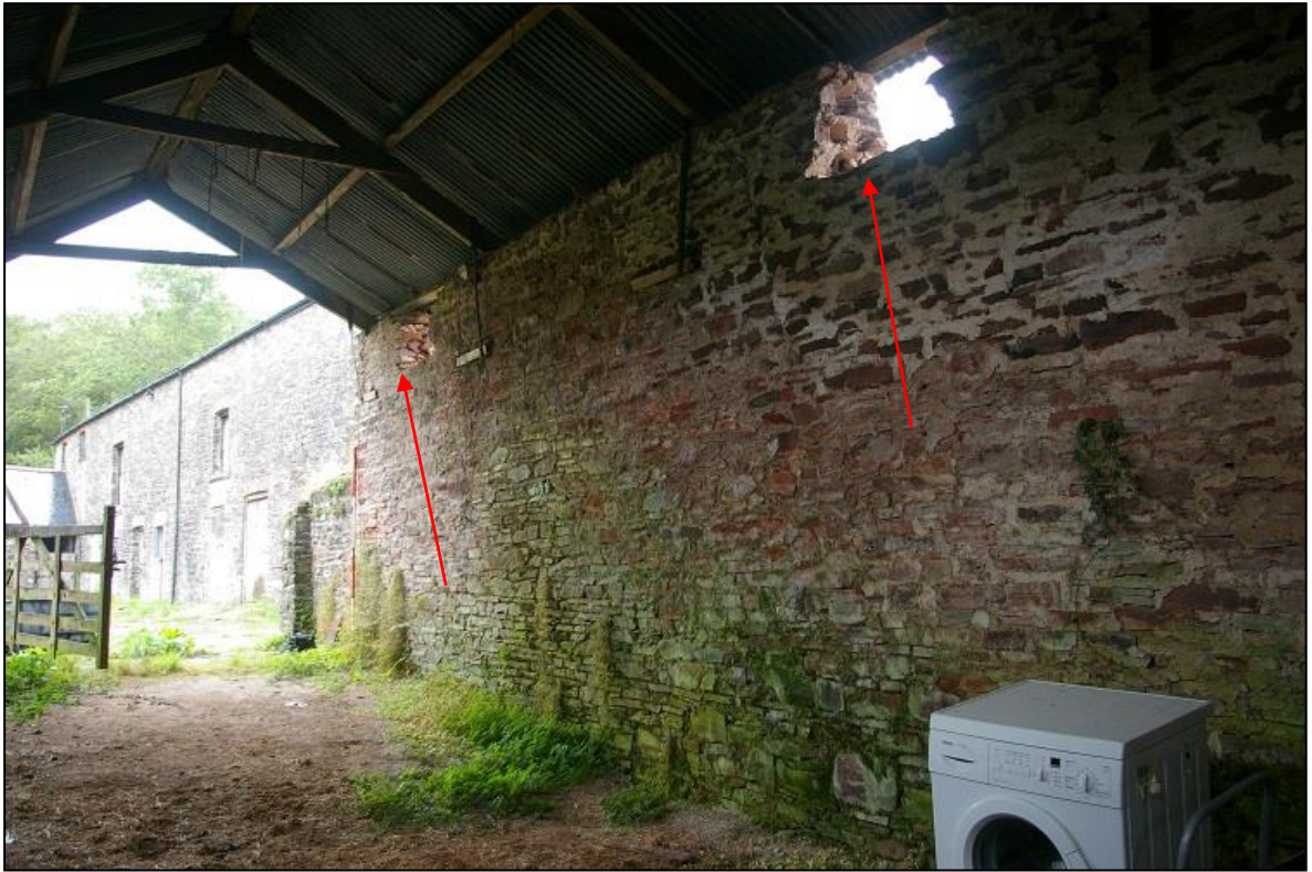
FIGURE 26: OPENINGS KNOCKED INTO THE EAVES OF B1 TO MAKE WINDOWS; FROM THE SOUTH-WEST, 2M SCALE.
