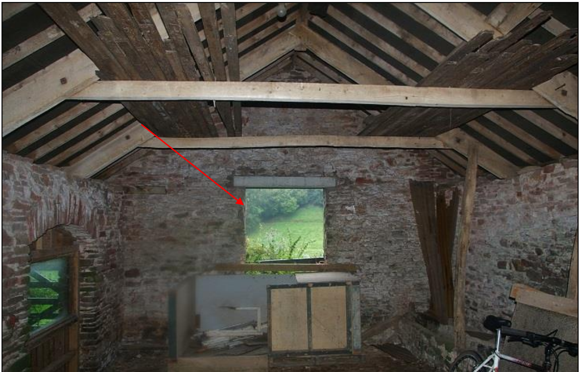
FIGURE 27: B7, THE WEST GABLE END - RECENTLY FORCED WINDOW WITH CONCRETE LINTEL; FROM THE EAST.
