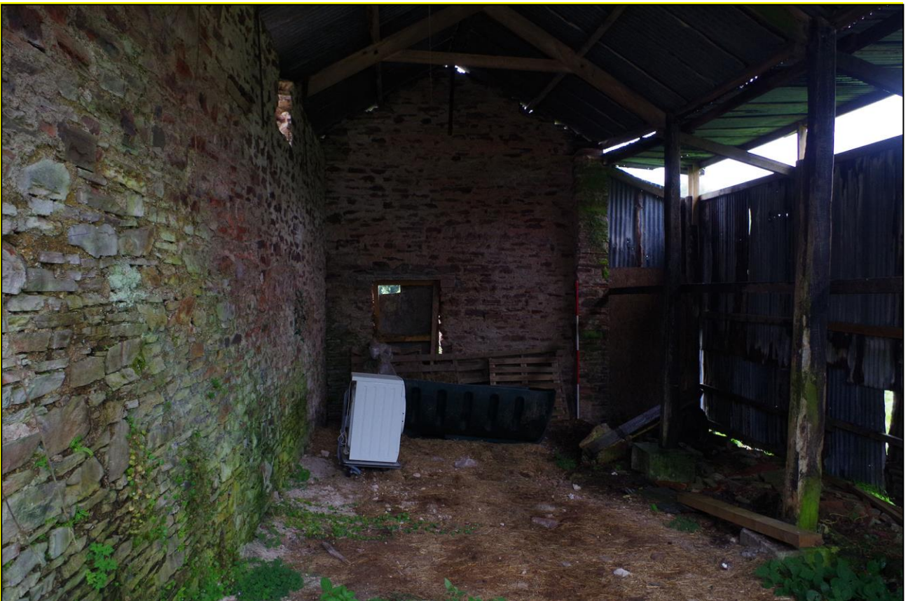
4. INTERNAL VIEW OF B1 SHOWING FORCED DOORWAY ON SOUTH WALL AND WEST CANOPY; VIEWED FROM THE N.
