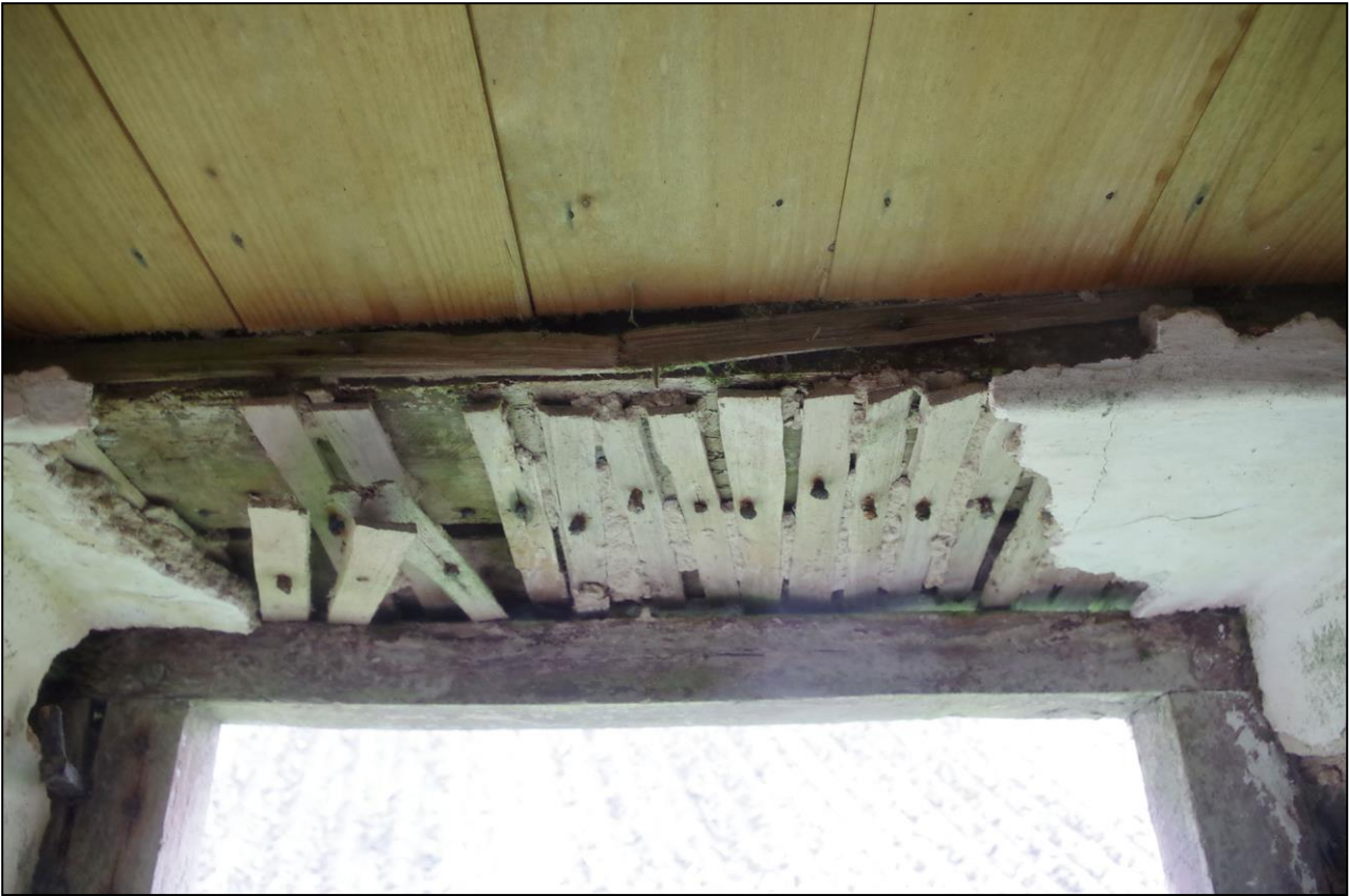
15. LATHE AND PLASTER STILL SURVIVING IN THE CEILING OF ENTRANCE IN PRIVY; VIEWED FROM THE W.
