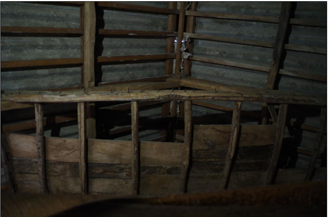
30. THE STICK SLEEPING LOFT, COMPLETE WITH FLOORBOARD SAND HANGING PINS; VIEWED FROM BELOW.
