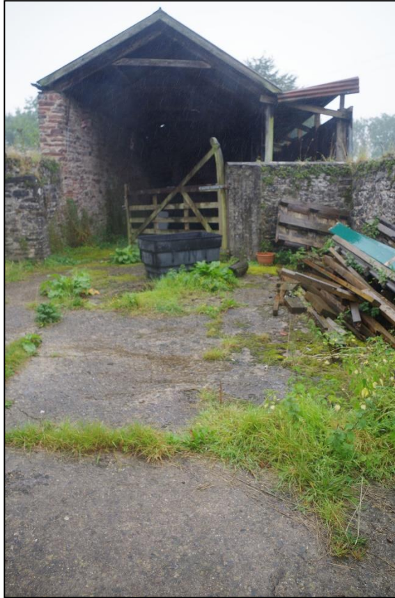
9. DOUBLE HEIGHT OPENING OF B1; VIEWED FROM THE BANK BARN YARD FROM THE N.
