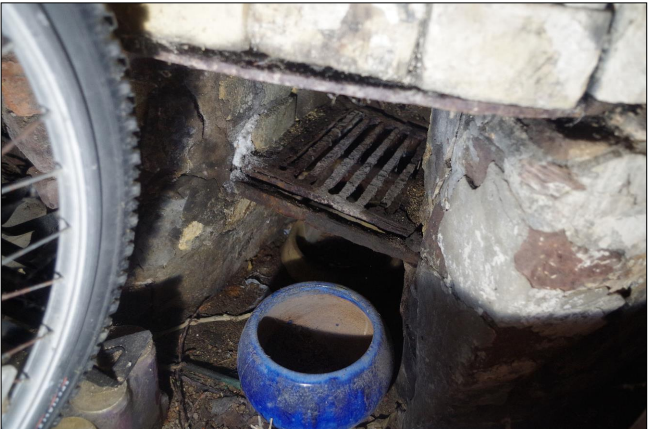
32. THE GRATE STILL SURVIVES TO THE COPPER BASIN STRUCTURE; VIEWED FROM THE NE.
