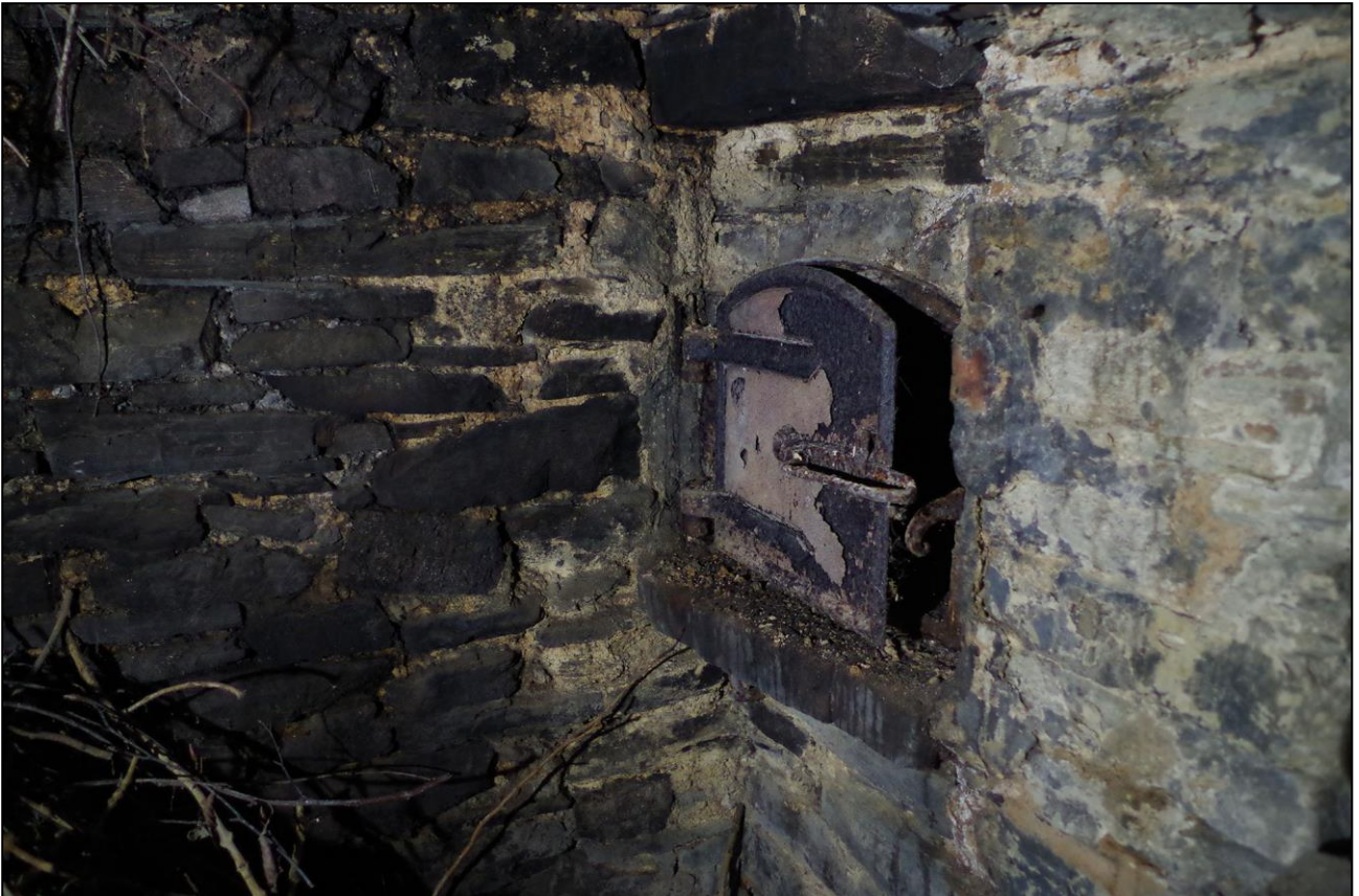
27. THE BREAD OVEN OPENING TO THE RIGHT OF FIREPLACE; VIEWED FROM THE NNE.
