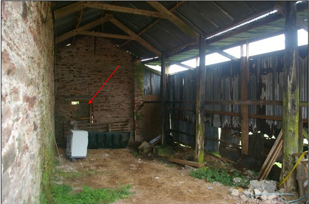
FIGURE 25: B1; DOOR KNOCKED IN SOUTH GABLE, CONCRETE LINTEL, SOFTWOOD FRAMING; FROM THE NORTH-EAST, 2M SCALE.
