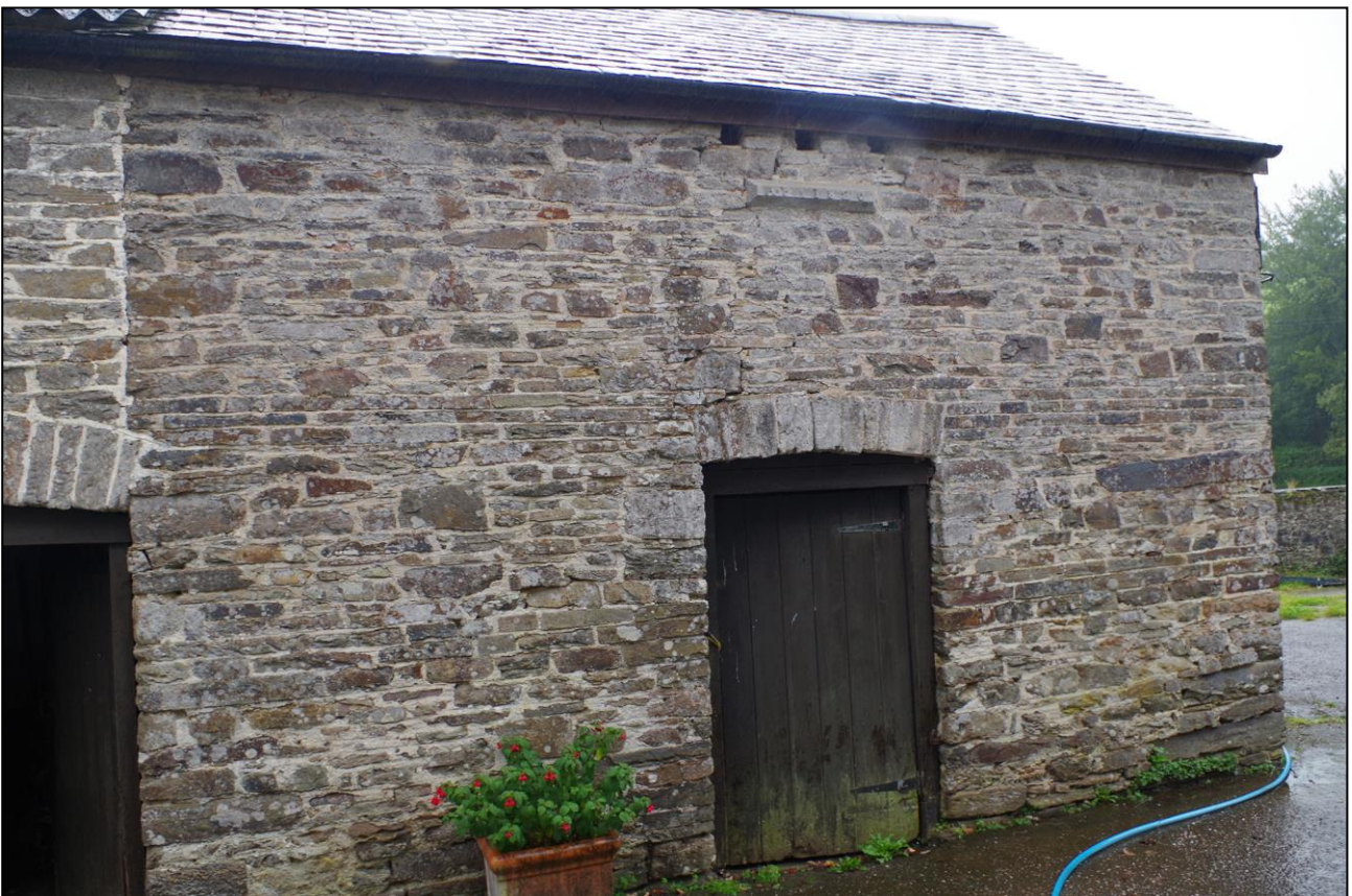
18. B4 WITH CENTRAL DOORWAY, DATE STONE AND DOVE-HOLES ABOVE; VIEWED FROM THE ESE.
