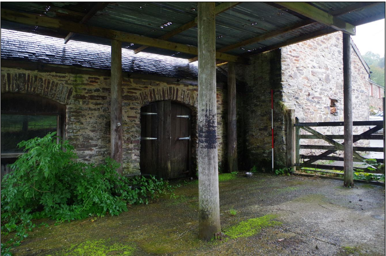
40. THE SOUTH ELEVATION OF B7A, WITH DOUBLE DOOR AND WINDOW; VIEWED FROM THE SW.
