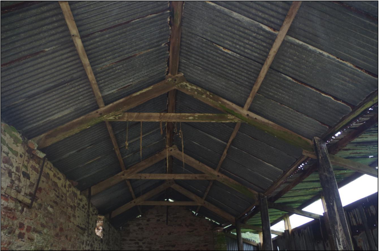
5. ROOF OF B1 AND FORCED OPENING TO THE SOUTH AT THE EAVES; VIEWED FROM THE N.
