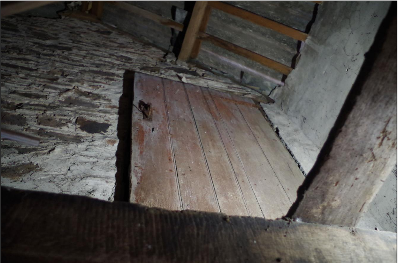
29. THE ORIGINAL PLANKED DOOR WITH BEADED DETAILING IN FORCED DOORWAY ON THE FIRST FLOOR OF B5; VIEWED FROM BELOW.
