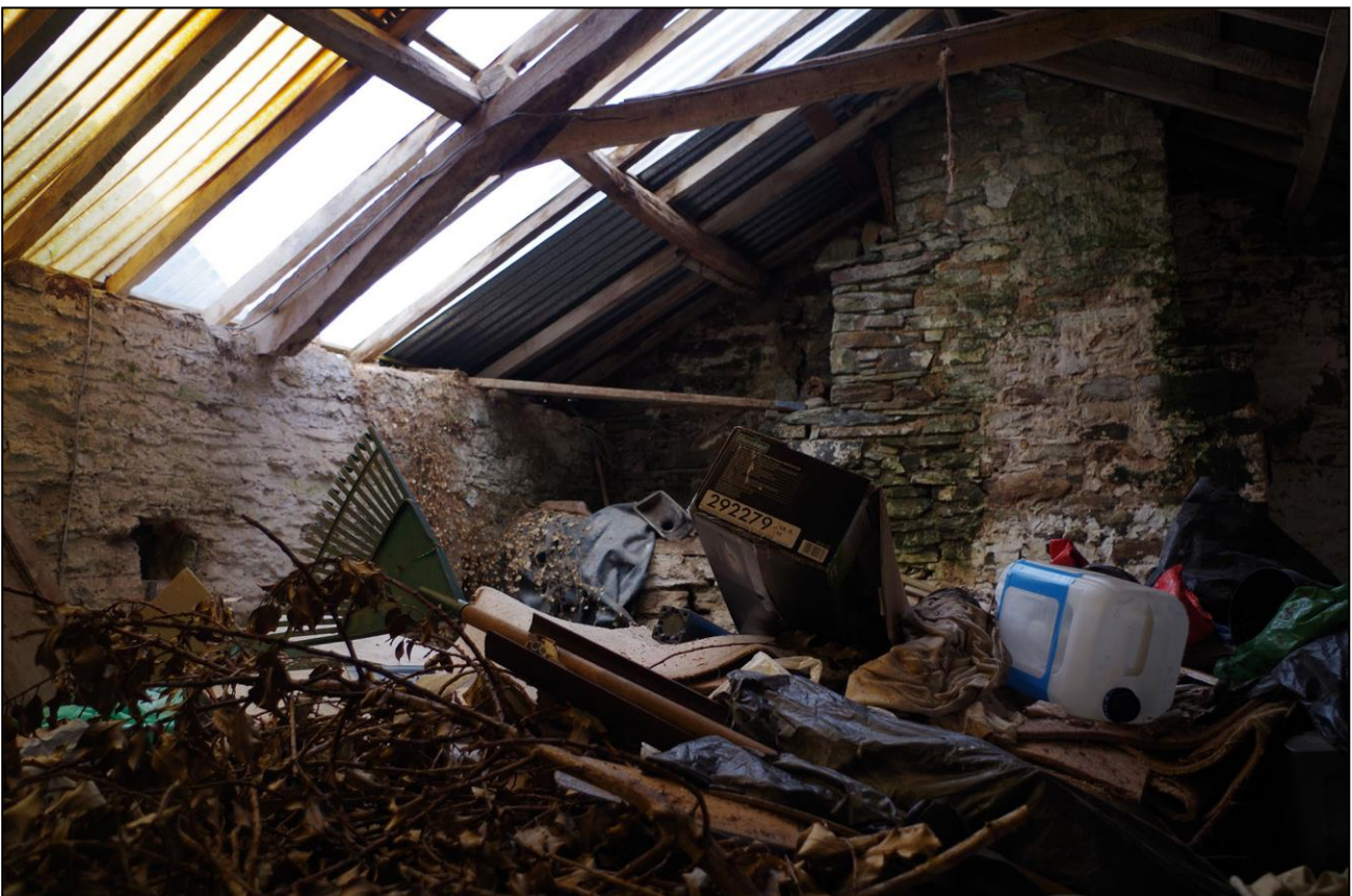
36. INTERNAL VIEW OF B6 NORTH GABLE END, SHOWING STEPPED EXTERIOR OF STEPPED STACK; VIEWED FROM THE S.
