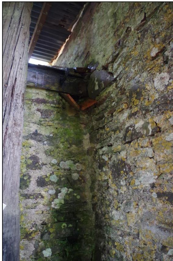
42. THE DRAINAGE ATTEMPT IN THE NE CORNER OF B7A SOUTHERN ELEVATION; VIEWED FROM THE SSW.
