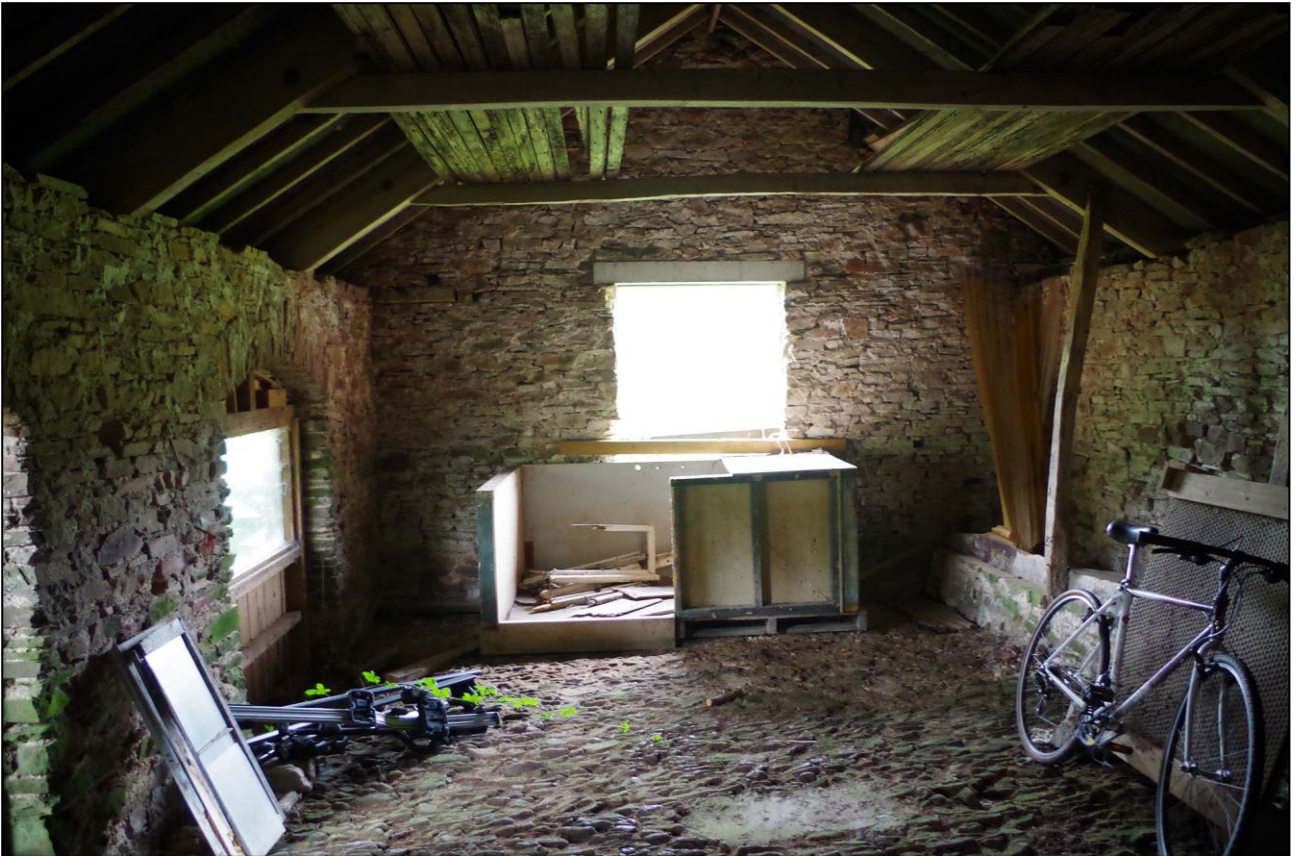
43. THE INTERNAL VIEW OF B7A, LOOKING TO THE WEST. THERE IS A BUILD LINE IN THE SW CORNER SUGGESTING S ELEVATION WAS INFILLED; VIEWED FROM THE E.
