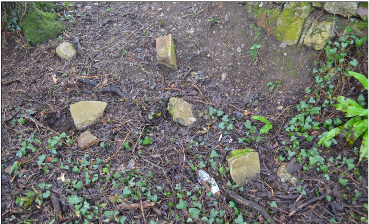
FIGURE 101: BOUNDARY BANK ON NORTHERN EDGE WITH MATERIALS FALLING OUT OF THE BOUNDARY, FROM THE NORTH.
