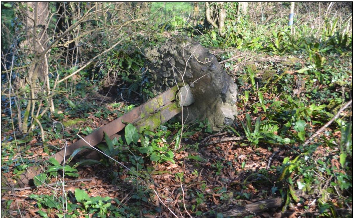
FIGURE 70: DETAIL OF METAL AND CONCRETE POST LOCATED TO THE WEST OF THE BANK FEATURE, FROM THE SOUTH WEST.
