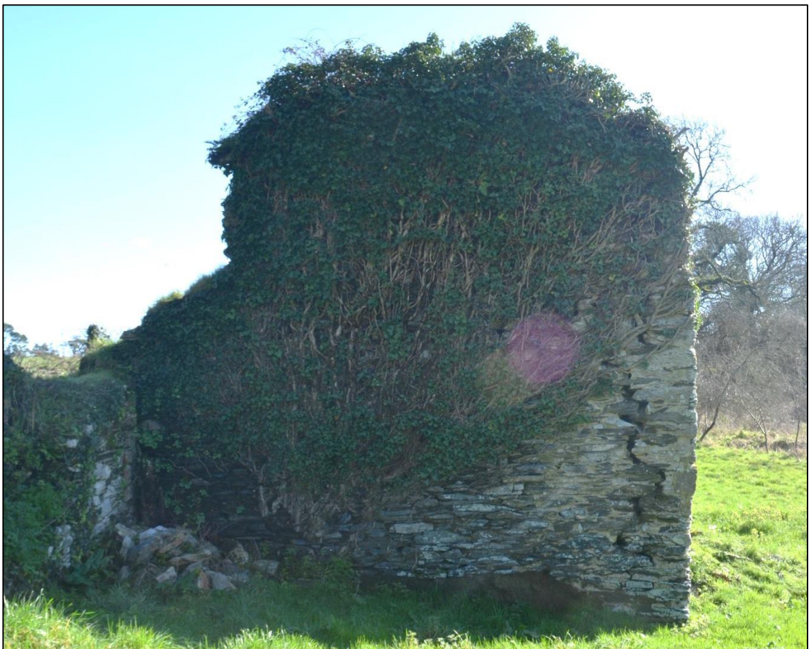
FIGURE 75: BICKHAM BARN SHOWING THE FRONT (SOUTH) ELEVATION PARTING FROM THE WESTERN ELEVATION.
