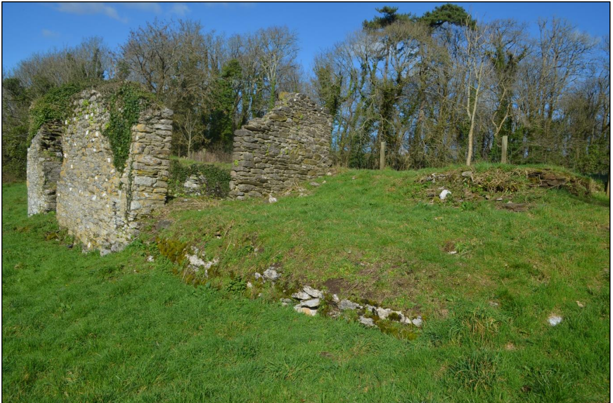
FIGURE 77: THE TRUNCATED EASTERN END OF BICKHAM BARN SHOWING THE CONTINUING STONEMWORK OF THE FORMER EXTENT OF THE STRUCTURE, FROM THE SOUTH-EAST.
