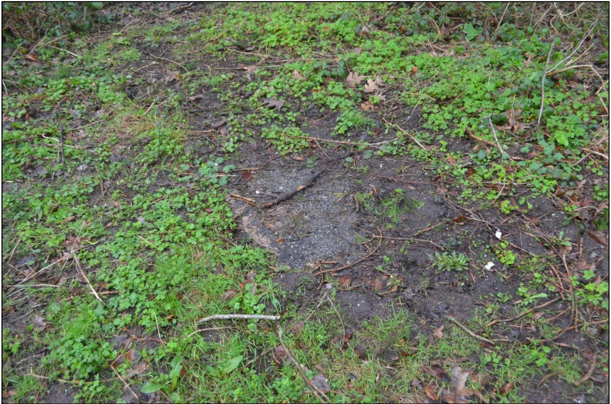
FIGURE 39: TARMAC COVERED CONCRETE ROADWAY NOW ALMOST ENTIRELY COVERED WITH VEGETATION, LEADING OFF SOUTH DRIVE; FROM THE NORTH.
