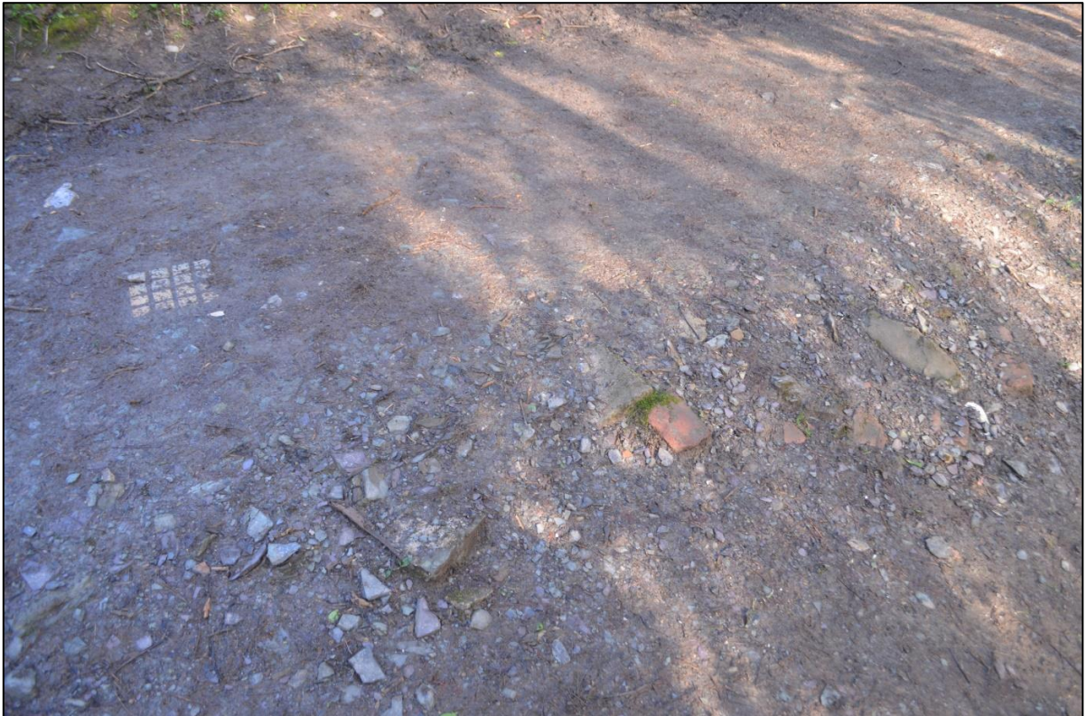
FIGURE 53: RANDOM CAST CONCRETE FLOOR TILE AND BRICKS ERODING FROM PATH EDGING.
