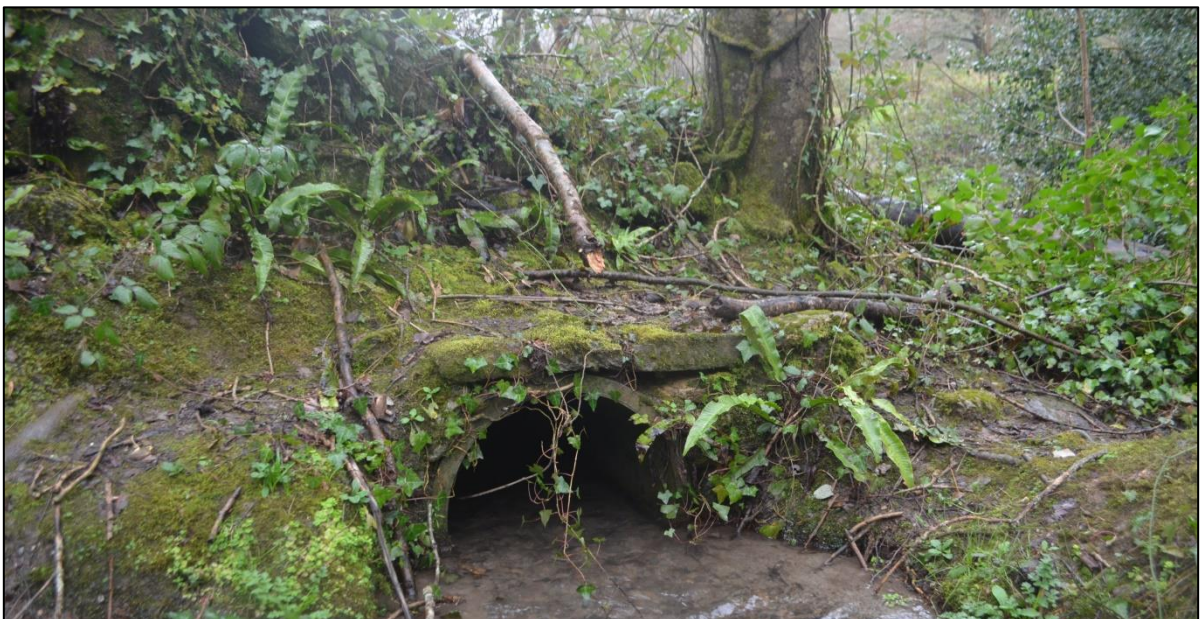
FIGURE 91: STONE FACED BOUNDARY BANK WITH HALF PIPE INSERTED TO ALLOW STREAM TO PASS UNDER. FROM THE WEST.
