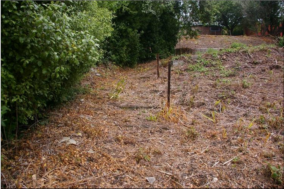
FIGURE 11: SLUMPED STONE HEDGE BANK AND FORMER CONCRETE STEPS AND PATH TO THE WEST OF THE SITE; FROM THE SOUTH.
