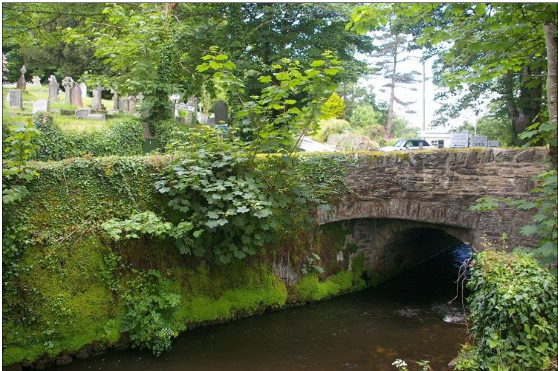
6. The historic bridge which links the two halves of the village: from the east-northeast.
