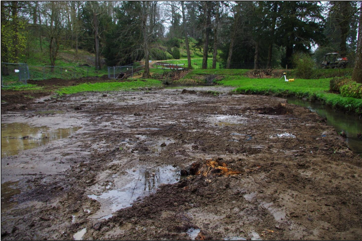
FIGURE 3. PRIOR TO DE-SILTING THE SILT TRAP, WITH TOPSOIL REMOVED. VIEWED FACING NORTH-EAST.
