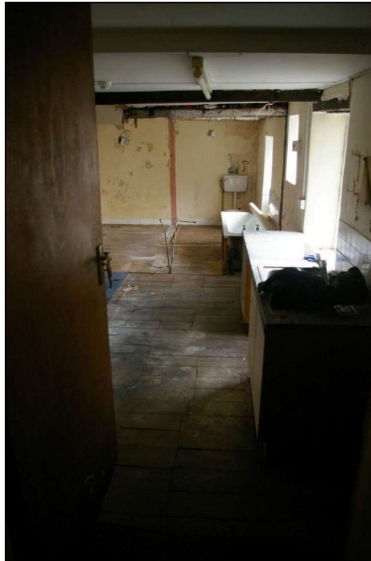
40. D29, LOOKING INTO THE FIRST FLOOR OF BUILDING 2, ROOM 20; FROM THE SOUTH.
