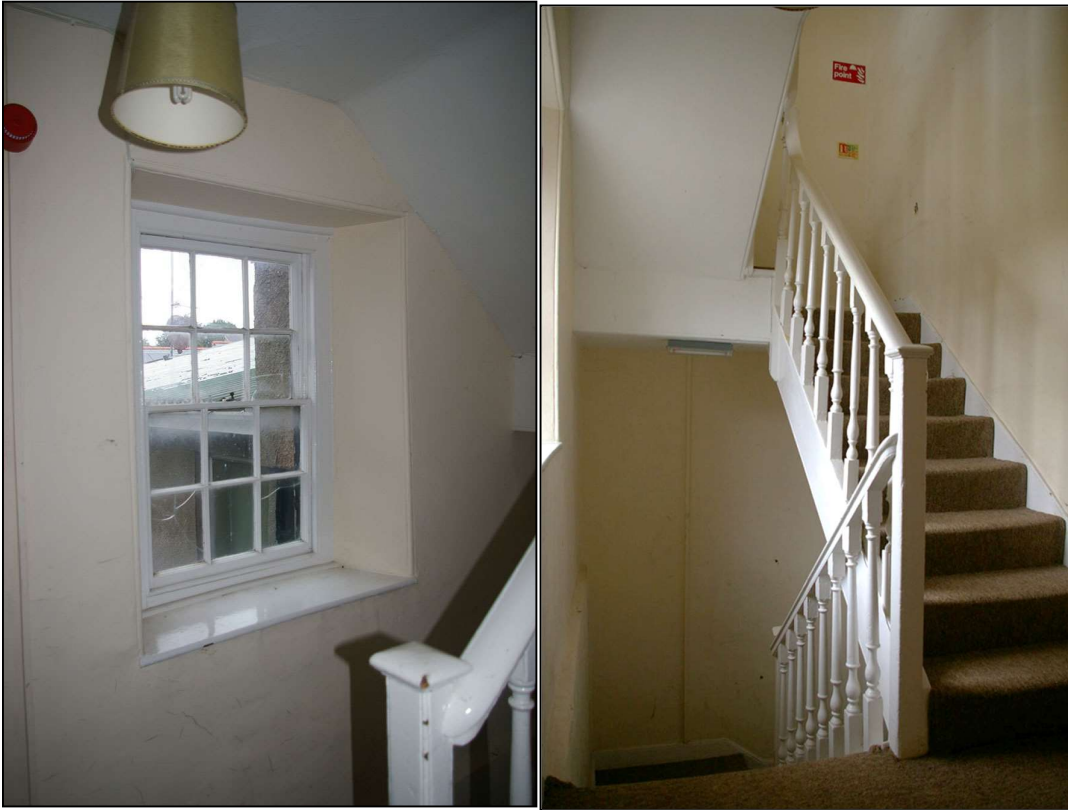
20. LEFT: THE SASH WINDOW IN R6, THE FIRST FLOOR LANDING, A HORNLESS SASH, IN A CHUNKY MOULDED SASH BOX; FROM THE SOUTH-WEST.
