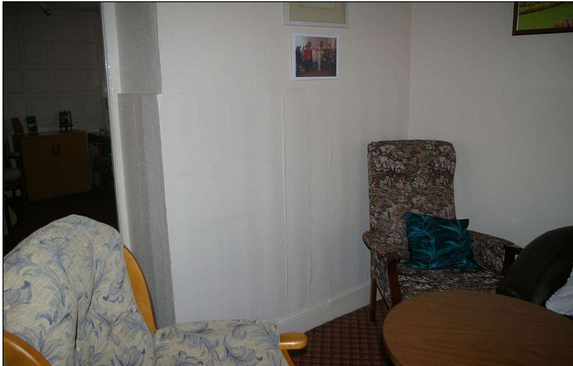
17. THE SURVIVING BEADED PLANK PANELLING IN THE NORTH-EAST CORNER OF R2, RUNNING INTO THE FORCED DOORWAY OPENING, PAPERED OVER WITH WOODCHIP WALLPAPER; FROM THE SOUTH-WEST.
