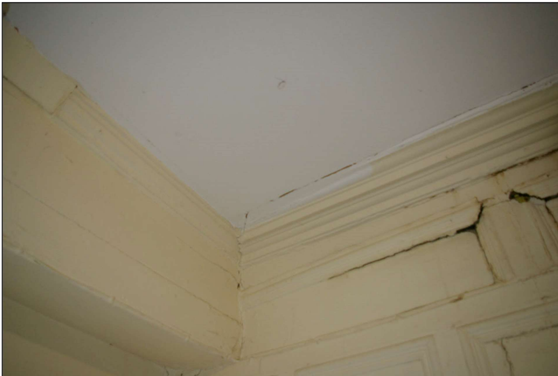
76. THE DIFFERENT WOODEN CORNICES MEETING IN THE SOUTH-EAST CORNER OF THE ROOM; FROM THE NORTH-WEST.
