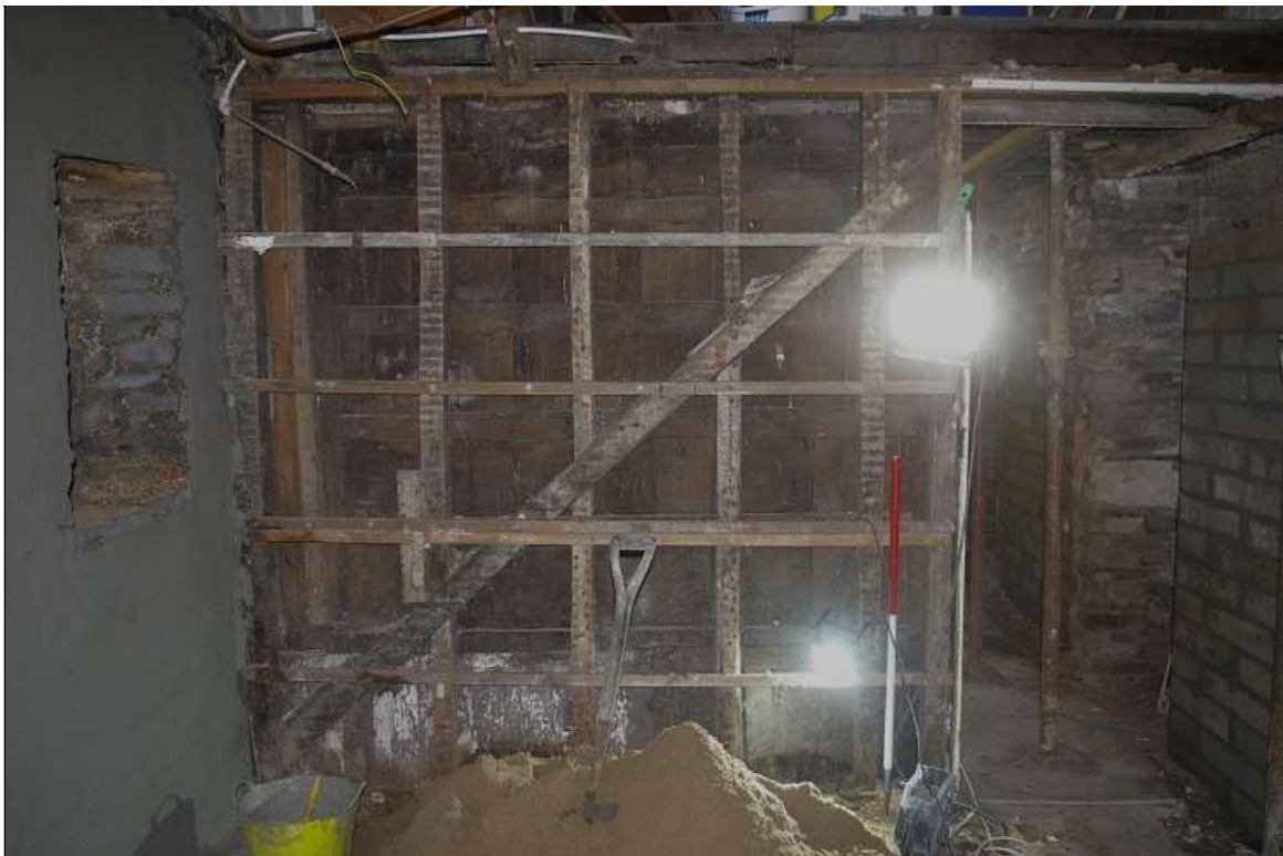
94. VIEW OF PARTITION WALL R18, WITH GOOD SLATE BUILT REVEALS TO FORMER SLIT VENT TO LEFT HAND SIDE, FROM THE NORTH (1M SCALE)
