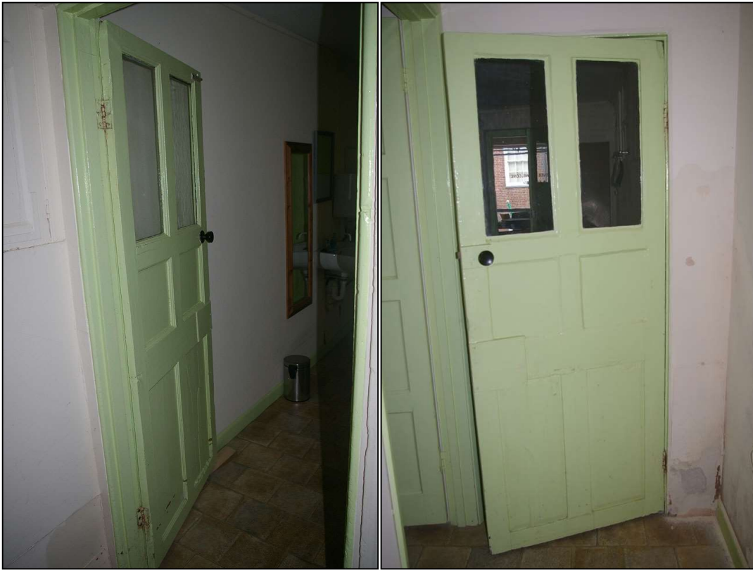
34. LEFT & RIGHT: D25, BETWEEN R17 AND R19, 18TH CENTURY STYLE DOOR WITH TWO GLASS PANES INSERTED; FROM THE SOUTH-EAST AND NORTH.
