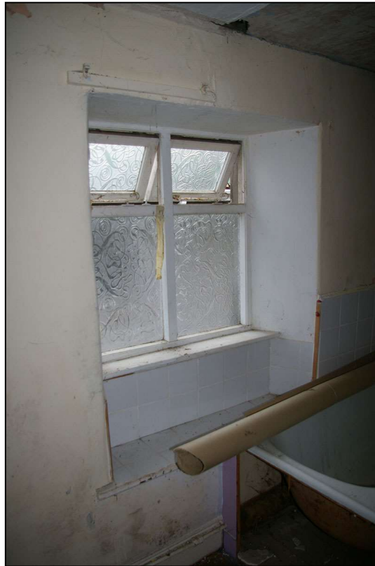
46. W19, SHOWING THE LOWERED WINDOW SEAT BEHIND THE BATH; FROM THE NORTH-WEST.
