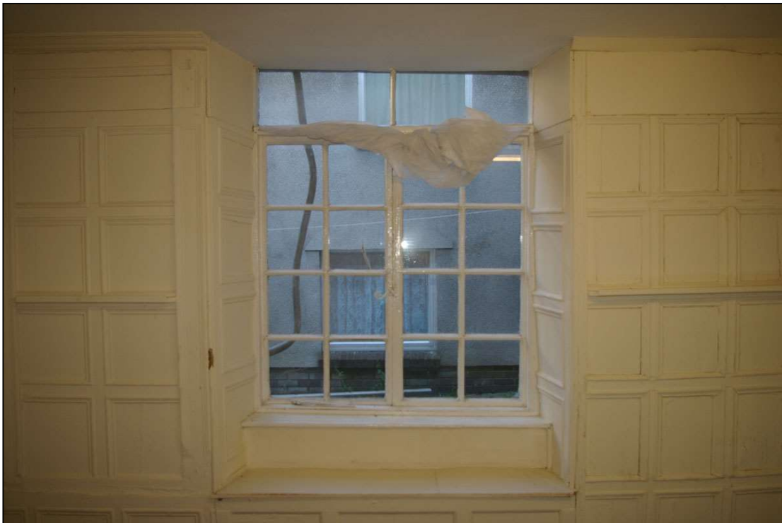
FIGURE 9: W13 IN ROOM 17, WITH RECYCLED AND RESET 18 TH CENTURY PANELLED SECTIONS TO THE SIDES. THE SHUTTERS, CUT AND NAILED SHUT, AND EARLY 19 TH CENTURY PANNELLING FORMING A WINDOW SEAT; FROM THE WEST.
