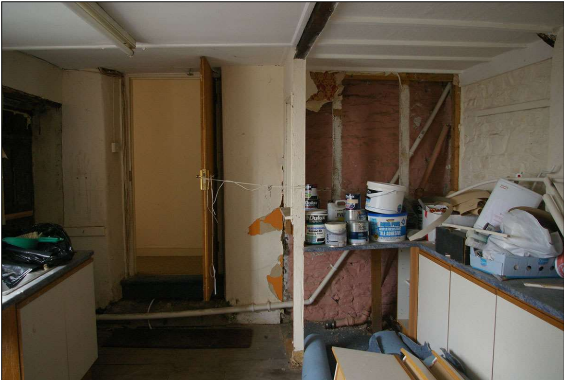
43. THE SOUTH PARTY WALL BETWEEN BUILDING 1 AND BUILDING 2, WITH FORCED DOOR, D29; FROM THE NORTH.
