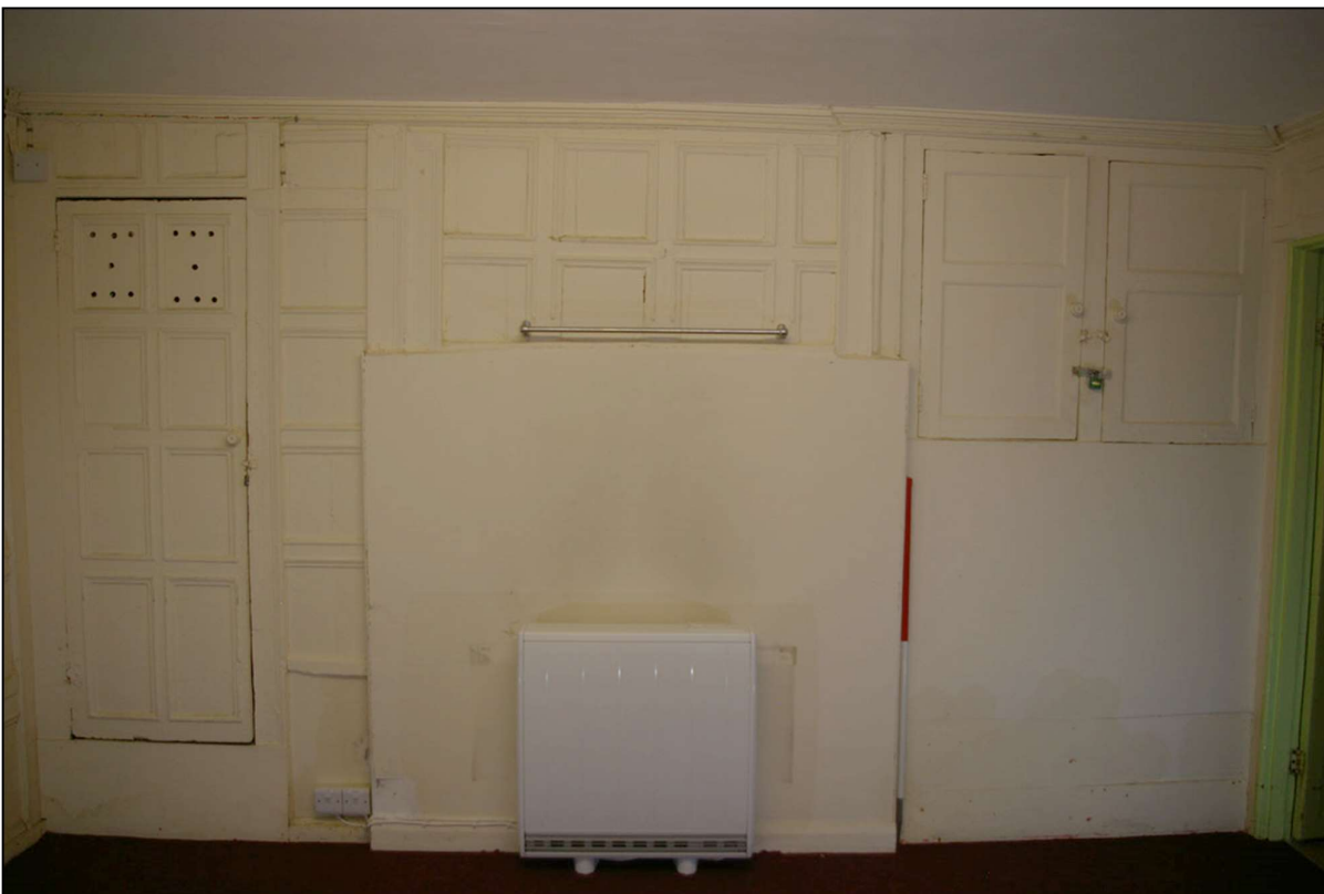
58. THE WEST WALL, WITH 1M SCALE, WITH CUPBOARD, BLOCKED FIREPLACE AND CUPBOARD TO NORTH; FROM THE EAST.
