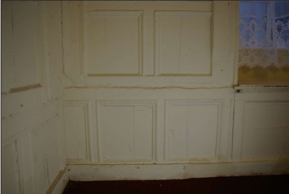
69. THE RAGGED JOINTS BETWEEN THE SECTIONS OF PANELLING ON THE EAST WALL; FROM THE WEST
