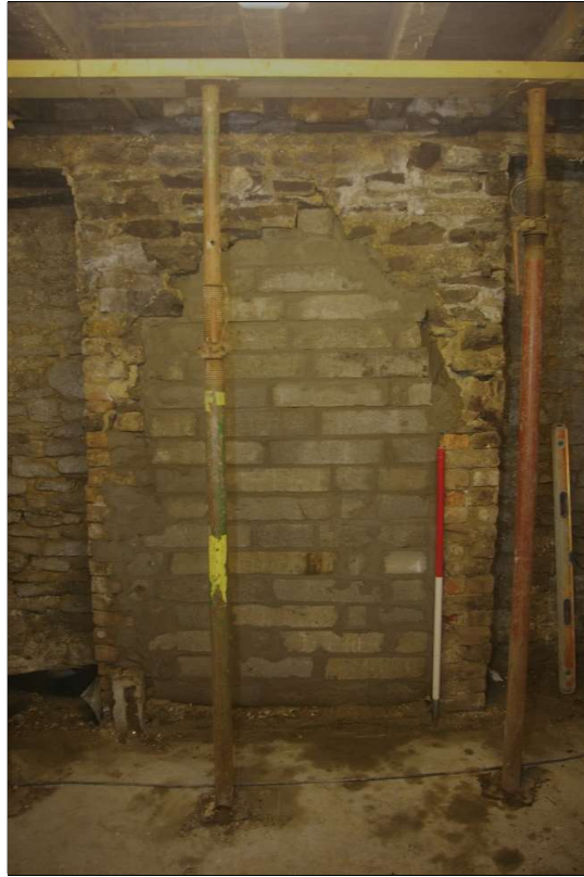
97. ALTERED STACK, SERVING NO.25, WITH FORCED AND NOW BLOCKED HEARTH SERVING NO.23; FROM THE EAST (1M SCALE).
