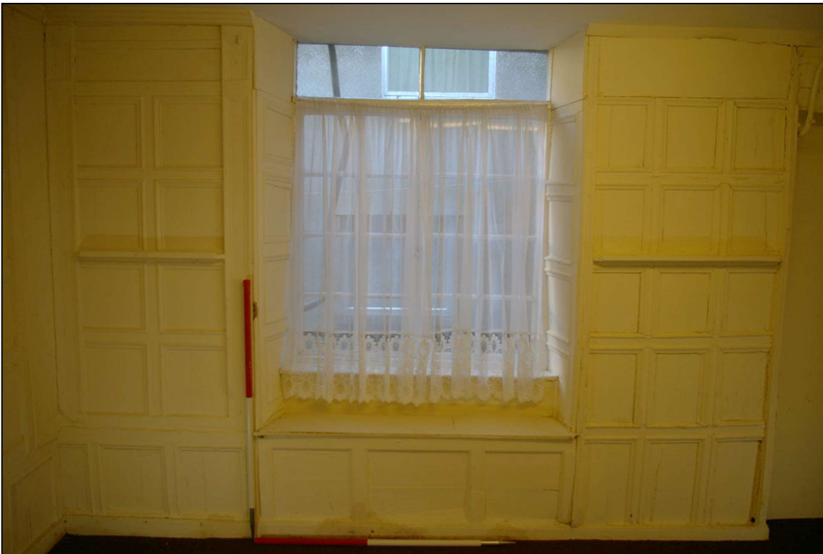
54. THE EAST WALL AND W13 WITH 2 X 1M SCALES; FROM THE WEST.
