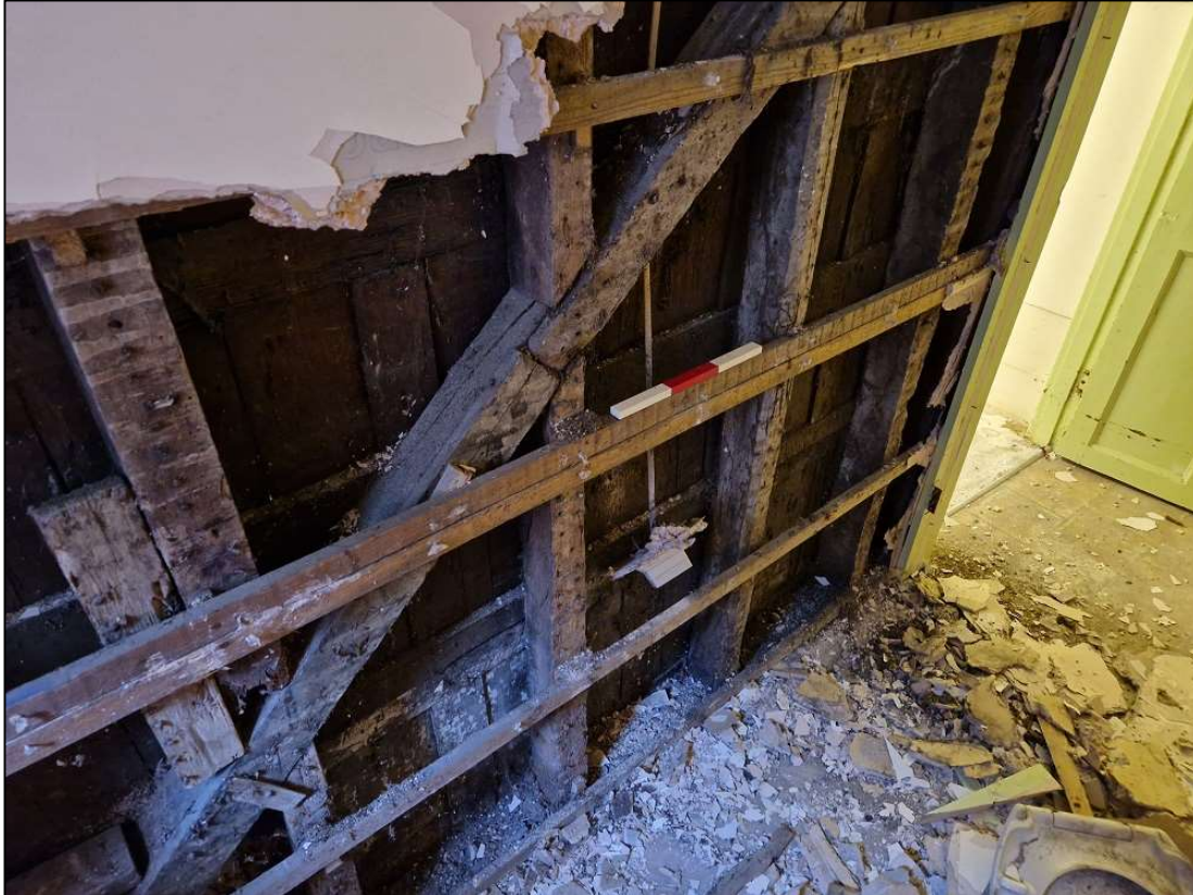
FIGURE 23: THE TIMBER-FRAMED PARTITION BETWEEN R17 AND R18; FROM THE NORTH-EAST (0.3M SCALE).
