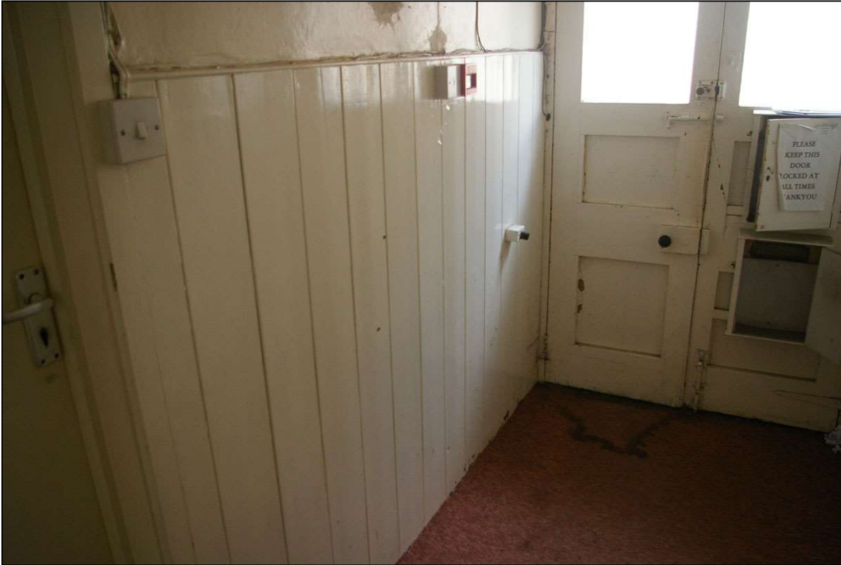
10. THE PLAIN BEADED PLANK PANELLING, 1803, TO THE EAST OF THE CORRIDOR; FROM THE NORTH-WEST.
