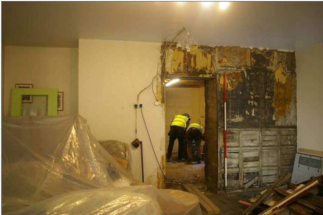
98. THE NORTH WALL OF R2, SHOWING PARTIALLY STRIPPED WALL COVERINGS, EXPOSING INTERESTING DECORATIVE SCHEMES AND RESET TIMBERWORK AND PANELLING; FROM THE SOUTH-WEST (2M SCALE).
