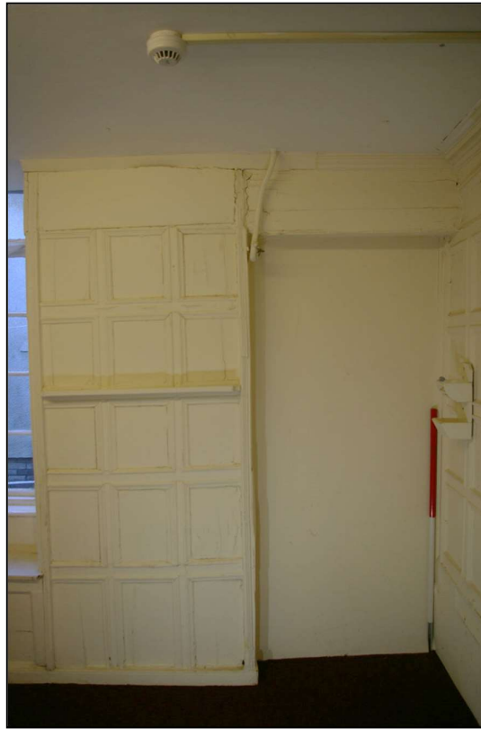
75. THE EAST WALL AT THE SOUTH END, WITH D7 AND 1M SCALE; FROM THE WEST.
