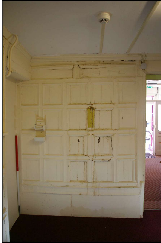
77. THE SOUTH WALL, EAST END, WITH 1M SCALE, D7 AND D24, SHOWING THE WATER DAMAGE TO THIS WALL; FROM THE NORTH.
