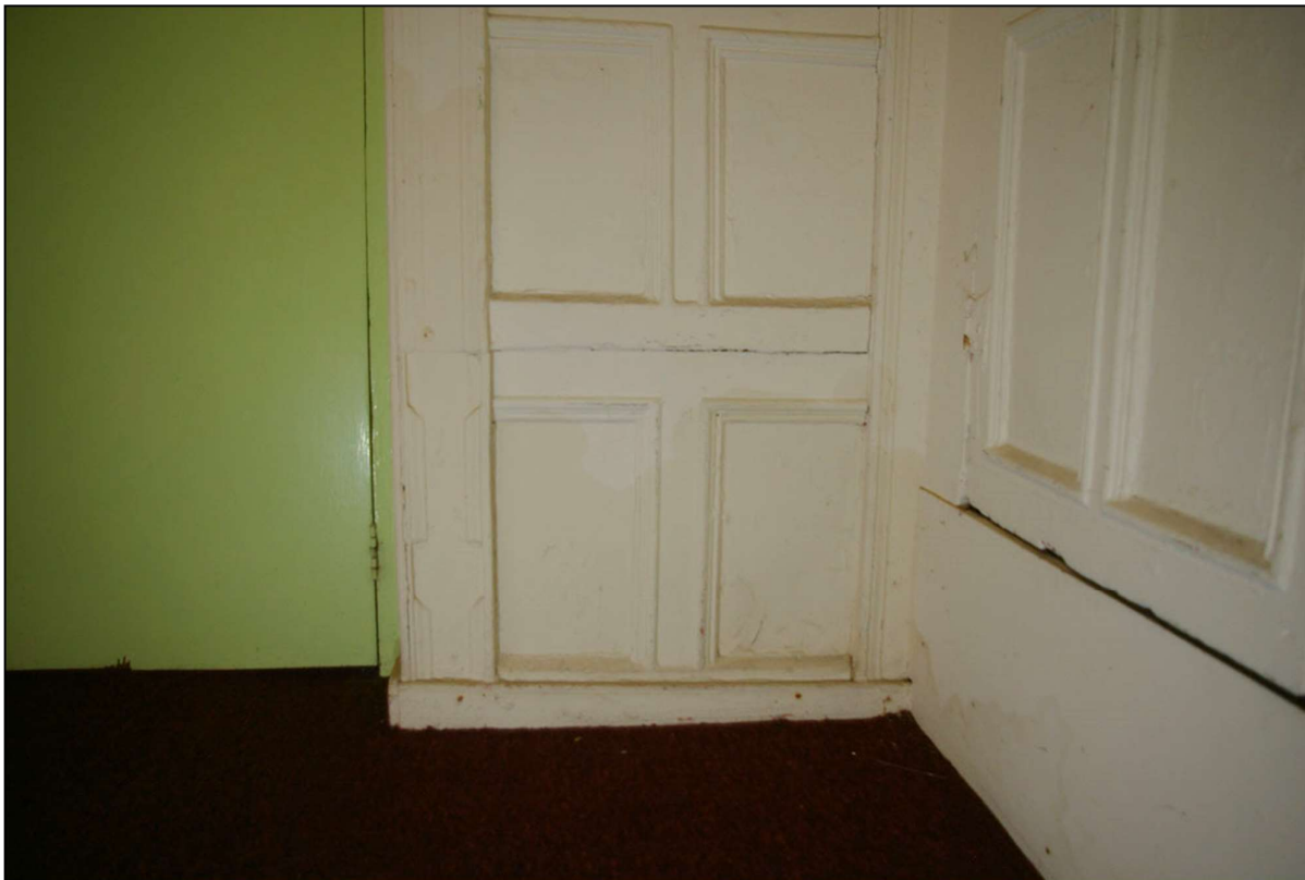
84. THE CUT AND RESET PANELLING IN THE SOUTH-WEST CORNER; FROM THE NORTH.
