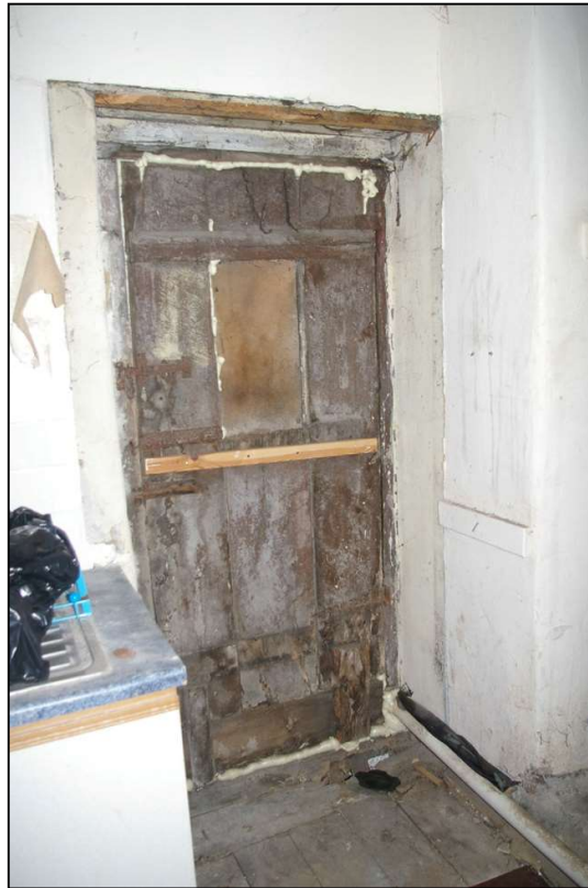
44. GOOD LATER 18 TH OR EARLY 19 TH CENTURY DOOR, D30, NAILED SHUT IN BOARDED OVER OPENING IN THE EAST WALL OF ROOM 20; FROM THE WEST-NORTH-WEST (WITH FLASH).
