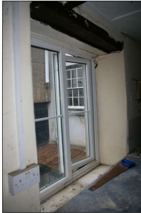
48. W17, SHOWING MODERN DOUBLE GLAZING IN DEEP OPENING, WITH WINDOW SEAT BELOW AND CHUNKY TIMBER LINTEL; FROM THE NORTH-WEST
