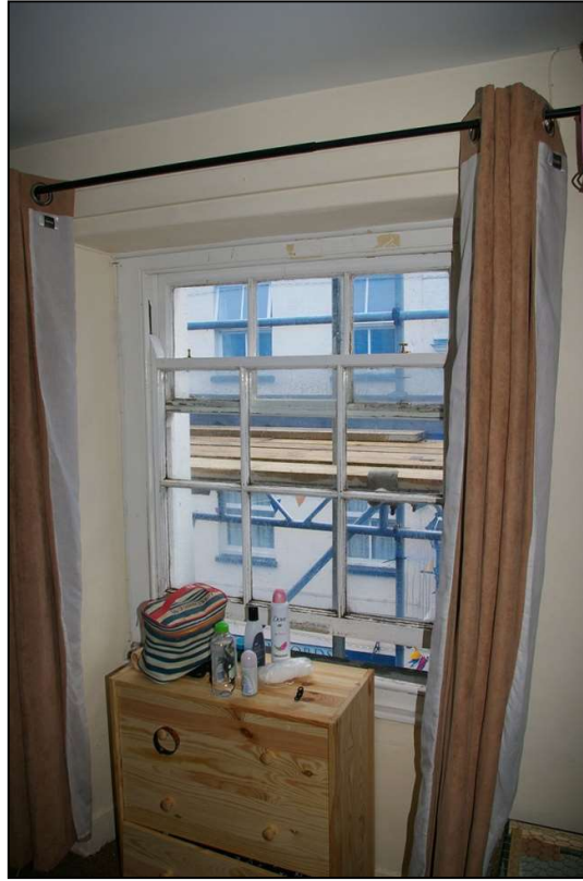
26. RIGHT: THE LATER HORNED SASH WINDOW WHICH LIGHTS R13; FROM THE NORTH-WEST.
