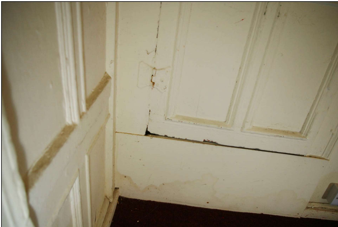
87. THE BUTTERFLY HINGES TO THE CUPBOARD IN THE SOUTH-WEST CORNER OF ROOM 17; FROM THE EAST.
