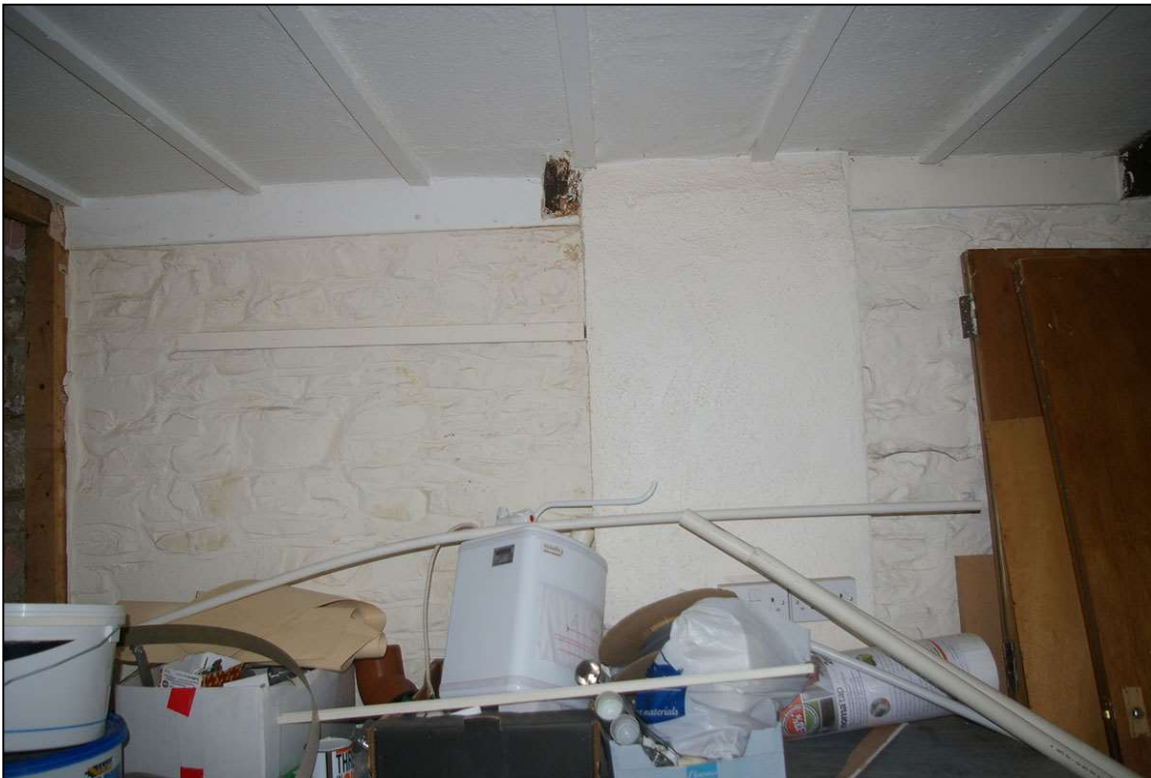
49. THE NARROW BRICK RENDERED STACK BUILT ONTO THE EARLIER HEAVY STONE RUBBLE WEST WALL OF ROOM 20; FROM THE EAST.
