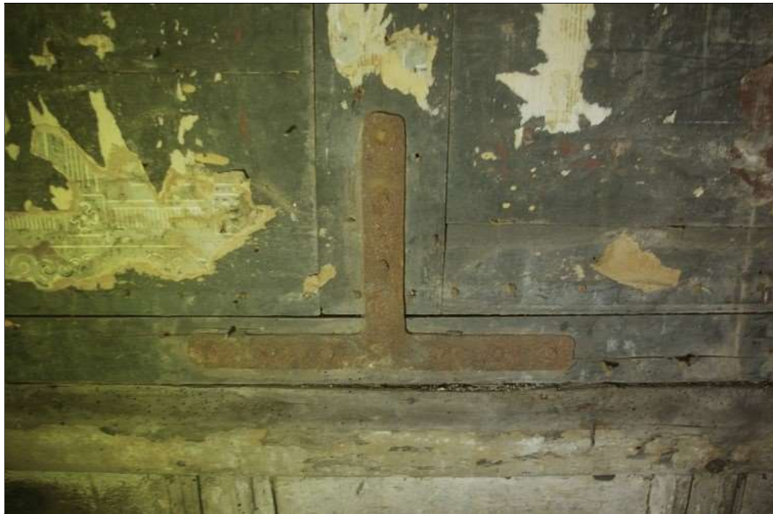
102. DETAIL OF ONE OF THE T-BRACE STRAPS ON THE RESET SHUTTER IN R2.
