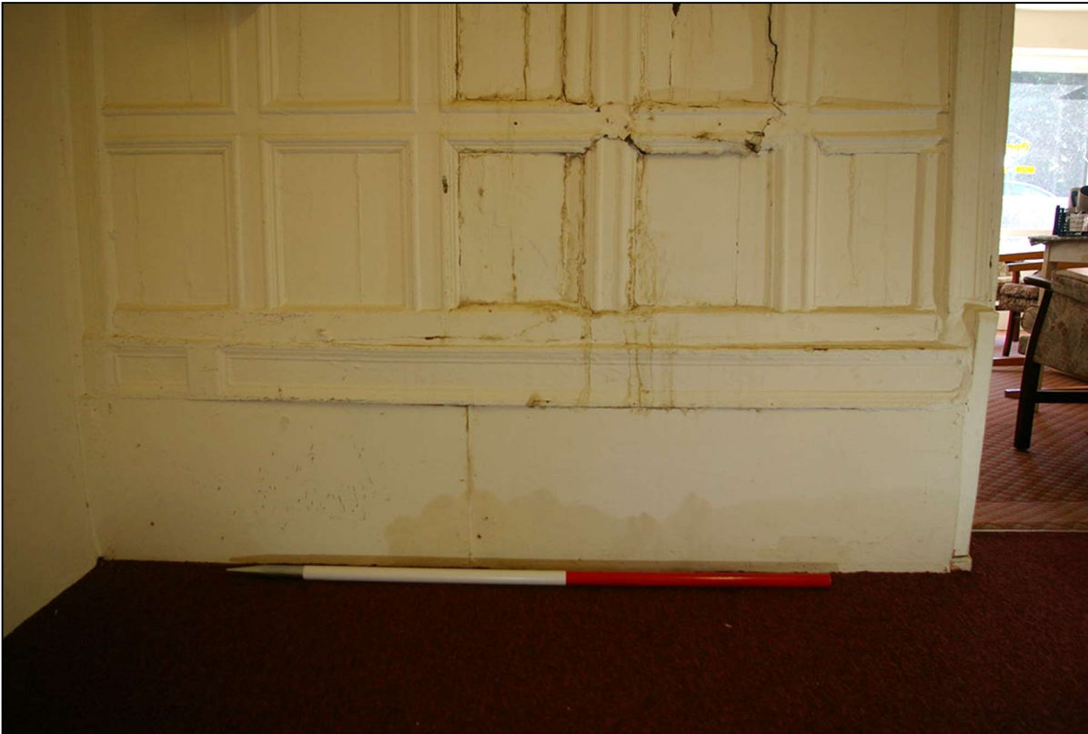
80. THE BASE OF THE SOUTH WALL, WITH 1M SCALE; FROM THE NORTH.
