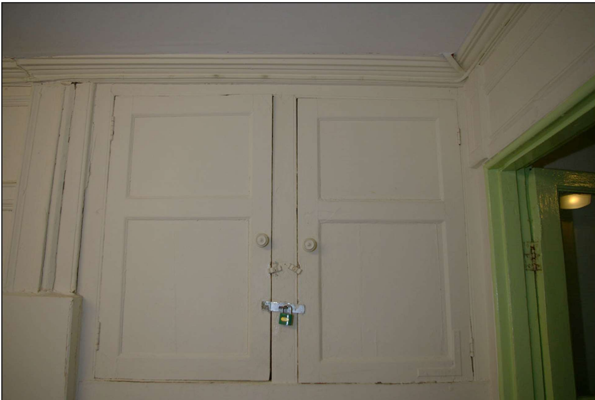
33. THE 18 TH OR EARLY 19 TH CENTURY BEADED, FLAT PANELLED CUPBOARD DOORS TO THE NORTH OF THE STACK IN R17; FROM THE EAST.
