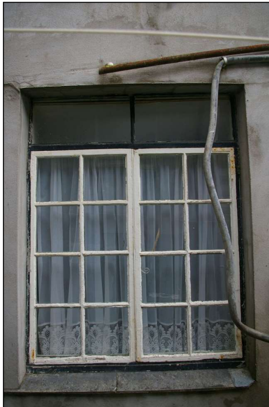
29. W13, 19 TH CENTURY CASEMENT WITH GLASS FILLET ABOVE, INFILLING AN ORIGINALLY TALLER OPENING; FROM THE EAST.
