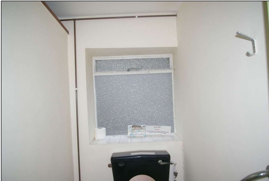
37. W15, ONE OF THE METAL FRAMED CRITTAL-STYLE WINDOWS IN ROOM 19; FROM THE WEST.
