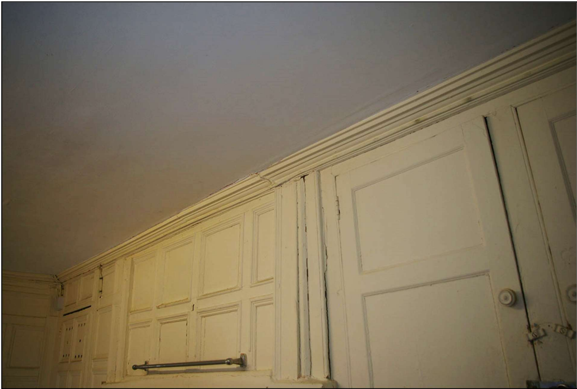
90. THE CUT AND RESET WOODEN CORNICE ALONG THE WEST WALL; FROM THE NORTH, NORTH-EAST
