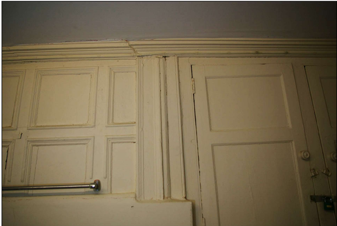
91. THE CUT AND RESET PILASTERS BETWEEN THE PANELLING AND CUPBOARD TO THE NORTH OF THE FIREPLACE; FROM THE EAST.
