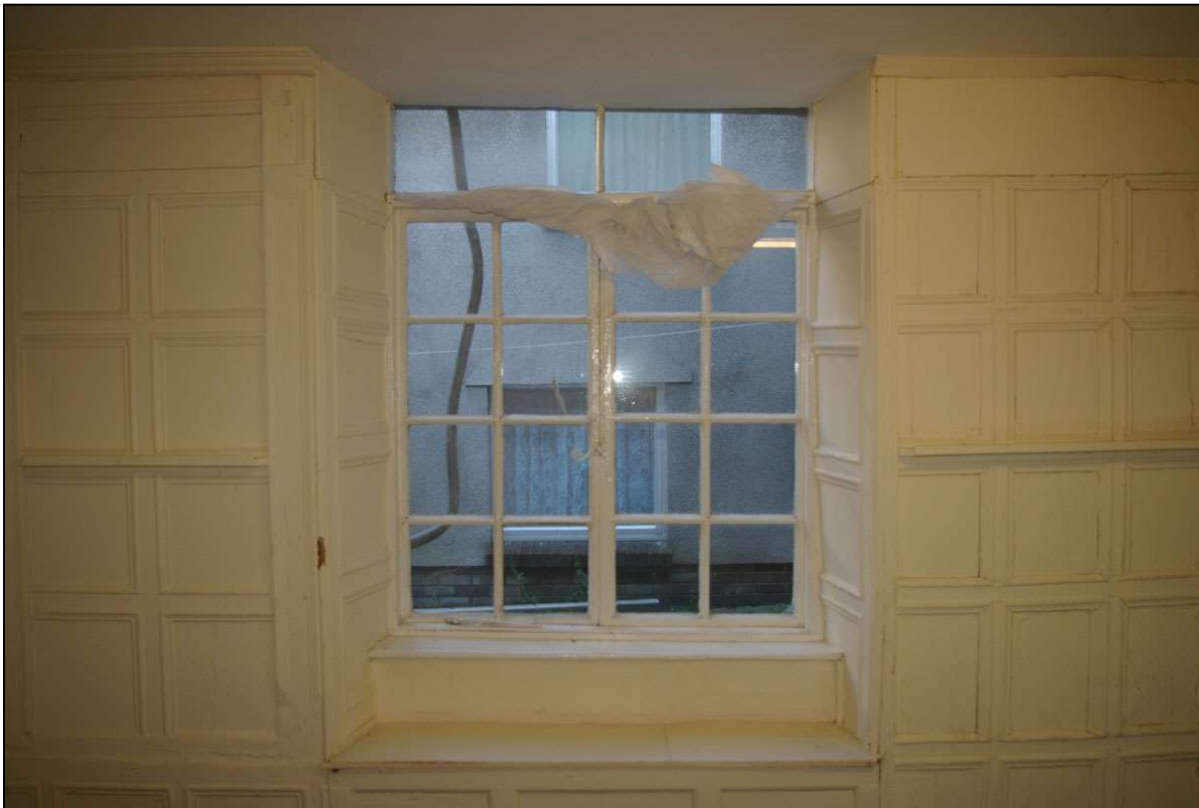
31. W13, WITH RECYCLED AND RESET 18 TH CENTURY PANELLED SECTIONS TO THE SIDES, SHUTTERS, CUT AND NAILED SHUT AND WINDOW SEAT; FROM THE WEST.
