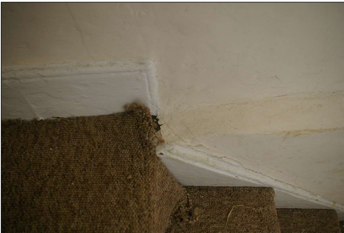
19. THE THICK SECTION OF GROUND FLOOR WALL, SHOWING A LEDGE DESIGNED FOR A FIRST FLOOR, SHOWING THIS STAIRCASE IS INSERTED INTO AN EARLIER SECTION OF BUILDING; FROM THE SOUTH-WEST.
