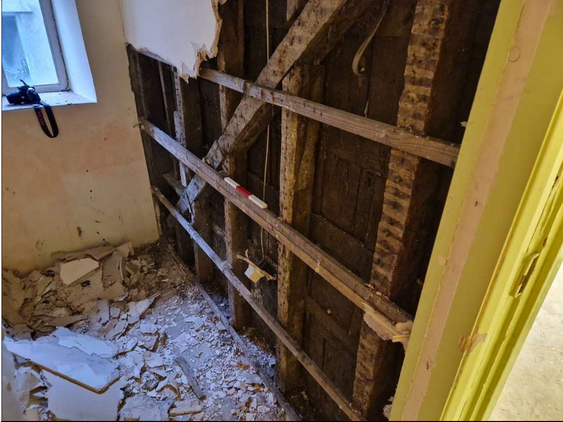
93. THE NORTH SIDE OF THE 19 TH CENTURY PARTITION BETWEEN R17 AND R18; FROM THE NORTH-WEST (0.3M SCALE).
