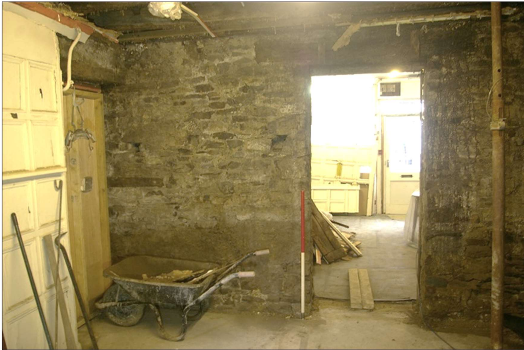
FIGURE 20: THE REAR WALL OF THE FRONT BLOCK, WITH PANELLING REMOVED; FROM THE NORTH (1M SCALE).
