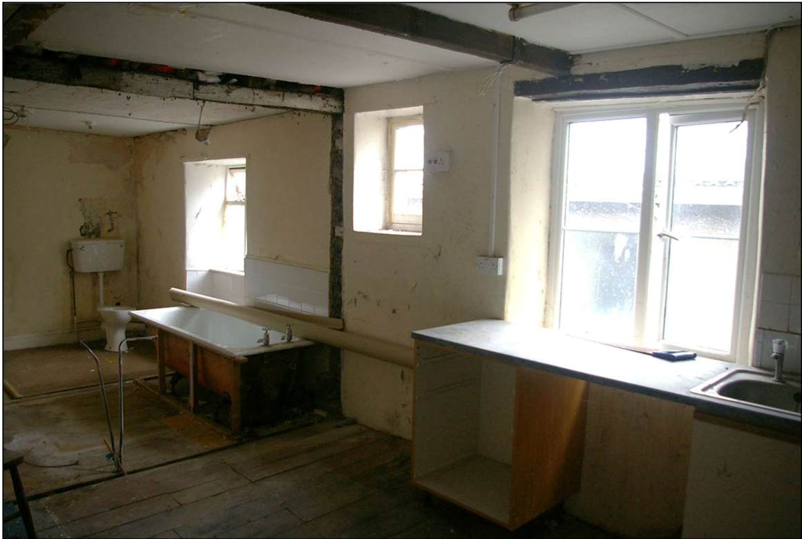
42. THE EAST WALL, ROOM 20, SHOWING W17, W18 AND W19; FROM THE SOUTH-WEST.
