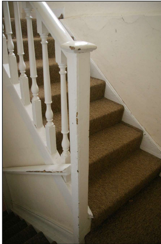
18. RIGHT: THE MOULDED HANDRAIL SERVING THE FIRST FLIGHT AND THE NEWEL POST TO THE HALF LANDING, R5; FROM THE SOUTH-EAST.
