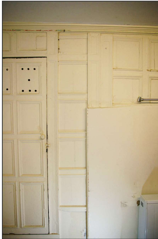
88. THE CUT AND RESET PANELLING AND PILASTERS TO THE SOUTH OF THE BLOCKED FIREPLACE; FROM THE EAST.
