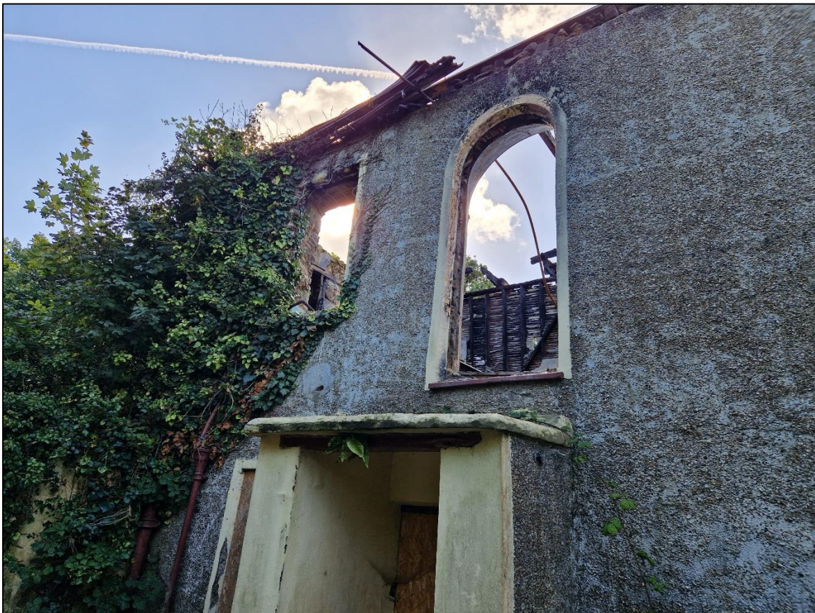
4. CHURCH VIEW, EAST ELEVATION, SHOWING FIRE DAMAGE, VIEWED FROM THE NORTH-EAST.
