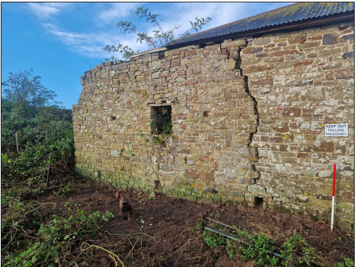
FIGURE 6: EAST ELEVATION FOLLOWING VEGETATION CLEARANCE, SHOWING DRAINS AND SINGLE WINDOW, FROM THE NORTH-EAST (1M SCALE).
