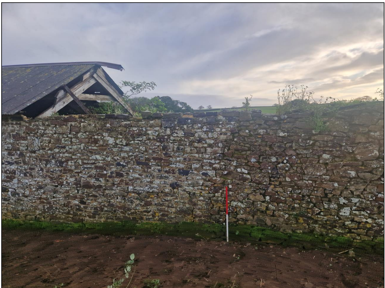
FIGURE 9: THE WEST ELEVATION, SHOWING CHANGE IN BUILD; VIEWED FROM THE SOUTH-WEST (1M SCALE).
