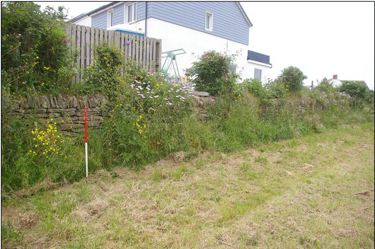
7. DETAIL OF THE STONE WALL BOUNDARY TO THE SOUTH-EASTERN CORNER OF THE SITE; VIEWED FROM THE NORTH-EAST (1M SCALE).
