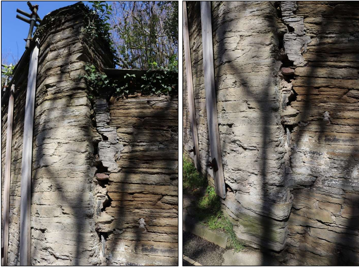
39. LEFT AND RIGHT: DETAIL OF DAMAGE TO THE EAST WALL AGAINST THE FIRST BUTTRESS.
