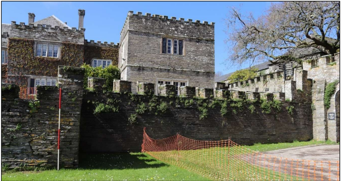
FIGURE 36: THE WALL NORTH OF THE EAST GATE, THE WALL TO THE RIGHT BEING A LENGTHY SECTION OF 19 TH REBUILD; VIEWED FROM THE EAST (SCALE 2M).
