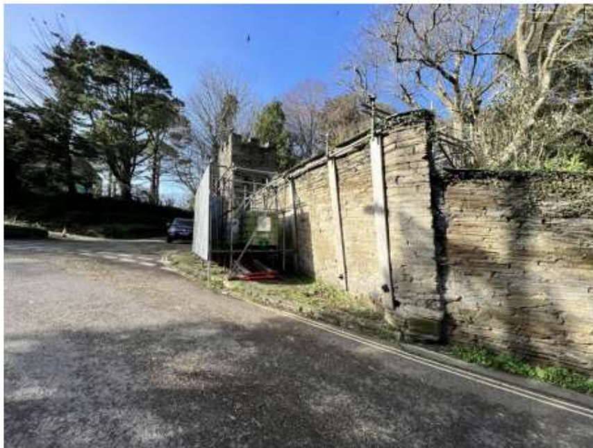
Figure 6 - Boundary wall following Easterly direction ("Front")- Temporary scaffolding supporting leaning wall panels.
