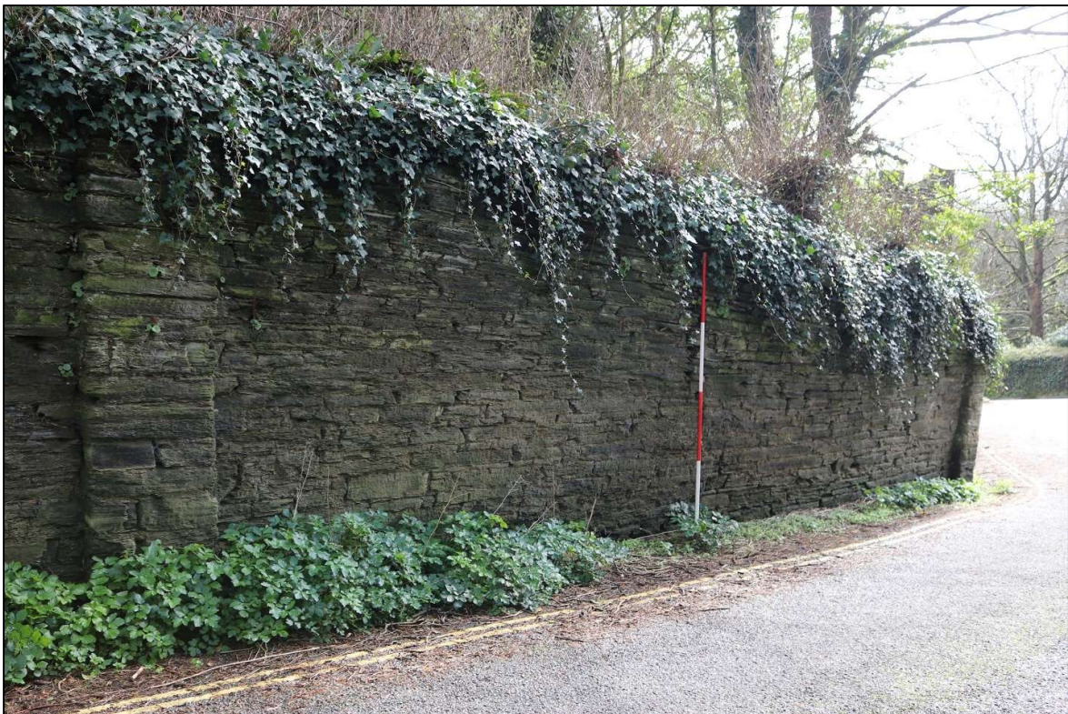
26. THE RETURN WEST WALL WITH NEATLY PROJECTING BUTTRESS, RESPECTING THE LANE; VIEWED FROM THE SOUTH-WEST (SCALE 2M).
