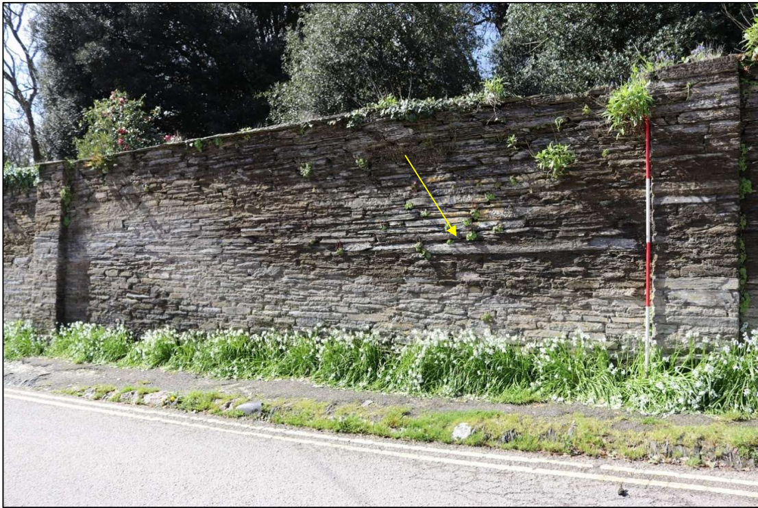
FIGURE 28: SLATE COPING STONES (INDICATED) AS SEEN ALONG THE WALL NORTH OF THE JUNCTION WITH TREGIRLS LANE; VIEWED FROM THE EAST (SCALE 2M).
