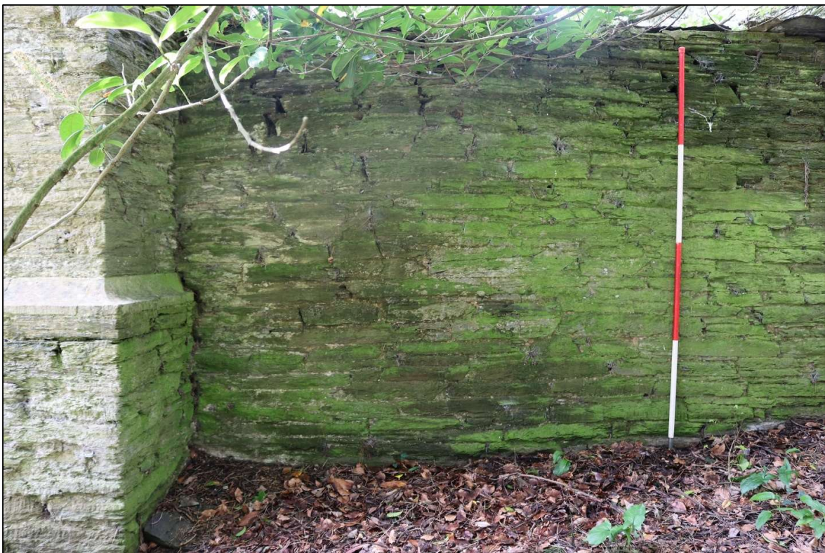
4. THE WEST WALL IS BUILT AROUND WEST PIER TO SOUTH GATE; VIEWED FROM THE NORTH (SCALE 2M).
