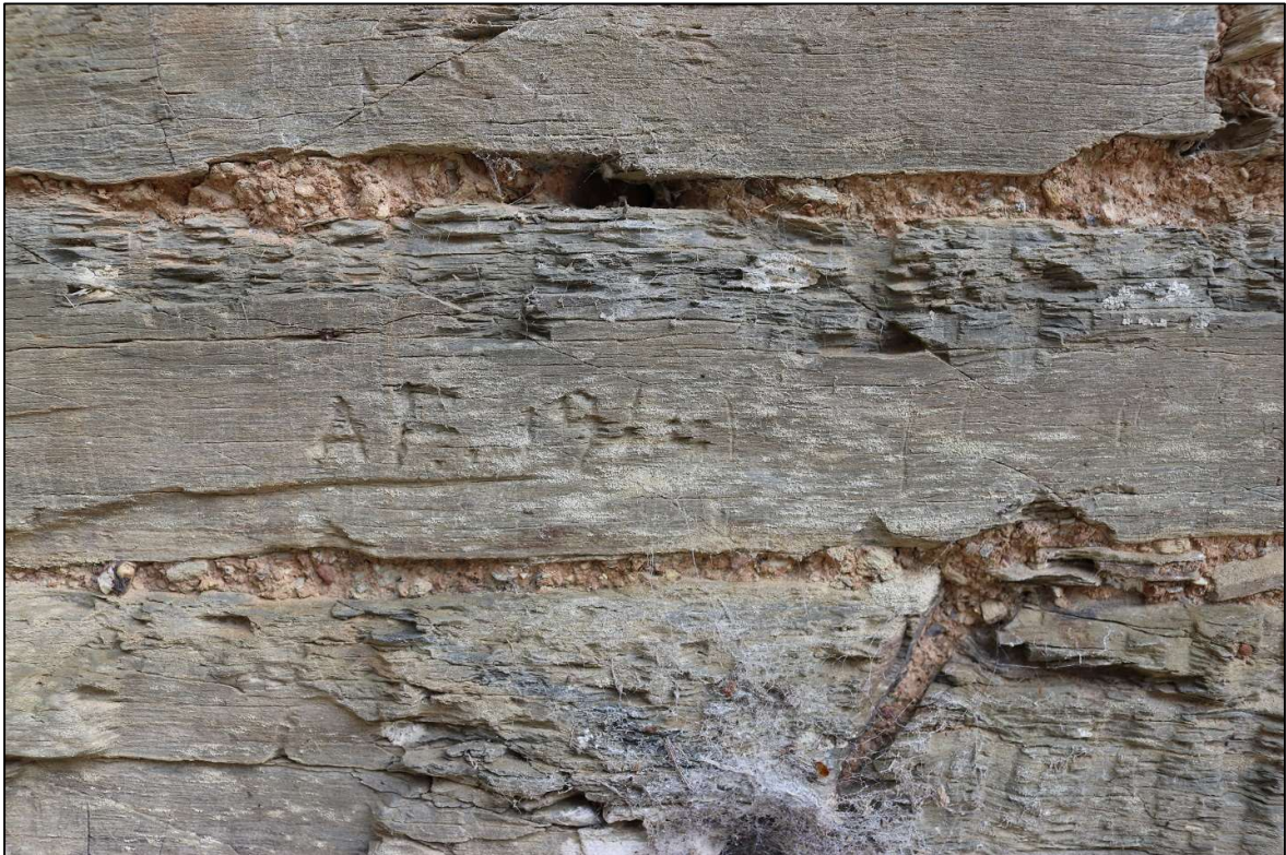
16. THE GRAFFITI SEEN ON SECTION OF WALL AGAINST WEST PIER; VIEWED FROM THE SOUTH.
