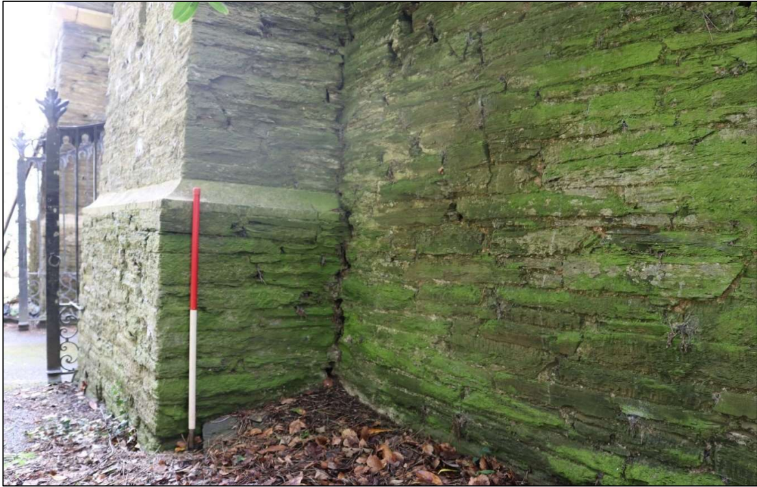
FIGURE 23: THE WEST INTERNAL WALL BUILT OVER AND AROUND WEST PIER; VIEWED FROM THE WEST (SCALE 1M).
