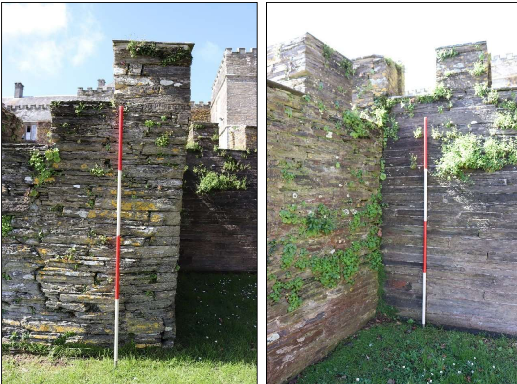
79. THE DETAIL OF A DEEP CHAMFER AT THE NORTH CORNER (LEFT) AND 19 TH C REPLACEMENT WALL MATCHING THAT OF THE FOOTBRIDGE, CONTINUING NORTHWARDS; VIEWED FROM THE EAST (SCALE 2M).
