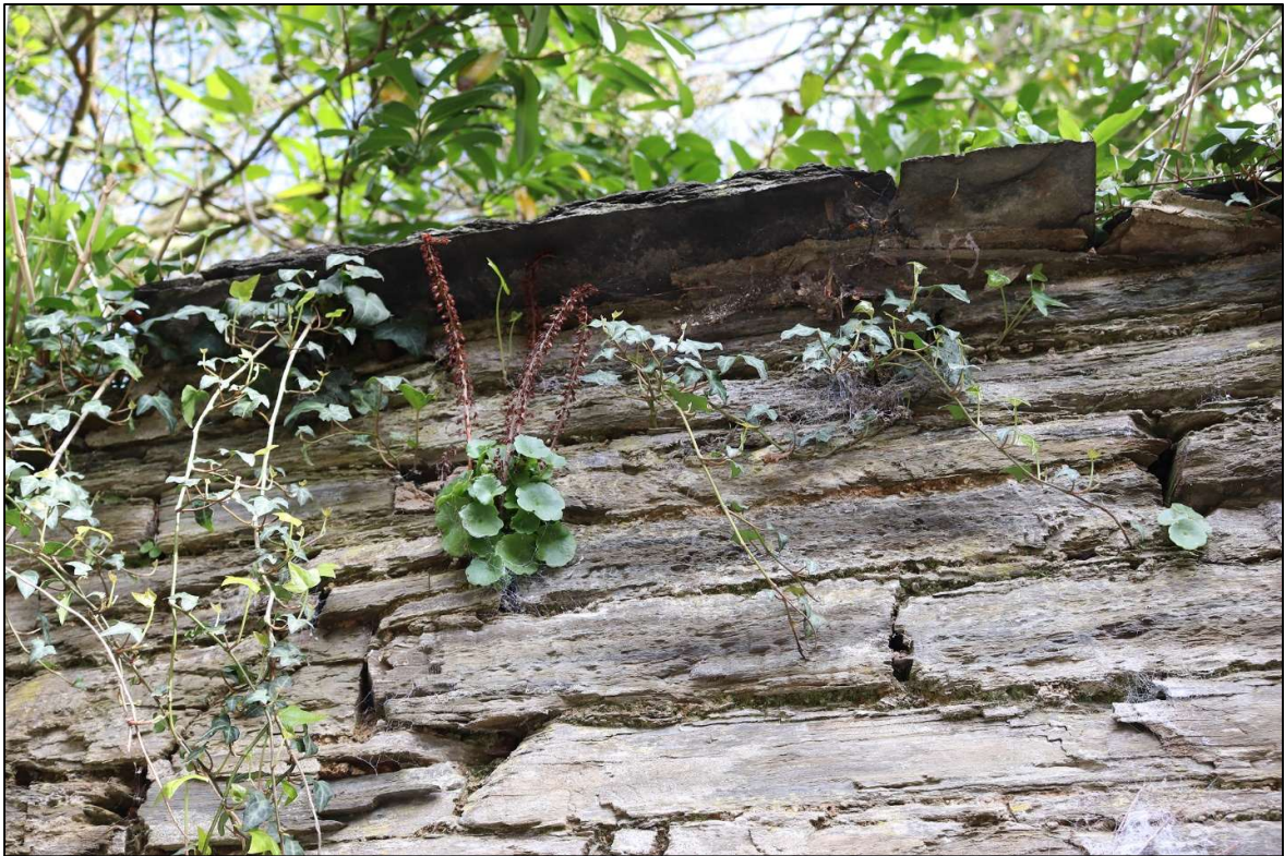
22. THE SLATE TILED TOP OF THE WALL, IN POOR CONDITION, BARELY SURVIVING.
