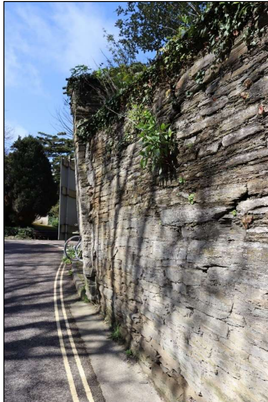
43. THE LEAN CAN BE SEEN FROM THE ROAD ADJACENT TO THE EAST WALL; VIEWED FROM THE NORTH-EAST.
