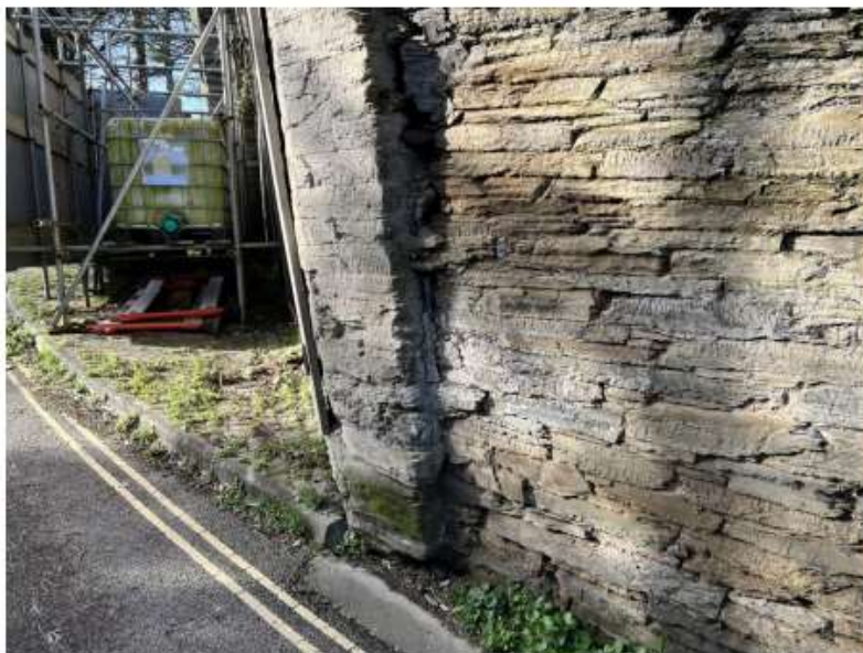
Figure 7 – Boundary wall following Easterly direction ("Front") – Significant leaning to piers and wall panels observed.
