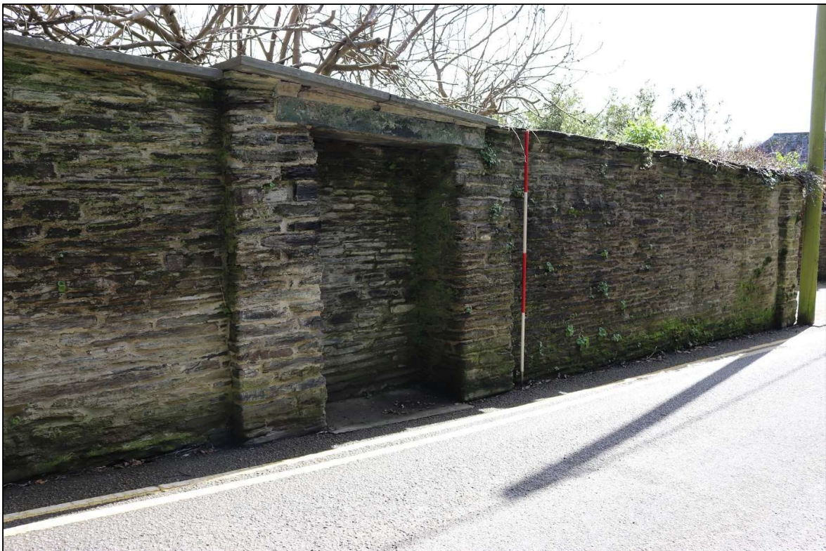
62. THE OPPOSING BLOCKED DOORWAY SEEN IN THE BOUNDARY OF THE NEIGHBOURING DOWER HOUSE; VIEWED FROM THE NORTH-WEST (SCALE 2M).
