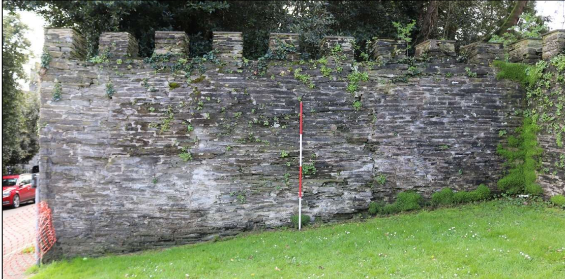
FIGURE 35: THE POSSIBLE BLOCKED OPENING IN THE SOUTH WALL; VIEWED FROM THE NORTH (SCALE 2M).
