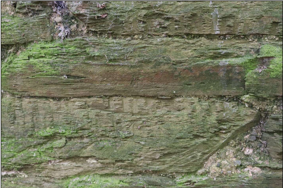
7. QUARRYING SCARS SEEN TO STONWORK ALONG WEST INTERNAL FACE.
