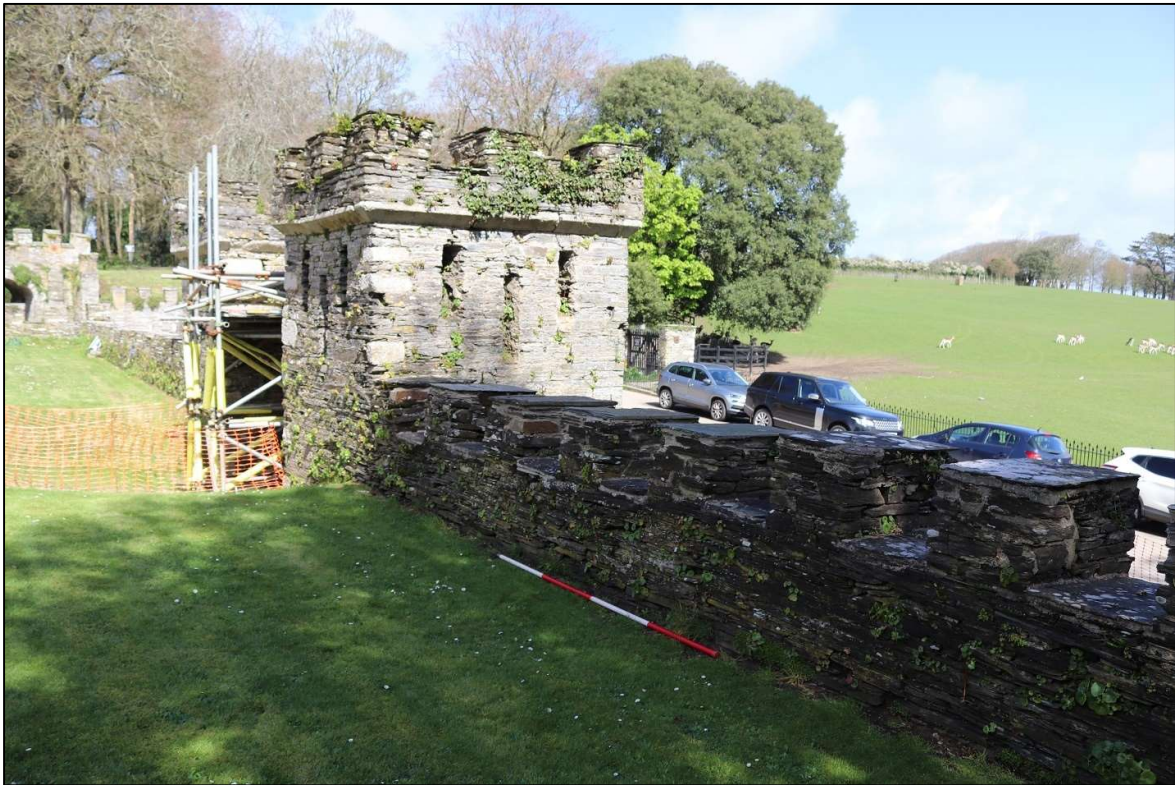
86. THE INTERNAL FACE OF THE SOUTH WALL FROM THE SOUTH PIER OF THE EAST GATE; VIEWED FROM THE SOUTH-WEST (SCALE 2M).
