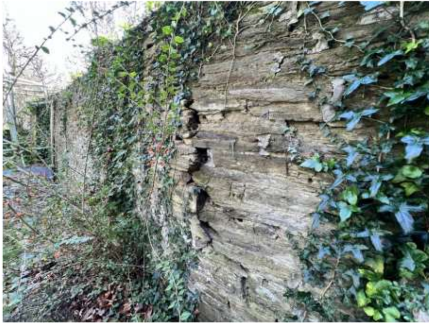
Figure 5 - Boundary wall following Easterly direction ("Rear") - Significant movement observed.
