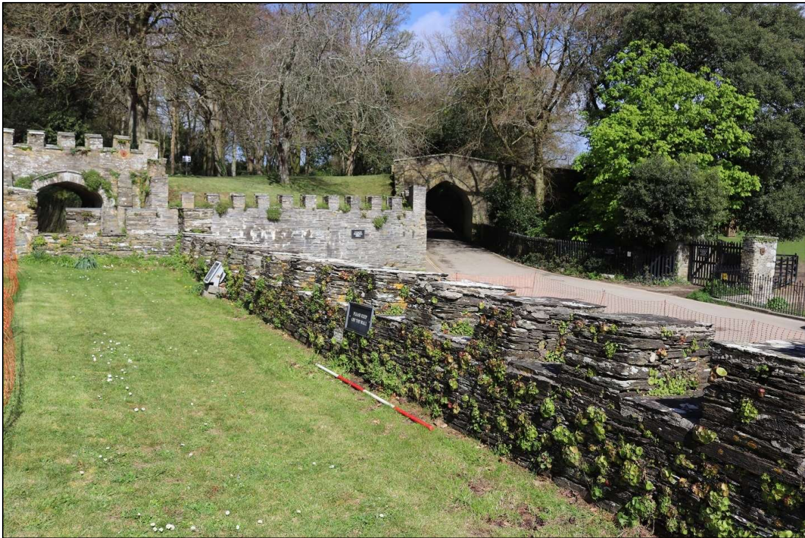
90. THE INTERNAL FACE OF THE NORTH WALL; VIEWED FROM THE SOUTH (SCALE 2M).
