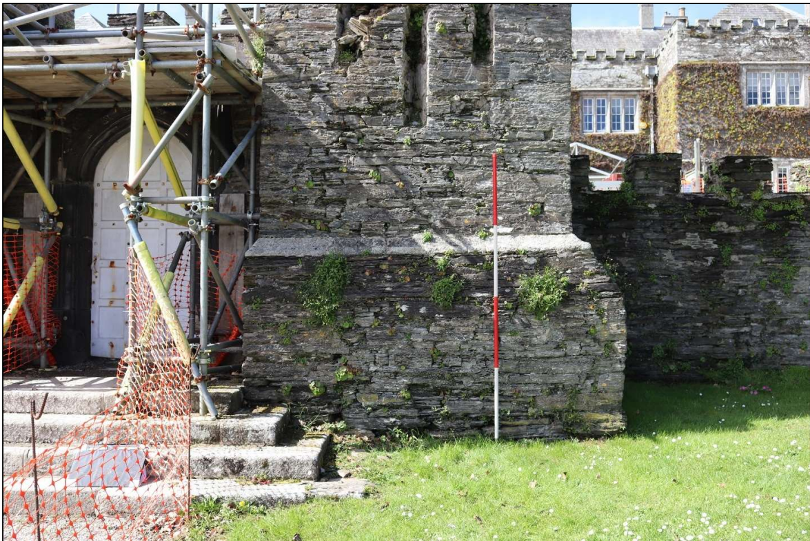
75. THE CRUDER, ROUNDED BASE PLINTH OF THE NORTH PIER; VIEWED FROM THE EAST (SCALE 2M).
