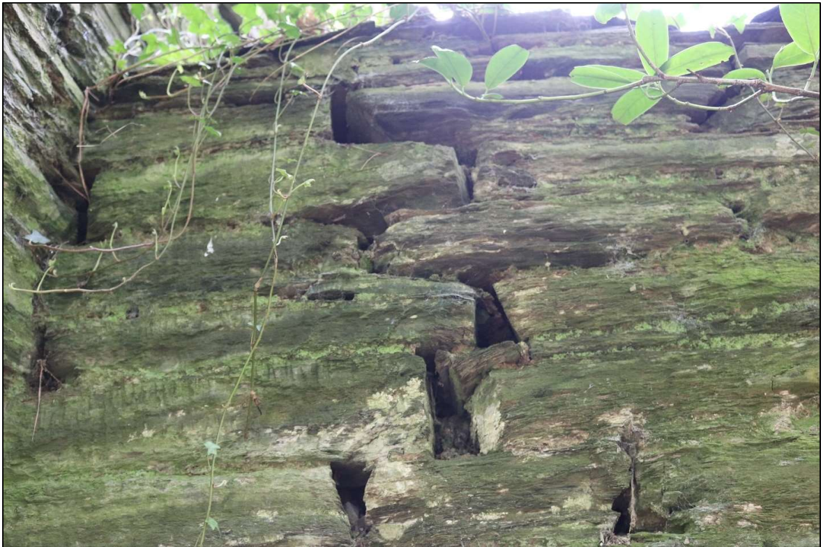
6. STRUCTURAL CRACKING BETWEEN TOP OF WALL AND WEST PIER.
