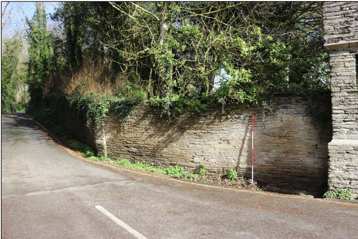
14. THE EXTERNAL FACE OF THE WEST WALL; VIEWED FROM THE SOUTH-EAST (SCALE 2M).
