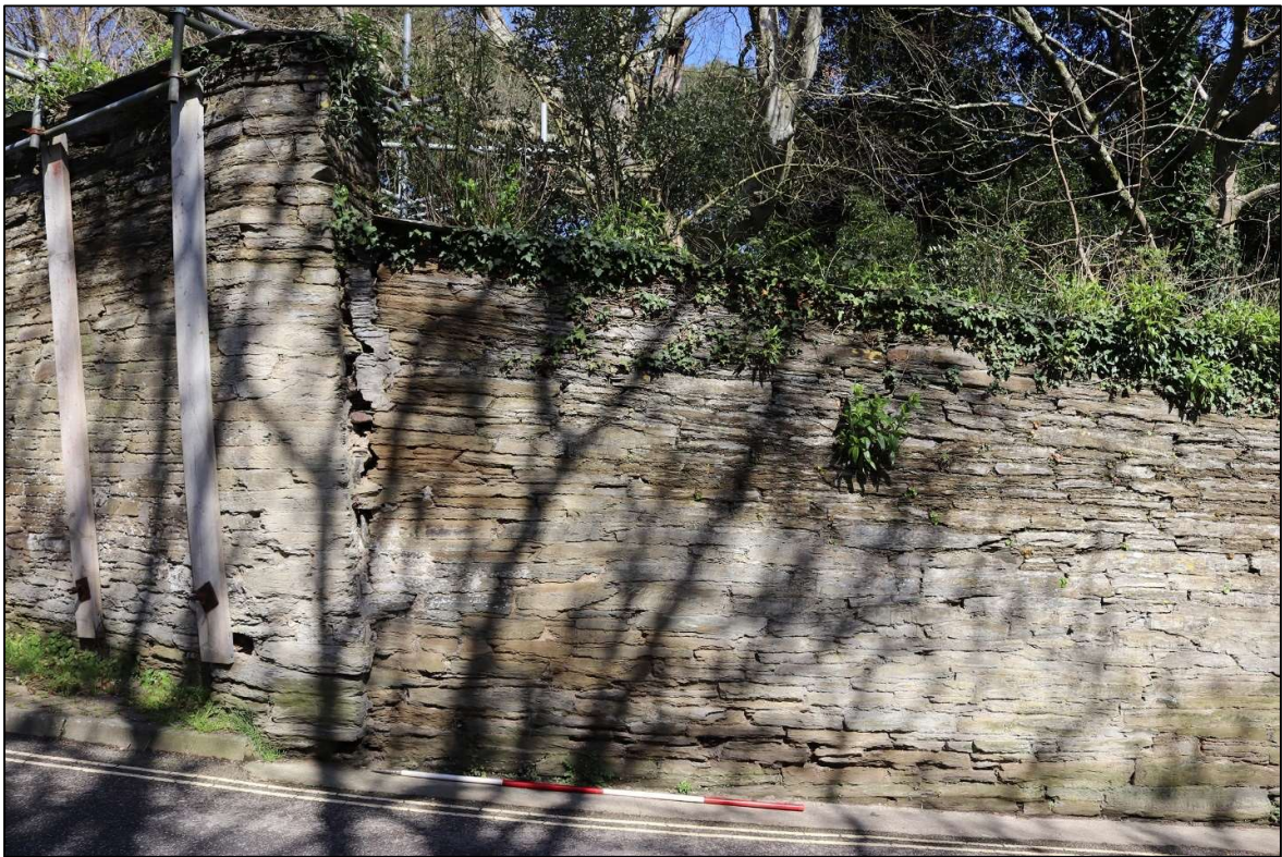
38. STRUCTURAL DAMAGE TO THE EAST WALL; VIEWED FROM THE SOUTH-EAST (SCALE 2M).
