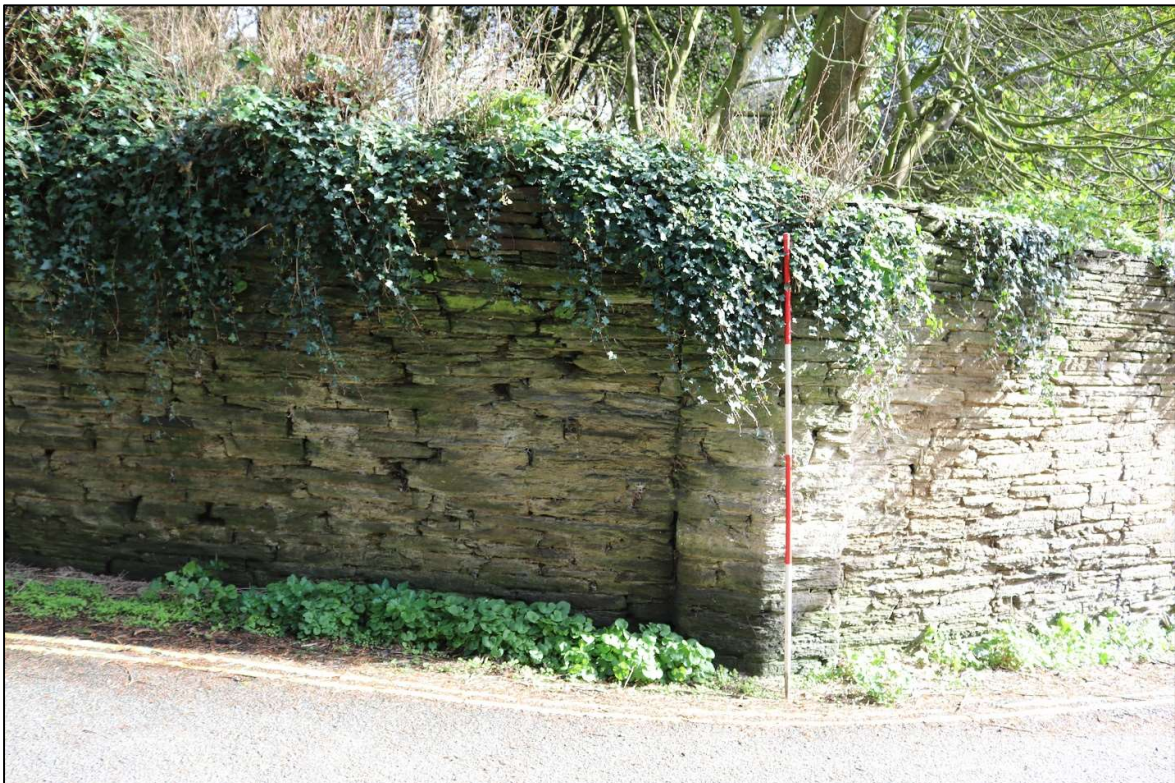
24. THE FIRST BUTTRESS WEST OF THE WEST PIER; VIEWED FROM THE SOUTH (SCALE 2M).
