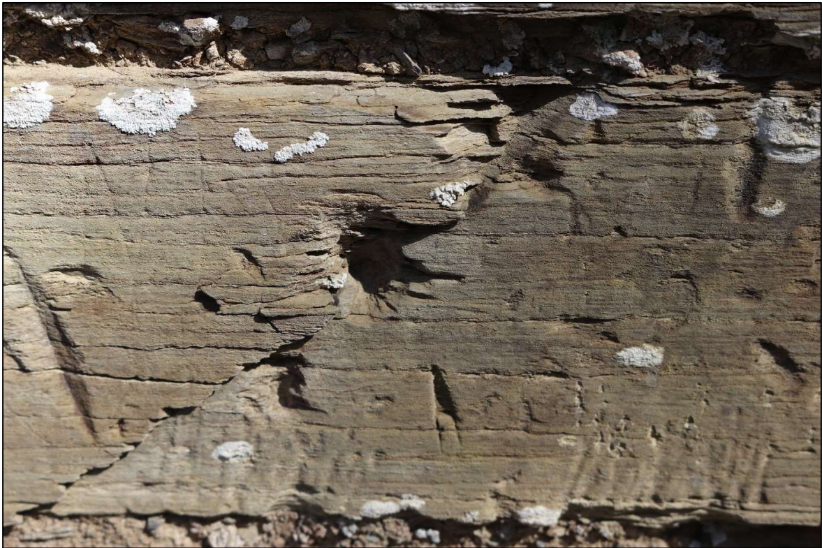
36. THE GRAFFITI SEEN ON SECTION OF WALL AGAINST EAST PIER; VIEWED FROM THE SOUTH.
