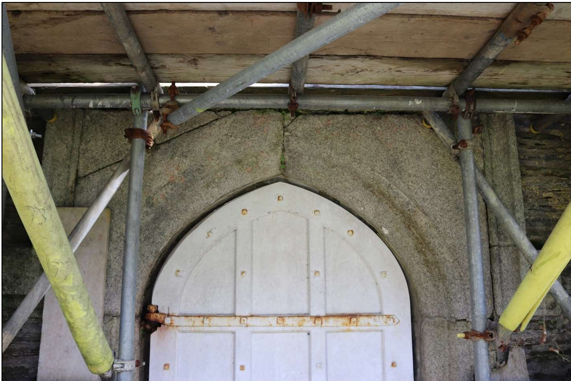
85. THE DETAIL OF THE GRANITE CARVED STONE SURROUND TO THE INTERNAL FACE OF THE EAST GATE; VIEWED FROM THE WEST.
