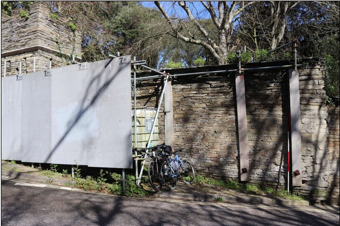
29. THE EAST WALL IS CURRENTLY IN POOR CONDITION AND BRACED WITH TEMPORARY SCAFFOLDING; VIEWED FROM THE SOUTH (SCALE 2M).
