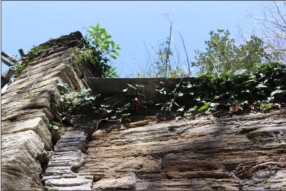
41. THE DAMAGE TO THE EAST WALLS AND FIRST BUTTRESS, CEMENT PATCHING.
