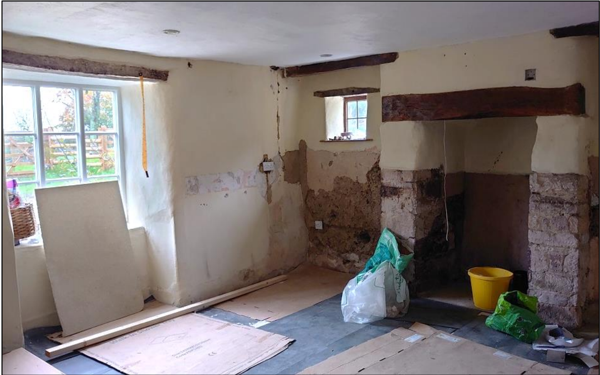
FIGURE 13: R2, THE FORMER KITCHEN OF THE HOUSE, WITH ITS SMALL DOMESTIC, PARLOUR-STYLE FIREPLACE, WITH RAISED AND REPLACED BRESSUMMER BEAM; VIEWED FROM THE SOUTH-EAST.
