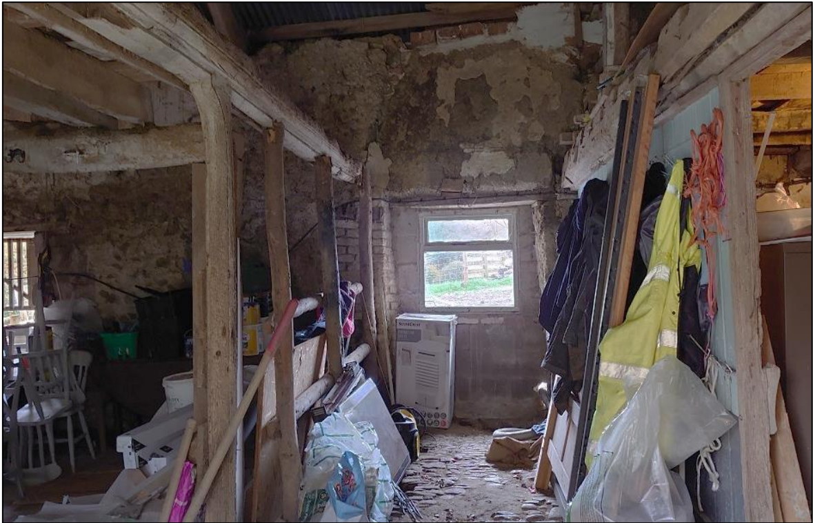
FIGURE 20: R14A, THE 'CROSS-PASSAGE', FORMED BETWEEN 19 TH CENTURY PLANK SCREEN (LEFT) AND INSERTED AND REUSED MEDIEVAL SCREEN (RIGHT); VIEWED FROM THE EAST.
