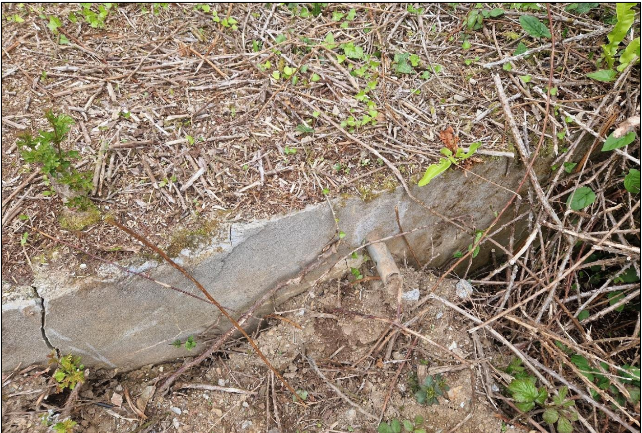
14. CLOSE UP OF A CRACKED CONCRETE BASE WITH A DRAINAGE PIPE PROJECTING; FROM THE SOUTH.
