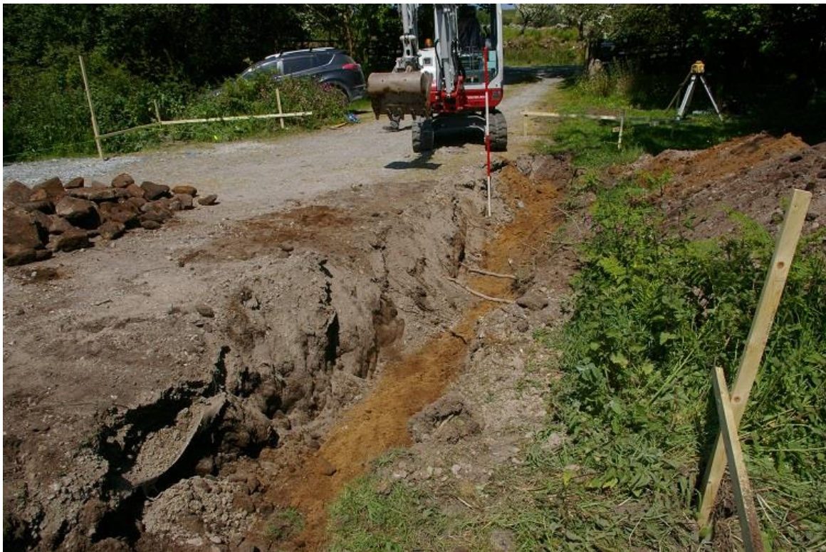
FIGURE 3: T2, SHOWING THE DEPTH OF THE MADE GROUND LAYER LAID OVER SHEETING, VIEWED FROM THE SOUTH -WEST (2M SCALE).
