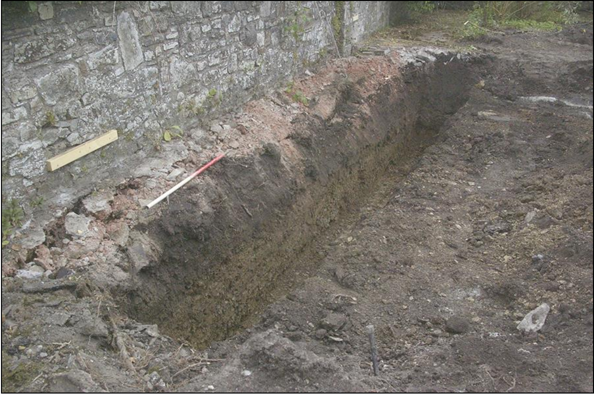
FIGURE 2: EASTERN FOOTING TRENCH, SHOWING NORTH-EAST SAMPLE SECTION; VIEWED FROM THE NORTH-WEST (1M SCALE).
