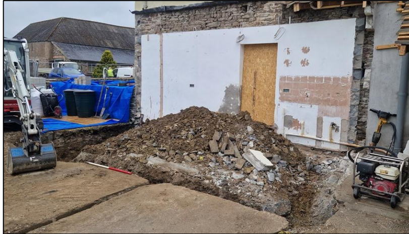
FIGURE 11: WORKING SHOT OF THE SITE OF THE DEMOLISHED EXTENSION AND EXCAVATED FOOTINGS, WITH CONCRETE APRON, FROM THE NORTH (1M SCALE).
