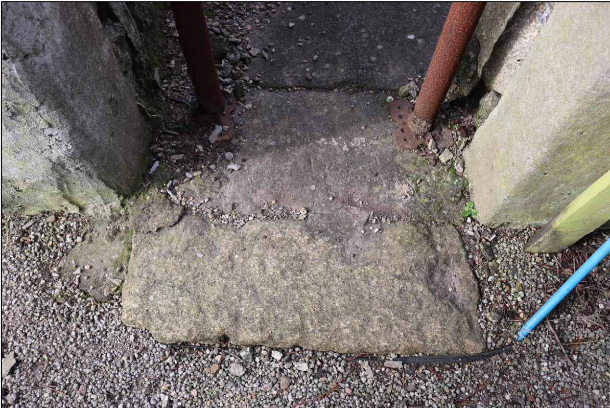
9. GRANITE THRESHOLD FOR ABOVE OPENING. MOUNTED WITHIN MODERN LANDSCAPING FABRIC AND LOOSE GRAVEL.
