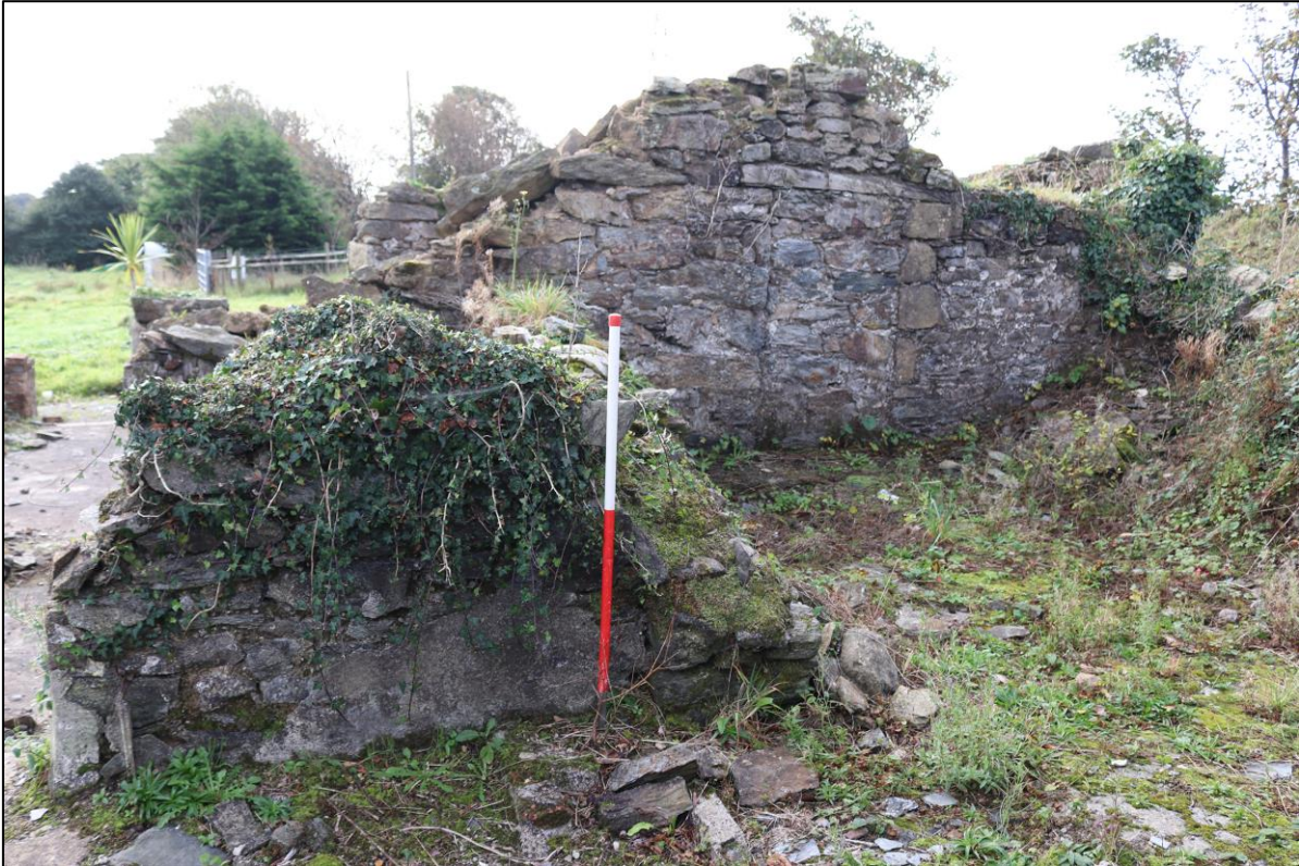
15. THE NORTH ELEVATION OF WEST BLOCK WITH BLOCKED DOORWAY; FROM THE NORTH WITH 1M SCALE.
