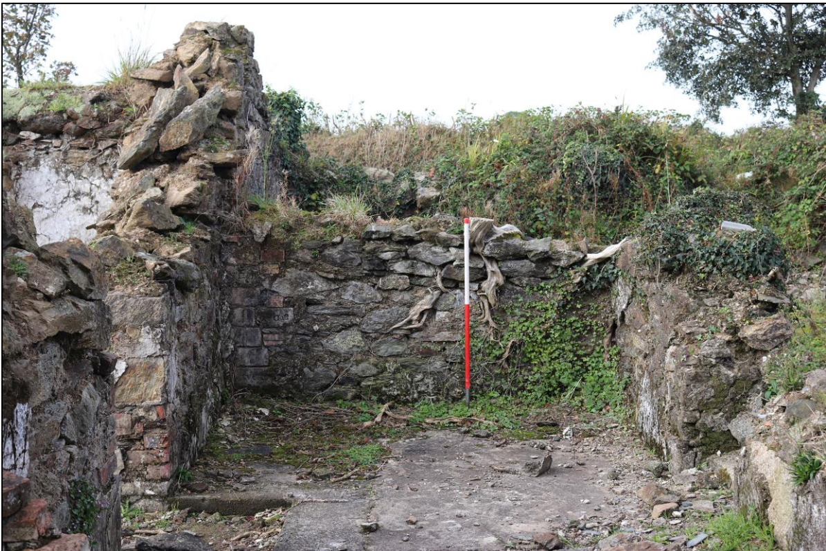
22. THE WEST OF THE LEAN-TO BUILT WITH BRICK TO THE CORNER NOT SEEN ELSEWHERE TO MASONRY, THICKNESS WALL TO THIS END DIFFERED FROM THE EAST. FROM THE EAST WITH 1M SCALE.
