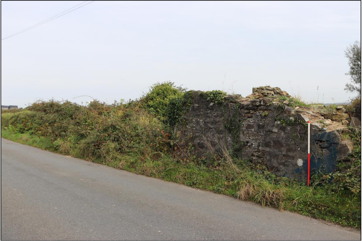
51. THE WEST ELEVATION RESPECTING OLD PORTREATH ROAD. FROM THE SOUTH-WEST WITH 1M SCALE.
