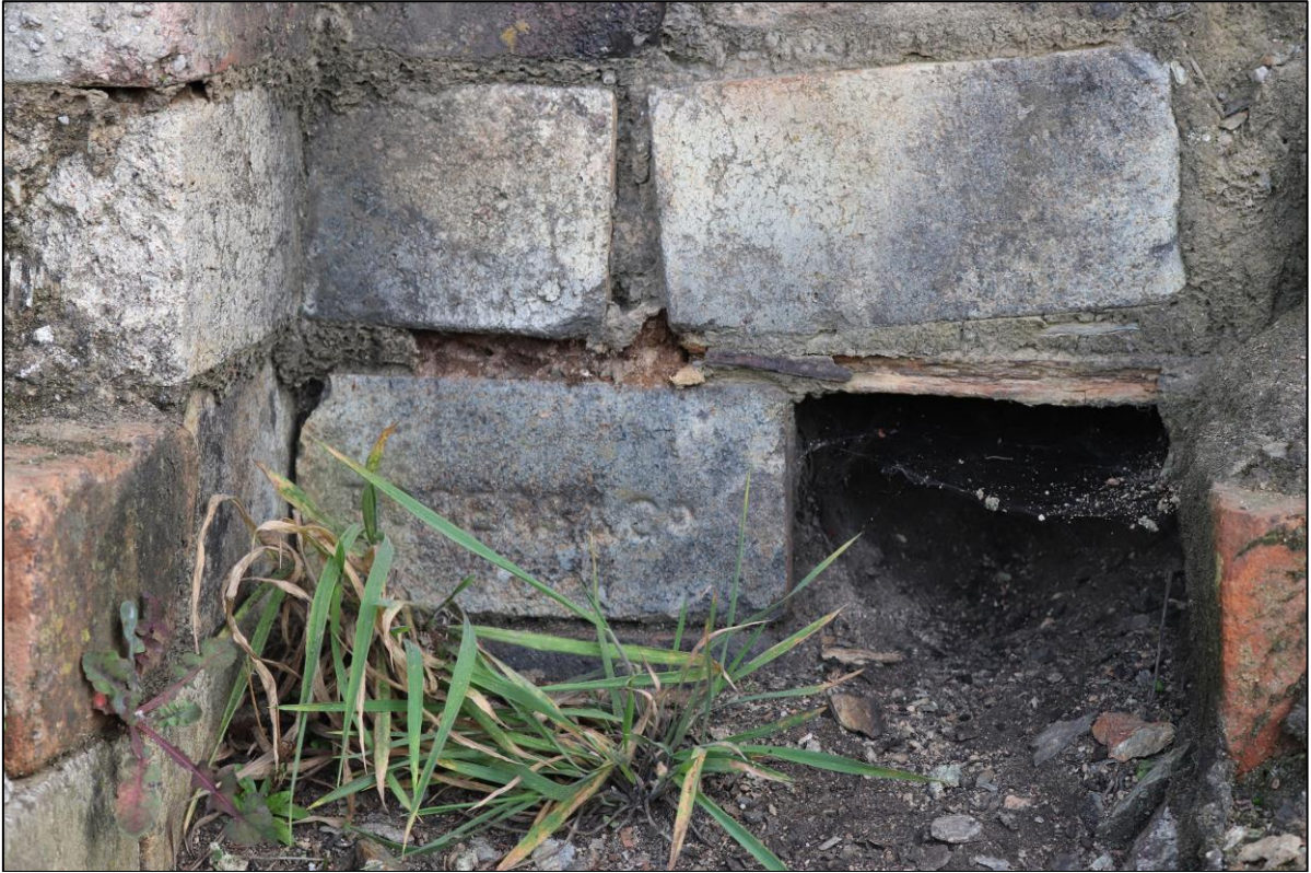
31. THE ROGER & CO BRICK SEEN TO ALTERATIONS MADE TO FIREPLACE. FROM WEST.
