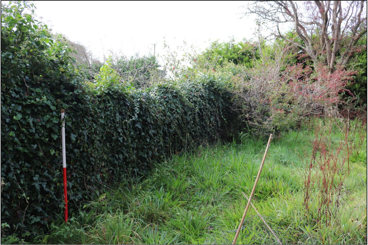
43. THE SOUTH RUBBLE WALL OF GARDEN OVERGROWN, FROM THE EAST WITH 1M SCALE.
