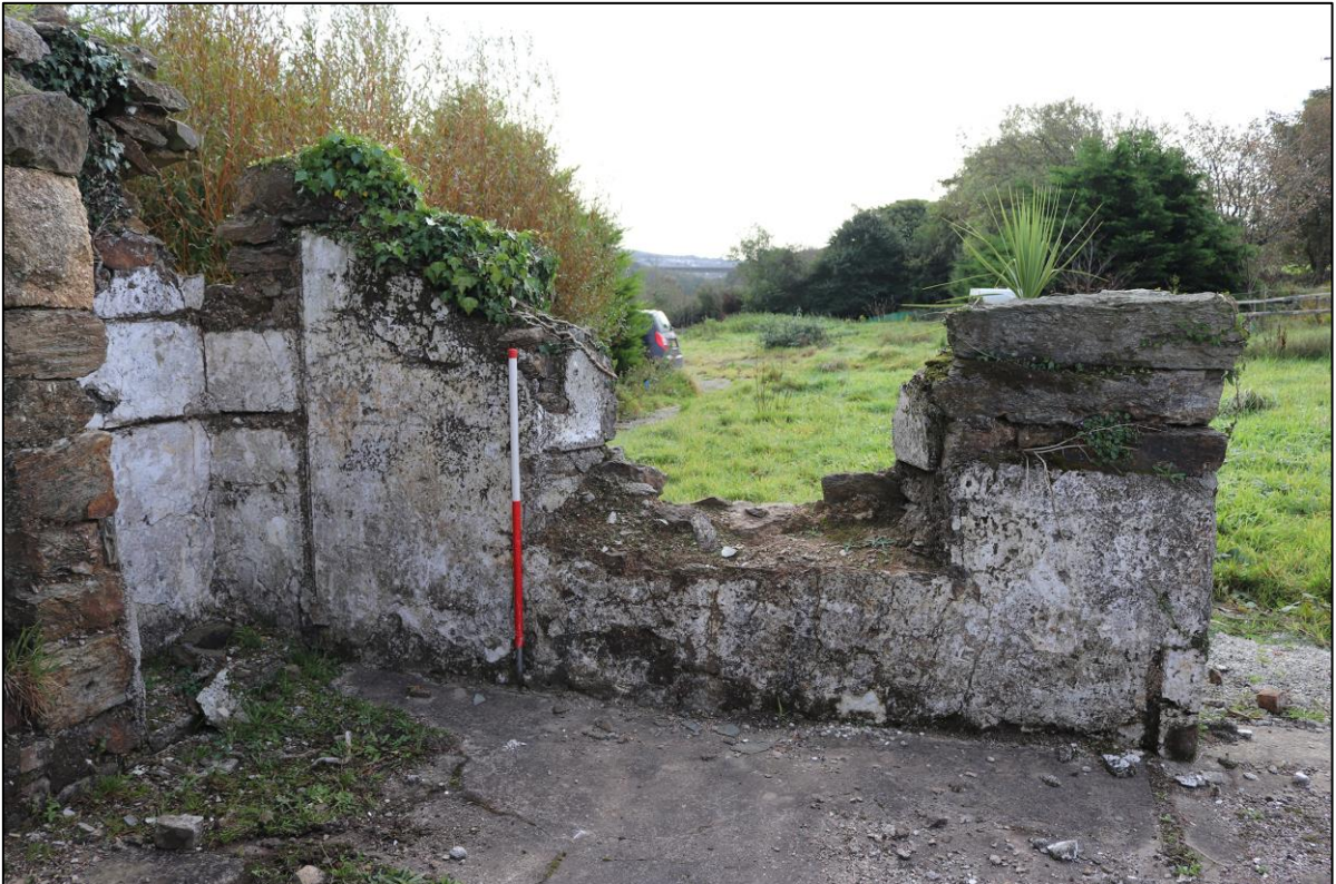
32. THE EAST WINDOW OPENING FOR C1, FROM THE NORTH-WEST WITH 1M SCALE.
