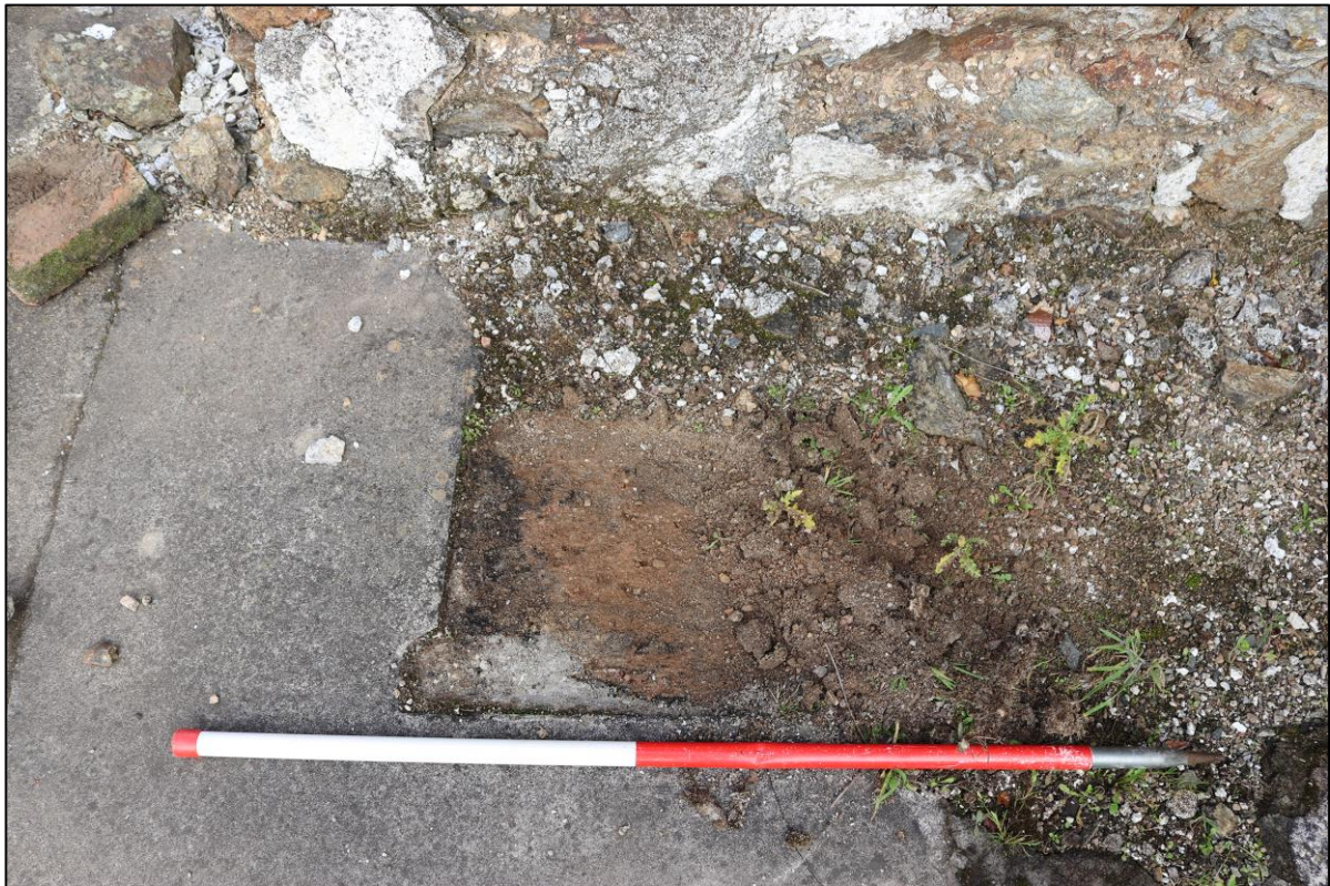
FIGURE 14: BENEATH SCREED LAYER A PACKED EARTH FLOOR IS VISIBLE. THE SHAPE TO THE WEST SIDE REFLECTS THE POSSIBLE BASE OF A NARROW STAIRCASE THAT ROSE AGAINST THE NORTH ELEVATION. THIS IS REFLECTED SIMILARLY TO C2. TAKEN FROM ABOVE FROM NORTH WITH 1M SCALE.
