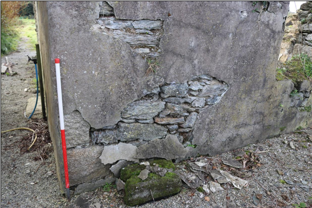
11. CORNER OF NORTH LEAN-TO, KILLAS RUBBLE AND GRANITE QUOINS UNDER MID-20THC RENDER; FROM THE NORTH WITH 1M SCALE.
