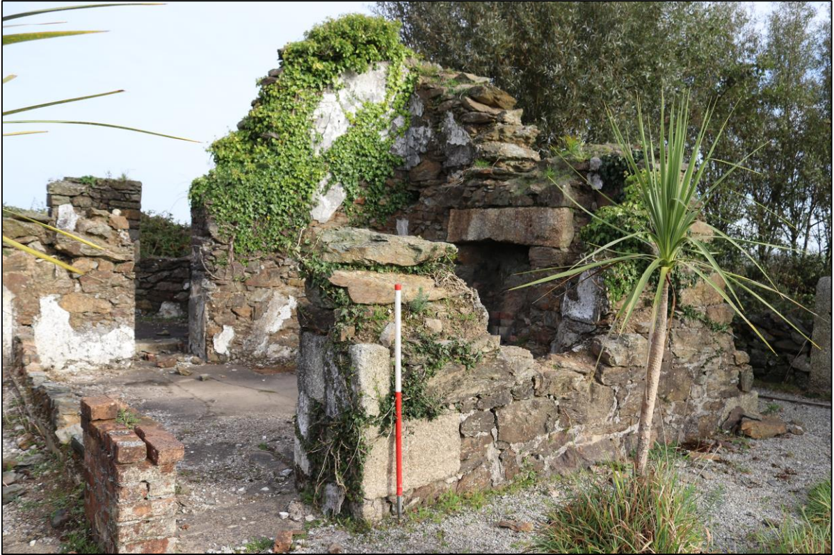
3. C1 EXTERIORS, BRICK PIER SHOWING DIVISION OF DOOR OPENING. FROM THE SOUTH-WEST WITH 1M SCALE.
