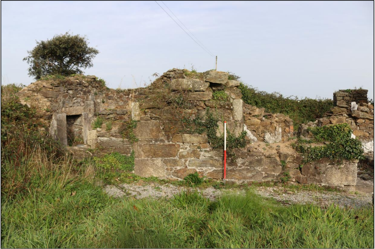
5. THE WEST EXTENSION BLOCK BUILT AGAINST QUOIN DETAILING OF THE MAIN RANGE; FROM THE SOUTH WITH 1M SCALE.
