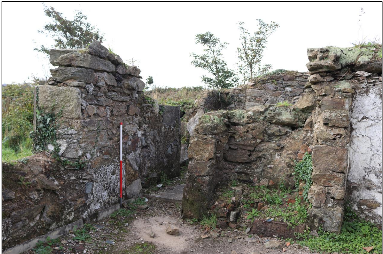
FIGURE 10: BREACHED OPENING TO THE SOUTH-WEST CORNER OF C2 AGAINST SOUTH SIDE OF STACK, TAKEN FROM EAST WITH 1M SCALE.
