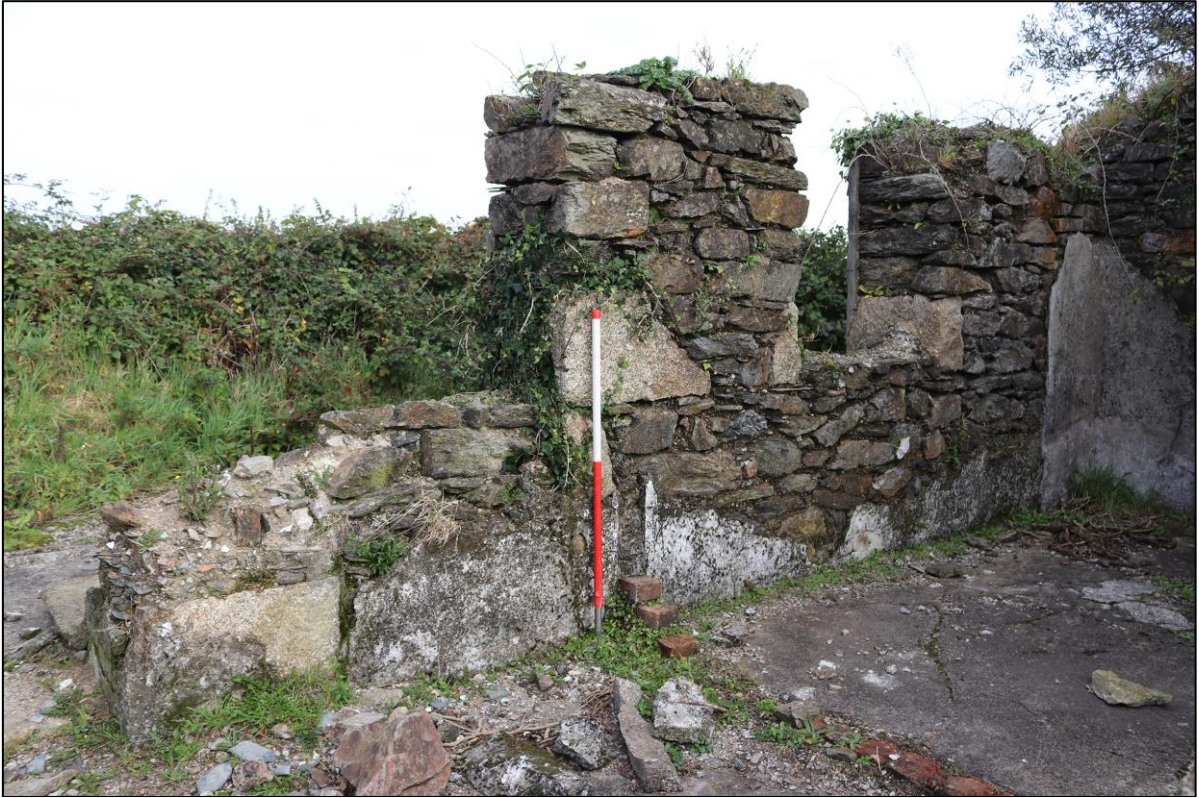
25. THE NORTH- EAST END BUILD LINE APPARENT, IMPLYING TWO PHASES OF LEAN-TO. FROM THE SOUTH WITH 1M SCALE.
