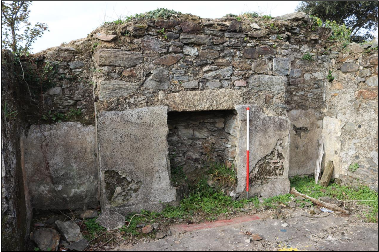
FIGURE 12: PROJECTING STACK TO WEST ELEVATION OF WEST BLOCK, INCLUDING PATCHING WITH BRICK AND SHORT LINTEL, FROM THE EAST WITH 1M SCALE.
