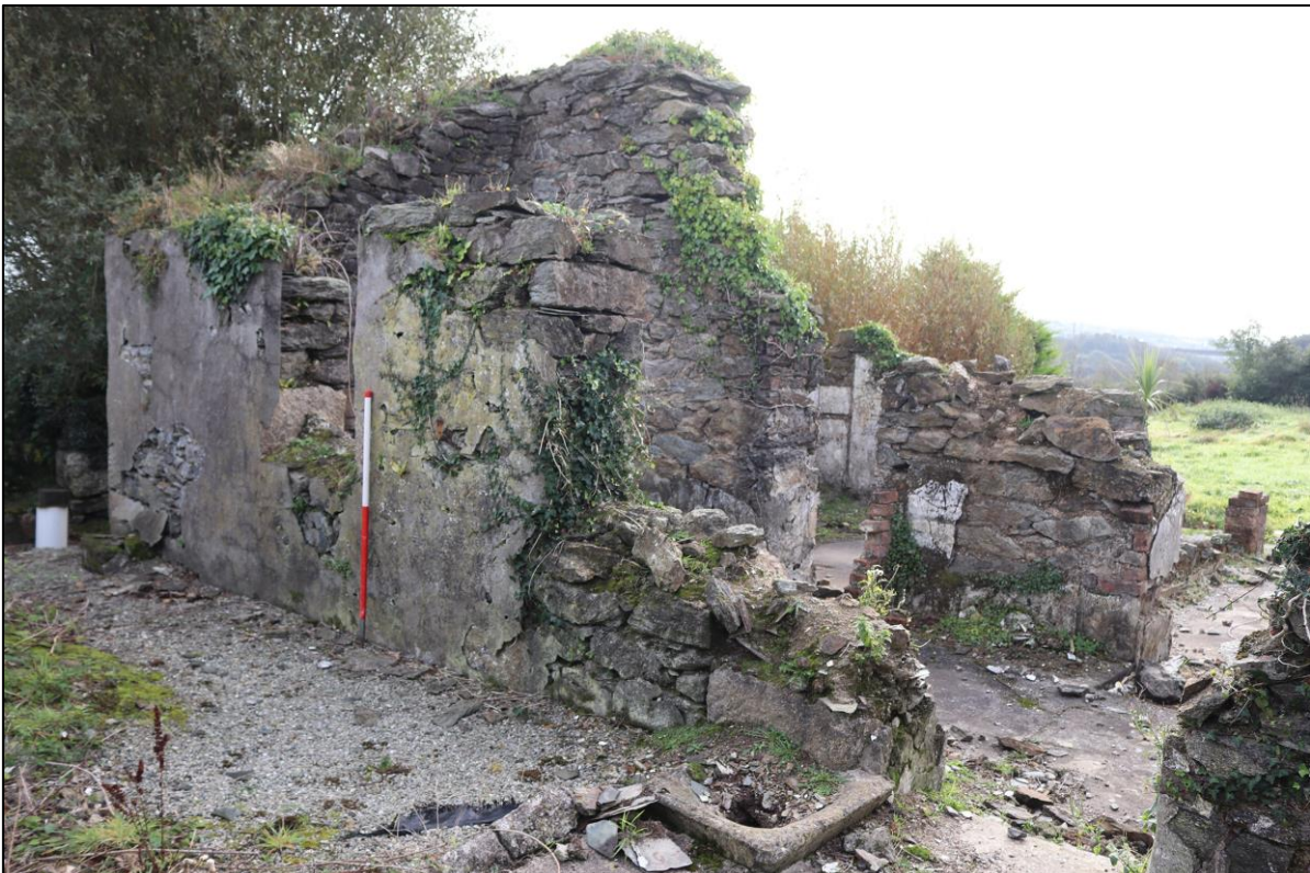
12. THE NORTH ELEVATION OF LEAN-TO SHOWING SHALLOW MONO-PITCH; FROM THE NORTH-WEST WITH 1M SCALE.
