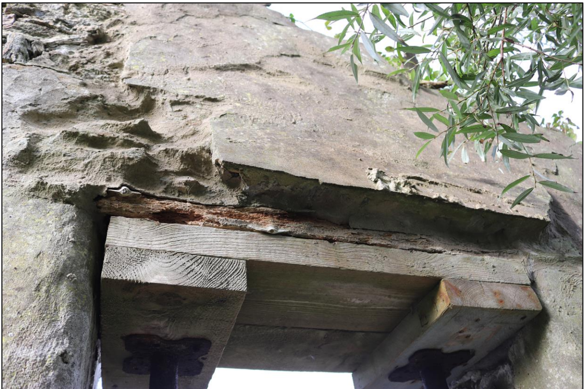
8. OPENING TO THE EAST SIDE OF NORTH LEAN-TO MODERN PINE SLABS PROP OLDER RUSTIC LINTEL. ABOVE HAS BEEN SHAPED WITH RENDER TO CREATE RUN-OFF.
