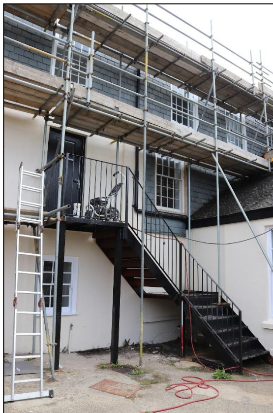
FIGURE 8: SLATE HANGING CONTINUES TO THE FF (MODERN) THE STAIRS HAVE BEEN RECYCLED FROM THOSE WHICH EXISTED INTERNALLY. TAKEN FROM THE NORTH-WEST WITH 1M SCALES.
