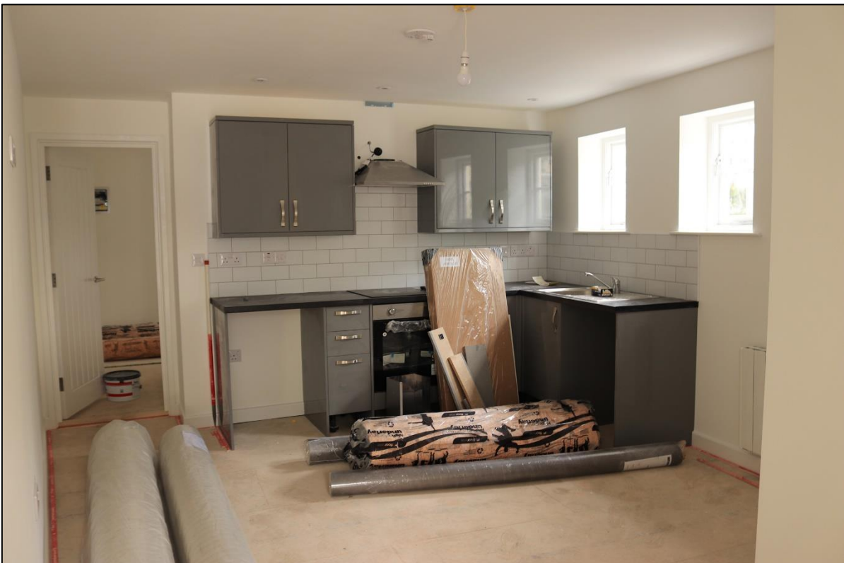
6. REAR CONVERTED GF FLAT; NO HISTORICAL FEATURES EXPOSED/ SURVIVE. TAKEN FROM THE NORTH WITH 1M SCALE.
