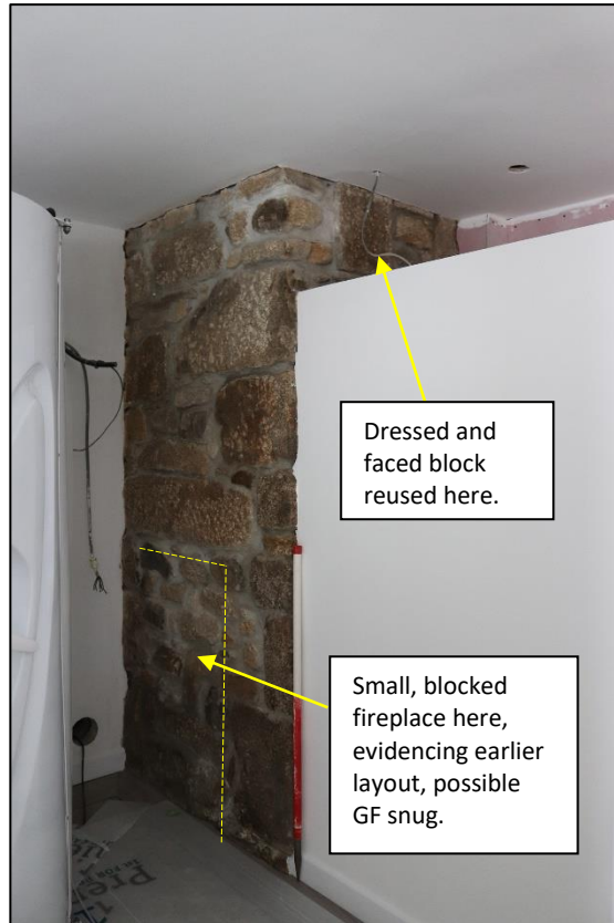
FIGURE 13: SMALL BLOCKED FIREPLACE TO THE WEST WALL WITHIN NEW CUBICLES, MATCHING LOCATION TO THE SMALL BLOCKED FIREPLACE TO WEST FLAT ABOVE, INCLUDING REUSED DRESSED AND FACED GRANITE BLOCK. TAKEN FROM THE SOUTH-WEST, WITH 1M SCALES.
