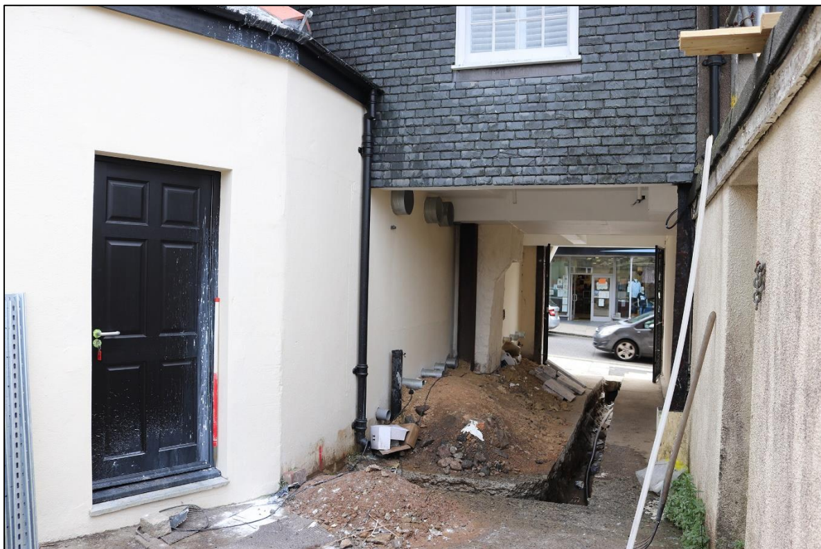
FIGURE 9: THE NORTH FACING REAR OF CARRIAGE PASSAGE WITH (MODERN) SLATE HANGING. TAKEN FROM THE NORTH WITH 1M SCALES.
