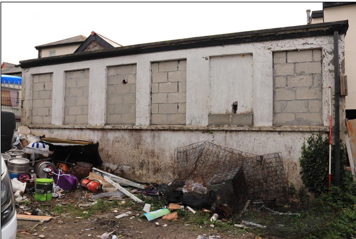
4. THE REAR 20 TH CENTURY STORAGE BLOCK; FROM THE NORTH WITH 2M SCALE.
