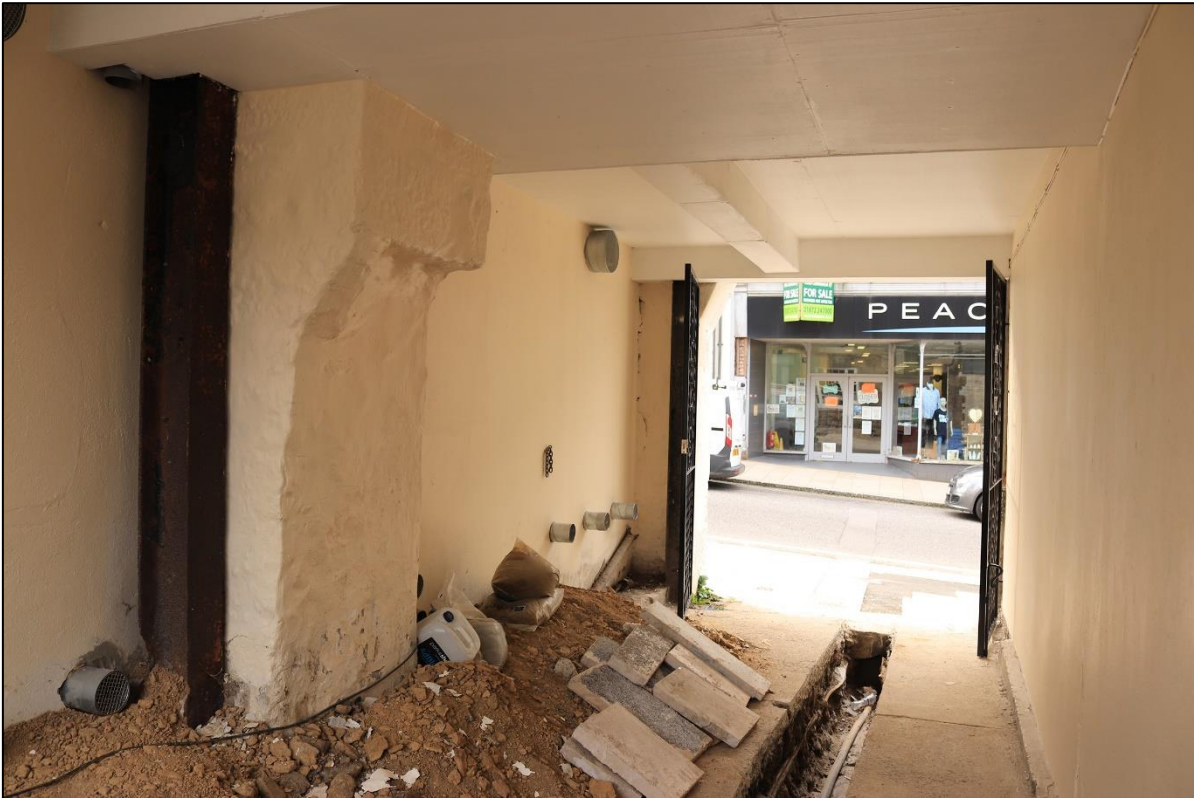
3. THE CARRIAGE PASSAGE FROM THE NORTH LOOKING BACK TO FORE STREET, SHOWING POTENTIAL CUT STACK WITH GRANITE DRESSINGS UNDER PAINTWORK; FROM THE NORTH.
