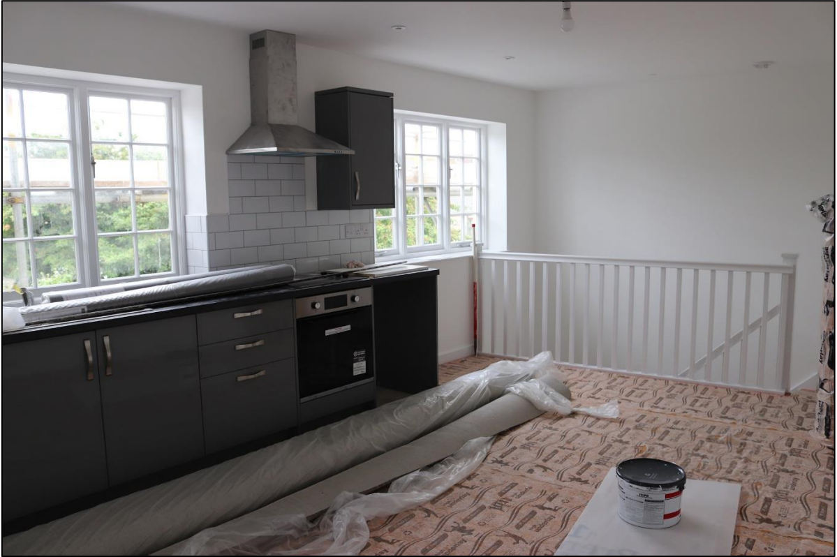
7. REAR FF FLAT; NO HISTORICAL FEATURES SURVIVE. TAKEN FROM THE SOUTH-EAST WITH 1M SCALES.
