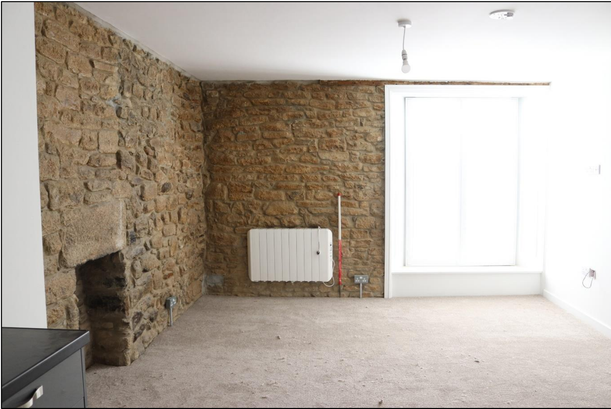
11. THE FF EAST FLAT, WITH EXPOSED FP AND MARKED DIFFERENCES IN MASONRY; FROM THE NORTH WITH 1M SCALE.
