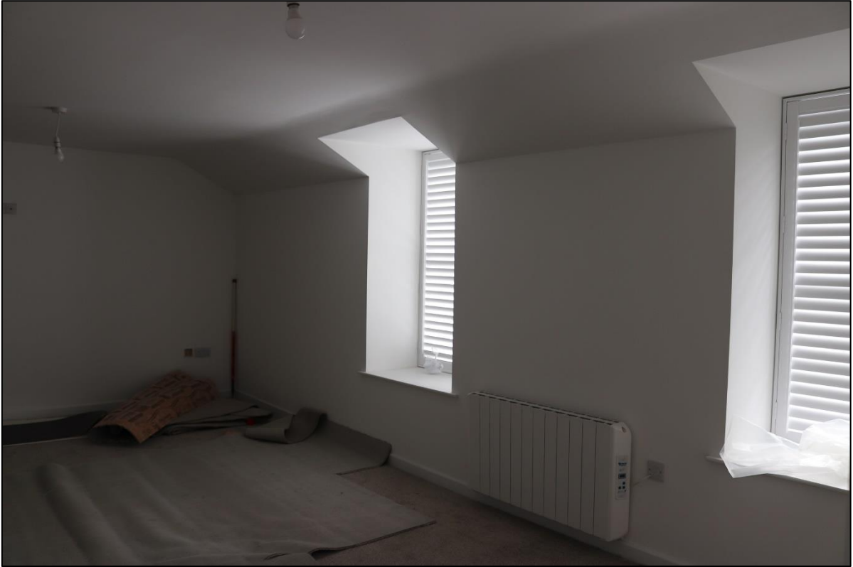
17. THE SF FLAT WITH NO SURVIVING FEATURES VIEW OF THE FRONT WINDOWS; FROM THE WEST.
