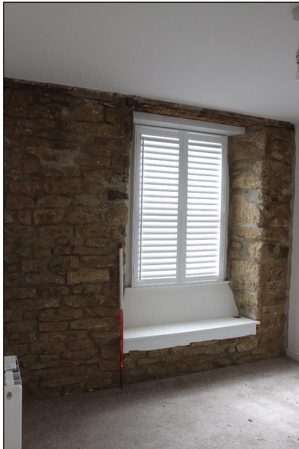
12. EXPOSED WALLING IN NEIGHBOURING BEDROOM ON THE 18 TH CENTURY FRONTAGE; FROM THE NORTH-WEST WITH 1M SCALE.
