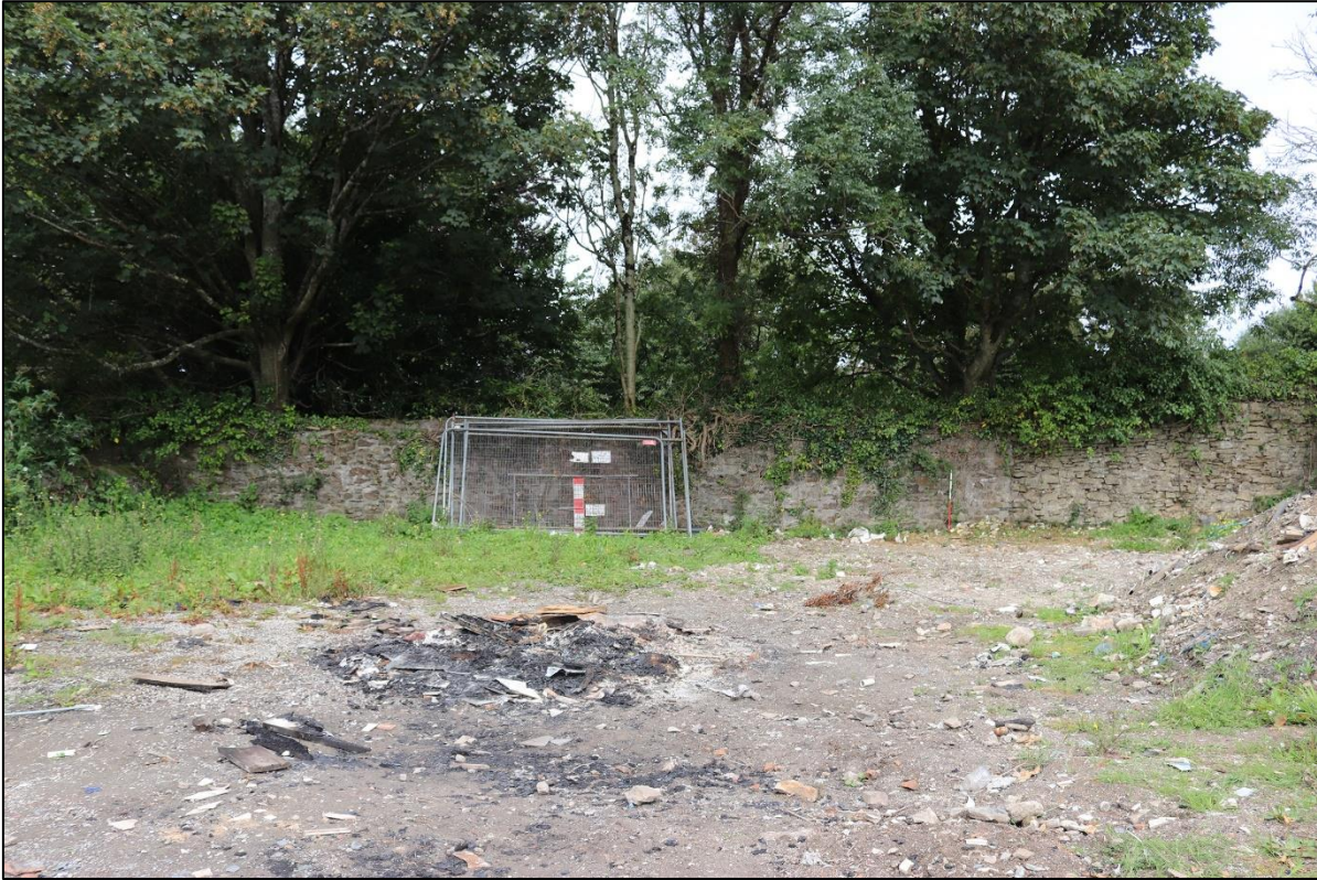
31. THE REAR NORTH COMPOUND WALL WITH BLOCKED OPENINGS; FROM THE SOUTH WITH 1M SCALE.
