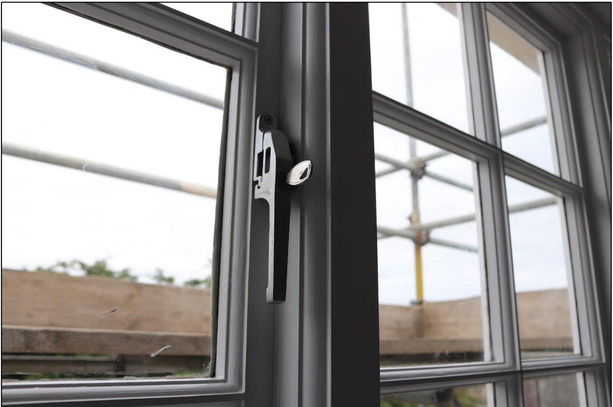
8. ALL WINDOWS WERE FULL REPLACEMENTS.
