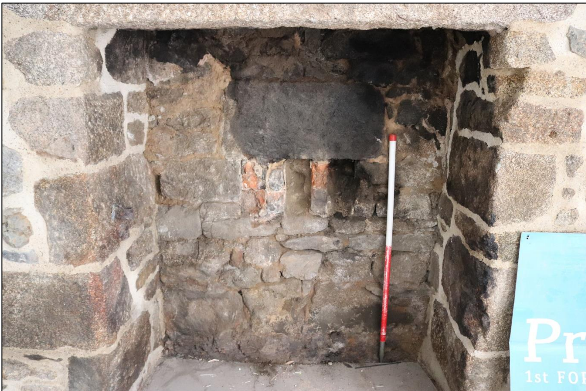
20. THE BACK PLATE OF STACK SHOWING DISTURBANCE FOR LATER STOVE FITTINGS; FROM THE WEST WITH 1M SCALES.
