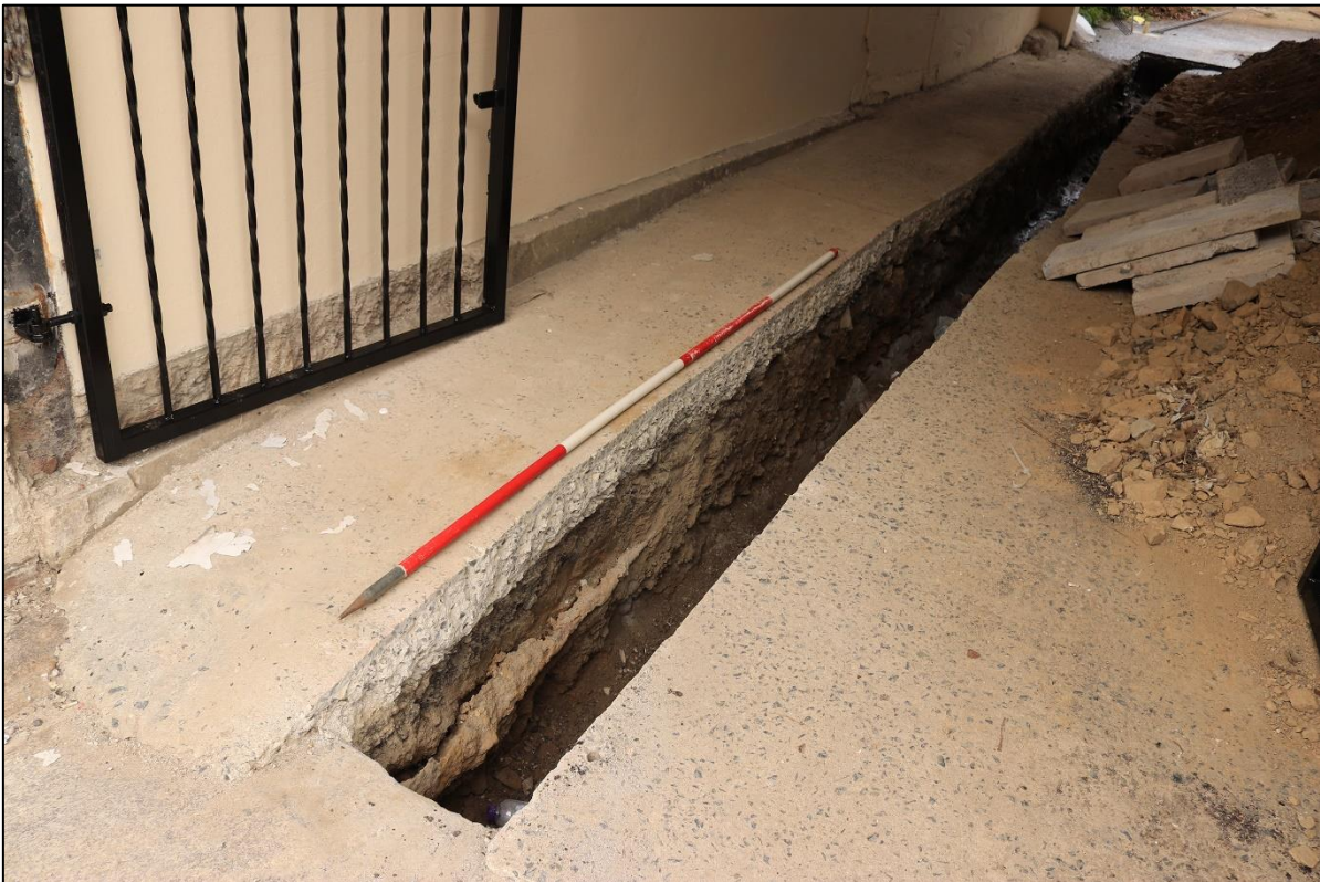
2. UNMONITORED GROUNDWORKS TO THE CARRIAGE PASSAGE SHOWING LATER DISTURBANCE AND RELAYING. TAKEN FROM THE SOUTH-EAST WITH 2M SCALE.
