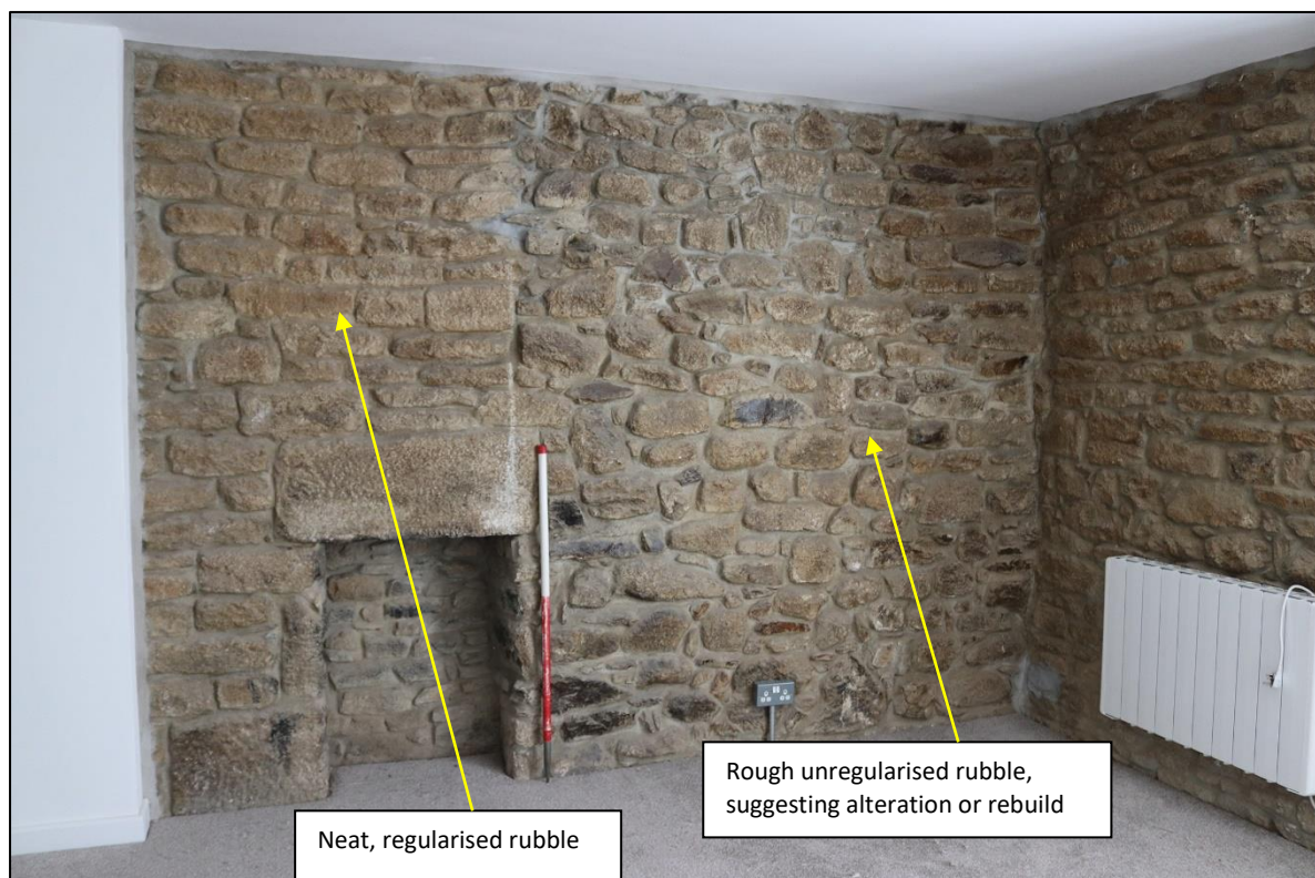
FIGURE 10: EXPOSED FIREPLACE TO FF FLAT TO EAST WITH AREA OF DISTURBANCE TO PARTY WALL, RELATED TO MASONRY ON GF. TAKEN FROM THE WEST WITH 1M SCALE.
