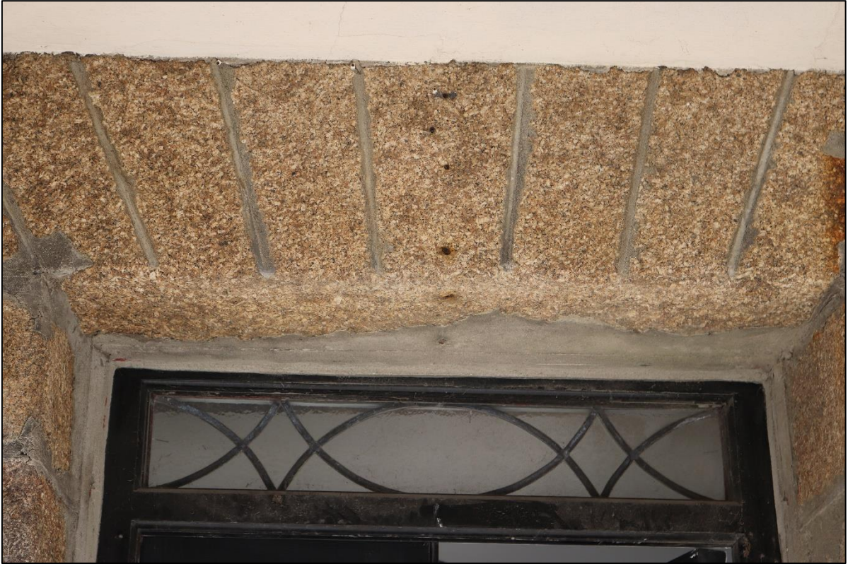
27. LINTEL DETAIL TO THE EXTERNAL FACE OF CENTRAL DOORWAY WITH SIGNIFICANT CEMENT REPAIR.
