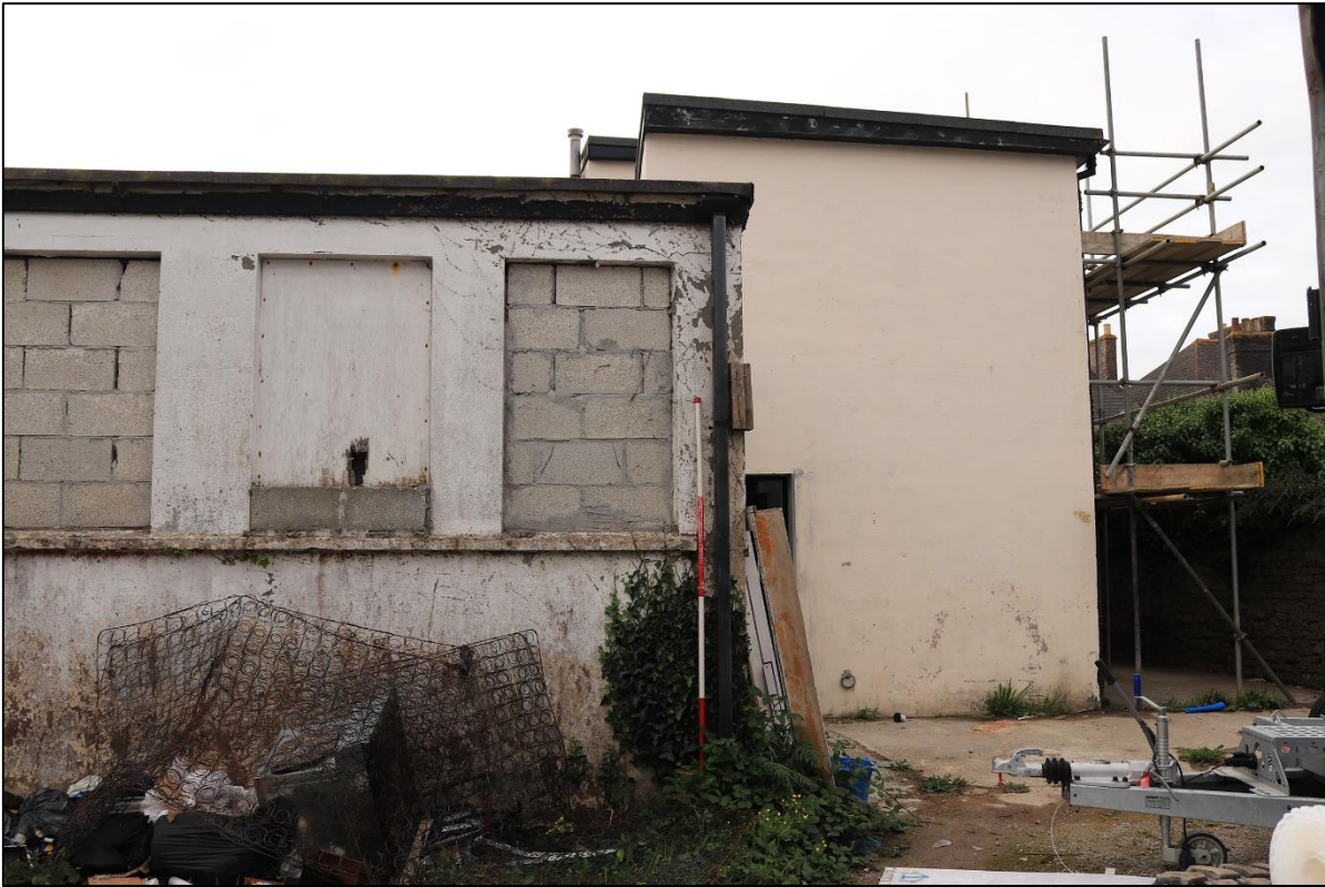
5. RELATIONSHIP BETWEEN 20 TH CENTURY STORAGE AND REAR OF 19 TH C BLOCK EXTENSION. TAKEN FROM THE NORTH WITH 2M SCALES.
