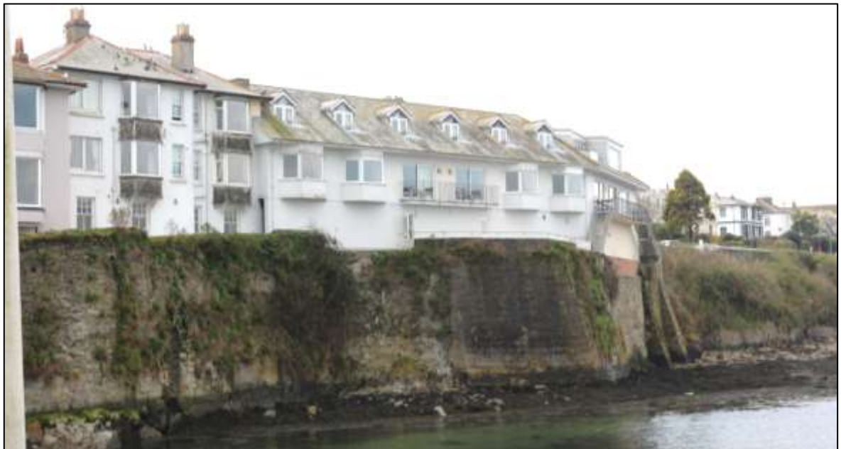
FIGURE 29: THE TALL RETAINING WALL BENEATH THE HOTEL, VIEWED FROM THE QUAY. VIEWED FROM THE ESE.
