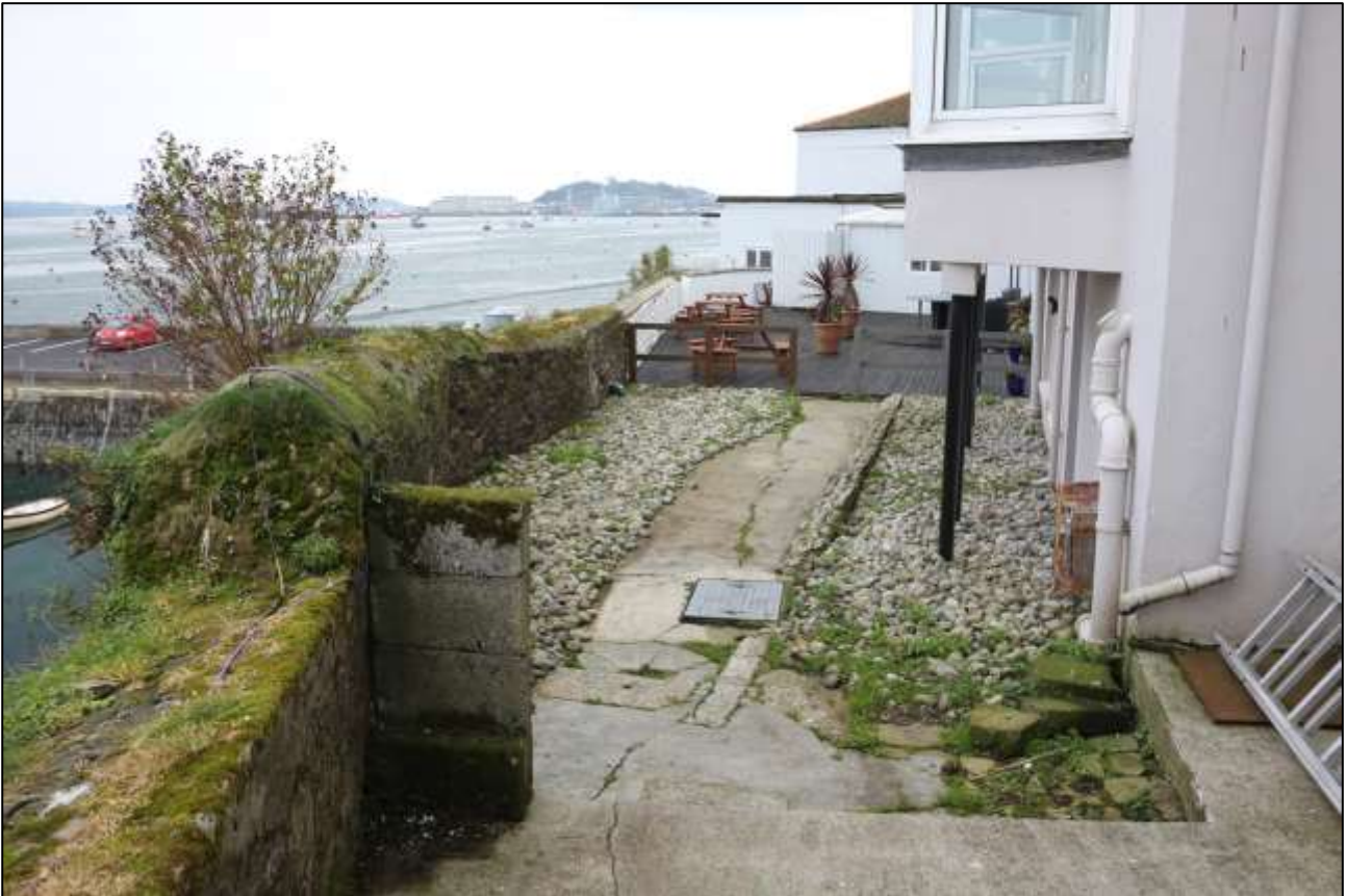
6. AREA 3, THE CENTRAL TERRACE, SURFACE TREATMENTS AND WALL; VIEWED FROM THE NNW.
