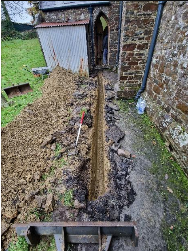
FIGURE 3: FIRST PHASE OF TRENCHING FROM THE VESTRY, VIEWED FROM THE WEST (SCALE 1M).
