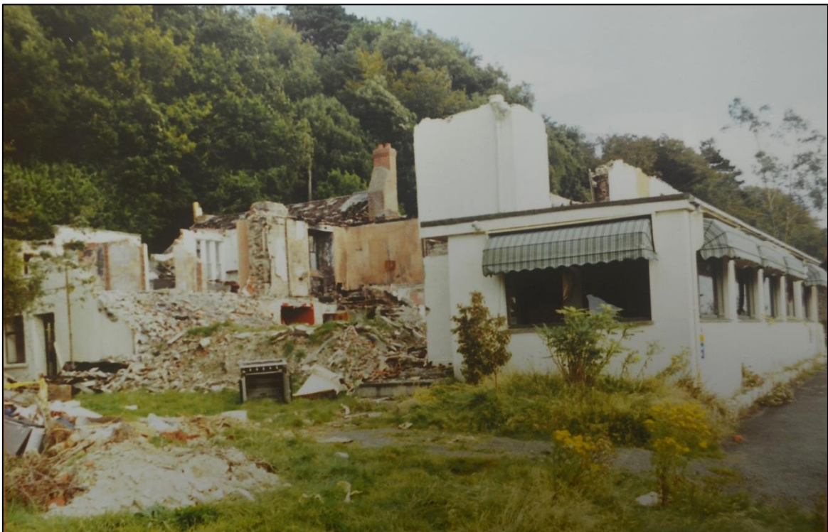
FIGURE 6: VIEW FROM THE SOUTH WEST OF THE HOTEL FOLLOWING THE FIRE IN THE 1990s (NDRO B513-1/126/1-5)
