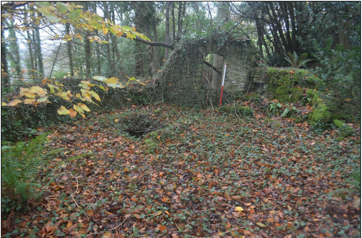
FIGURE 36: SUMMERHOUSE TERRACE VIEWED FROM THE SUMMERHOUSE LOCATION. COLLAPSED BRICK VAULTED ROOF OF GROUND FLOOR LEVEL VISIBLE (FROM THE EAST 1M SCALE).
