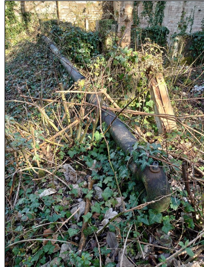
FIGURE 36: EXAMPLE OF A CAST-IRON PIPE FROM THE HEATED GLASSHOUSES.
