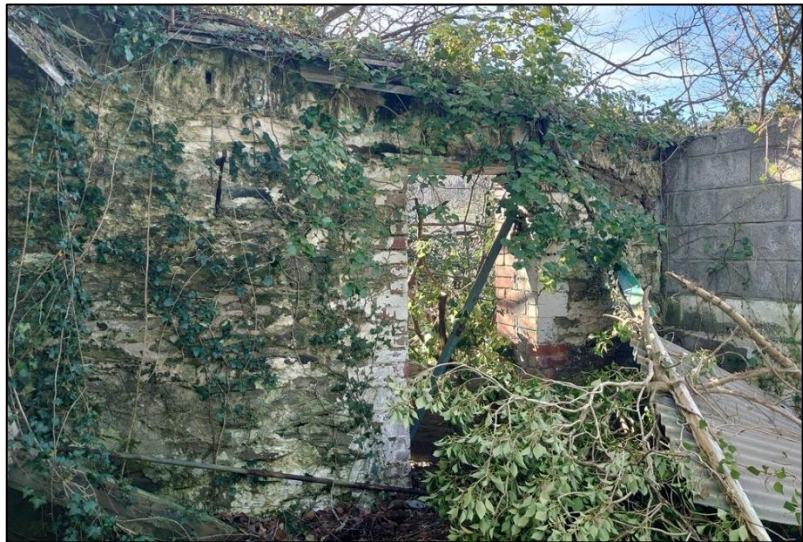
FIGURE 32: THE FORCED DOORWAY IN THE SOUTH GARDEN WALL; FROM THE NORTH-EAST.
