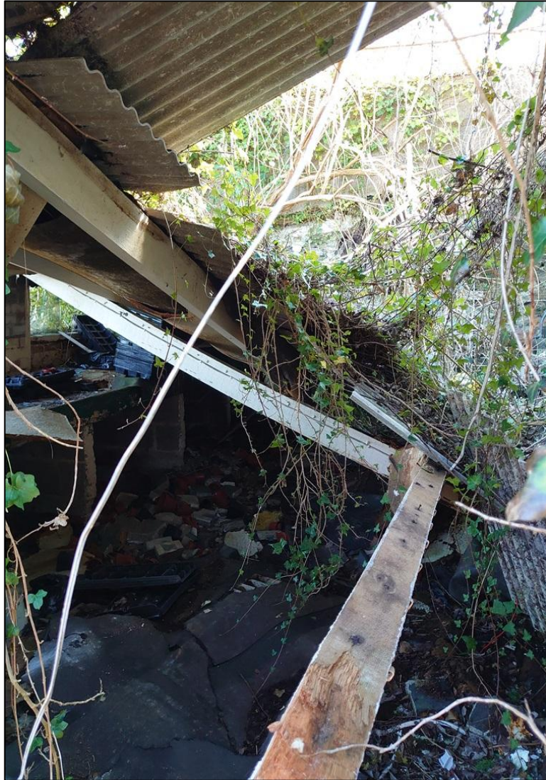
FIGURE 24: THE INTERIOR OF COLLAPSED BUILDING 4; FROM THE WEST.
