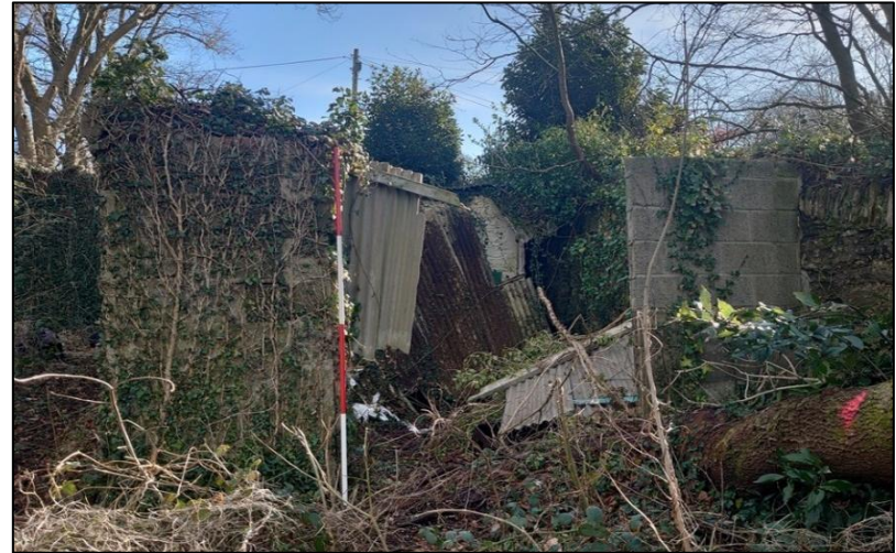
FIGURE 18: B3A, CONCRETE EXTENSION, WITH COLLAPSED ROOF (2M SCALE); FROM THE WEST.
