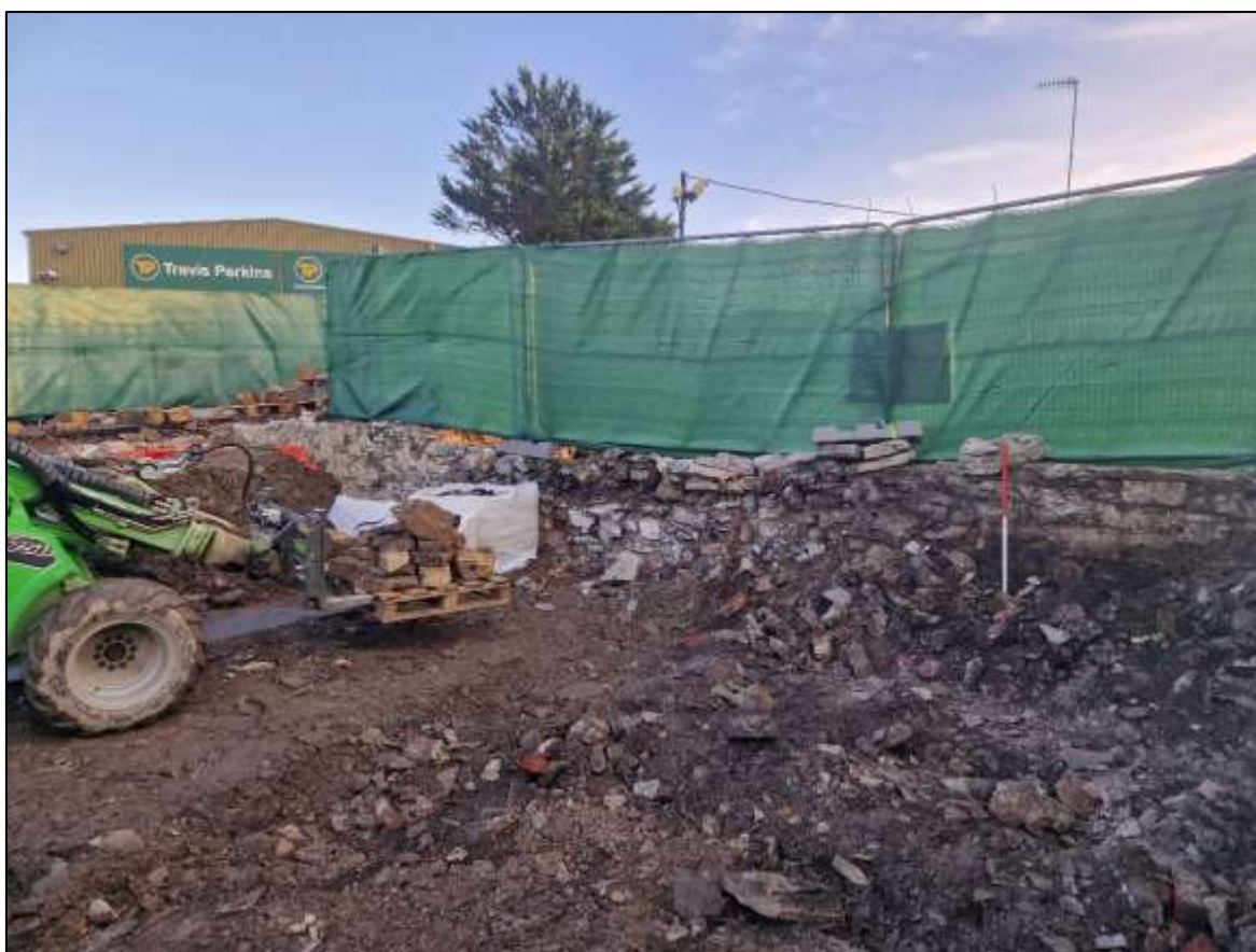
FIGURE 4: SITE DURING WORKS, MASONRY VISIBLE ON PALLET, WITH MASONRY WALL FORMING THE SITE BOUNDARY, VIEWED FROM THE NORTH-WEST (1M SCALE).
