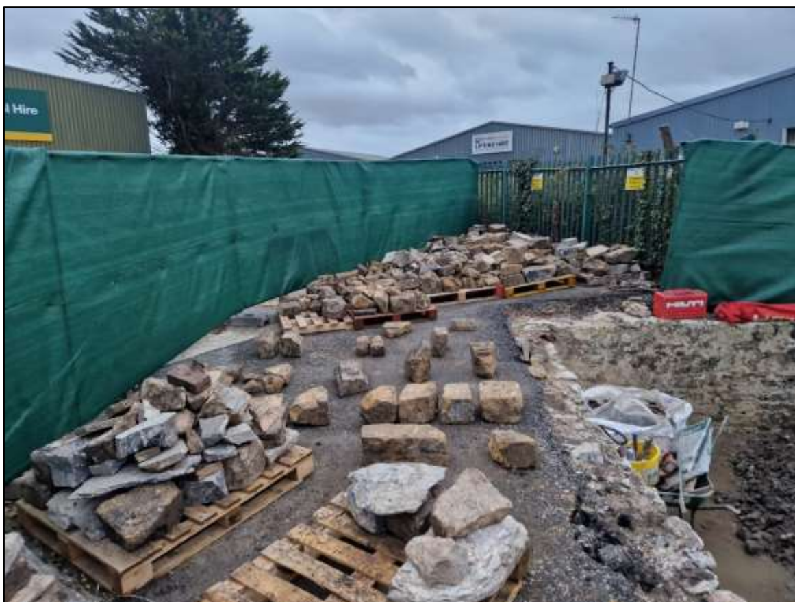
FIGURE 5: SITE DURING WORKS, THE MAJORITY OF THE RECOVERED MASONRY VISIBLE ON PALLETS IN SHOT, THE MASONRY WALLS FORMING THE DEMOLISHED BUILDING ARE TO THE LEFT OF SHOT, VIEWED FROM THE NORTH-WEST (NO SCALE).
