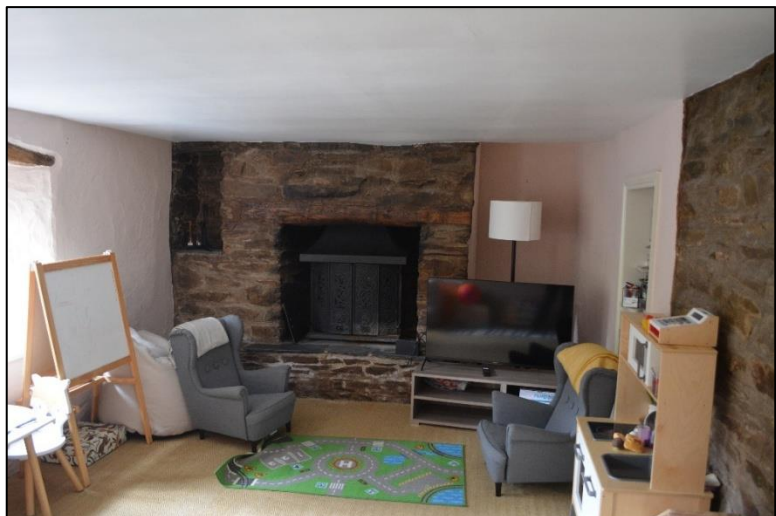
6. MAIN HOUSE PLAYROOM REPRESENTING THE OLDEST PART OF THE STRUCTURE, WITH BLOCKED DOORWAY, FIREPLACE AND THICK STONE WALLS.
