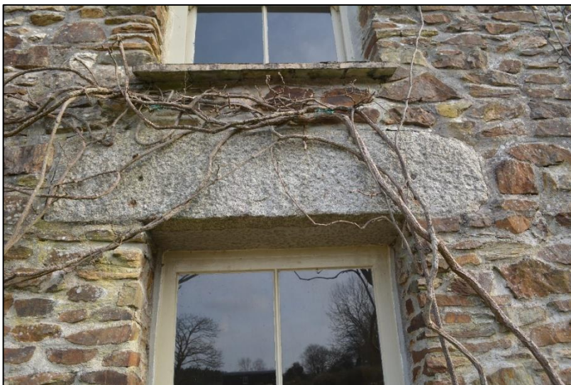
17. GRANITE LINTEL IN WEST ELEVATION WITH HOLES INDICATING REUSE IN THIS LOCATION
