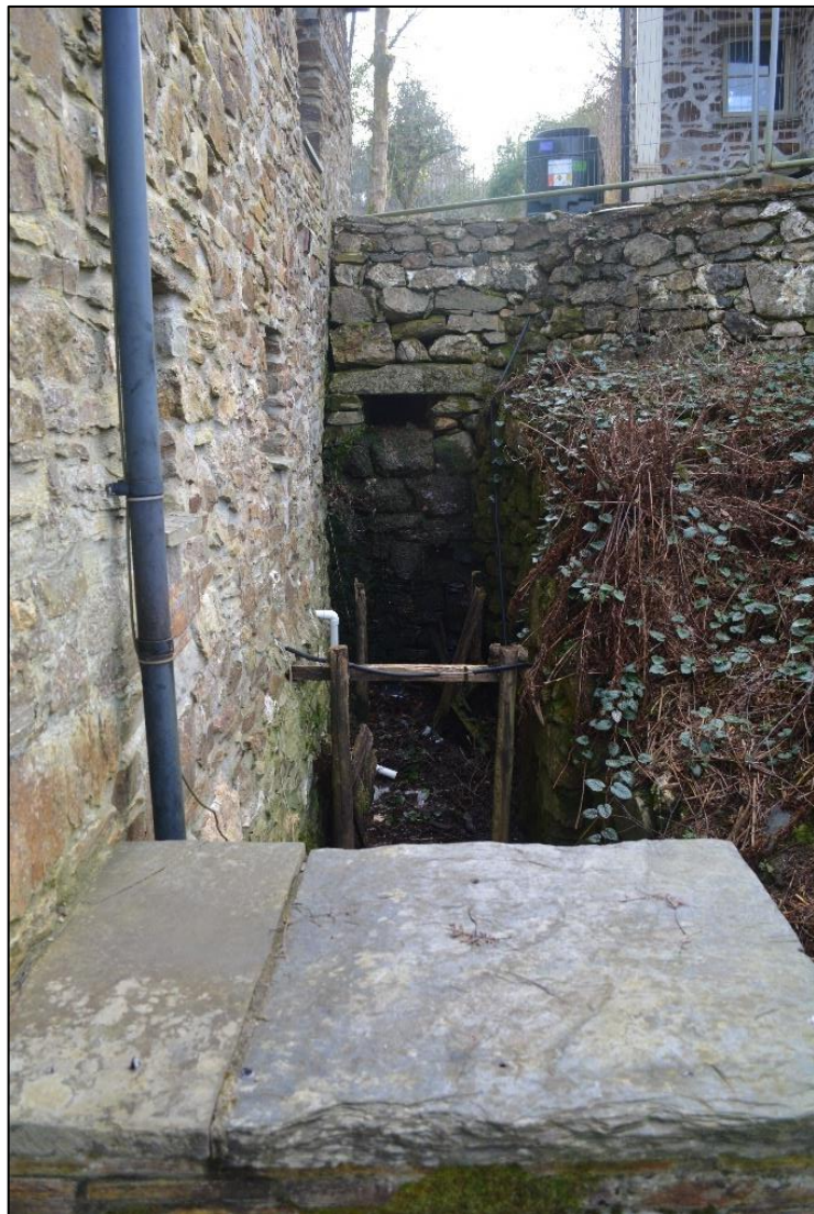
29. WHEEL PIT TO WESTERN SIDE OF MILL SHOWING LEAT FOR OVERSHOT WHEEL WITH FRAGMENTARY REMAINS OF WHEEL.
