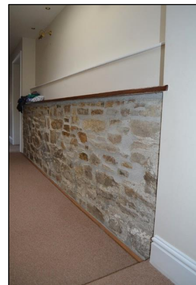
12. MAIN HOUSE SHOWING NORTHERN WALL OF SNUG AT FIRST FLOOR LEVEL INDICATING A NUMBER OF RAISES TO THIS SECTION OF THE PROPERTY. SOME WHITEWASH IS VISIBLE ON THE LOWER STONES OF THE EXPOSED WALL. FROM THE WEST.
