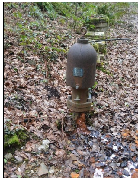
41. HISTORIC HYDRAULIC RAM LOCATED NEAR STREAM TO NORTH OF HOUSE, NOW REPLACED.
