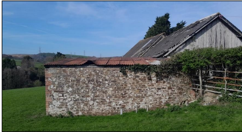
FIGURE 12: B3, THE LONG EAST WALL, SHOWING BRICK QUINS AND CORRUGATED TIN SHEETING FOR ROOF; FROM THE EAST.
