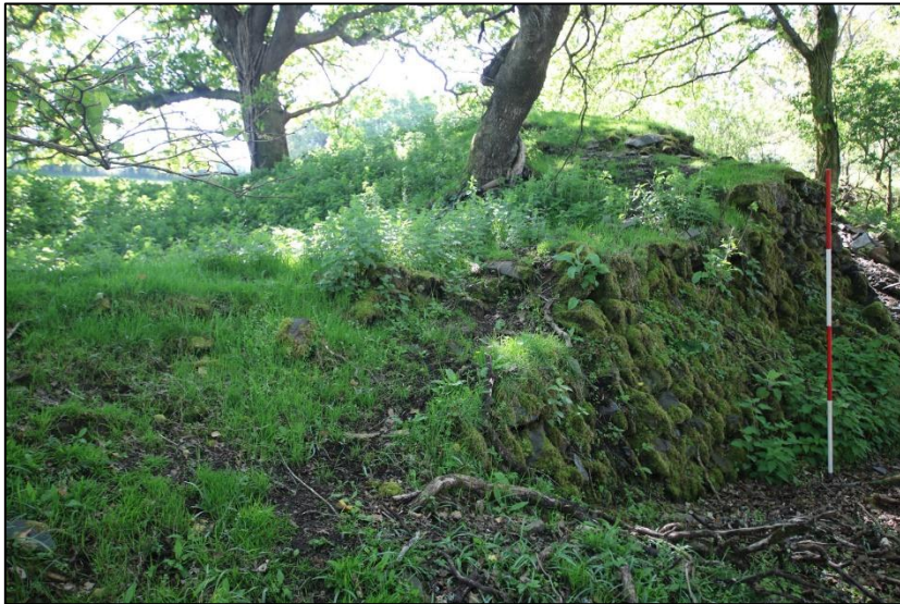
FIGURE 55: THE RETAINING WALL BELOW THE CRUSHER HOUSE; FROM THE NORTH-EAST (SCALE 2M).
