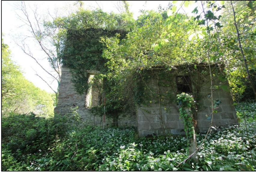
FIGURE 17: THE NORTH-WEST ELEVATION; FROM THE NORTH-WEST (SCALE 2M). THE BUILDING IN THE FOREGROUND IS THE C20 PUMP HOUSE.
