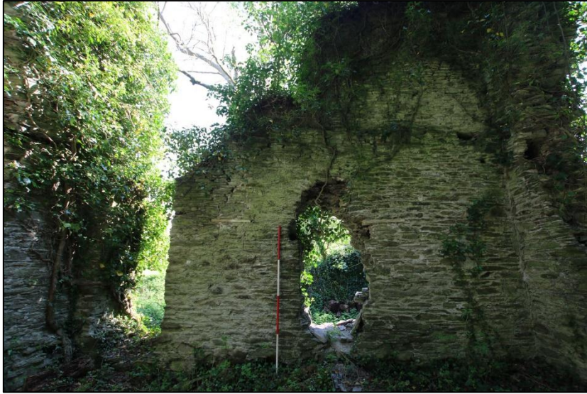
FIGURE 19: THE INTERNAL ELEVATION OF THE SOUTH-EAST WALL; FROM THE NORTH-WEST (SCALE 2M).
