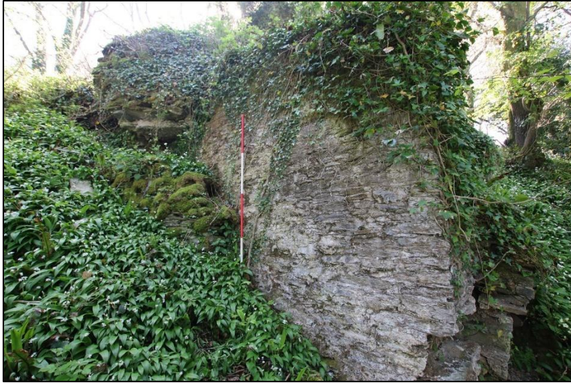
FIGURE 30: THE SIDE OF THE EASTERN BALANCE BOB PIT WALL; FROM THE NORTH (SCALE 2M).
