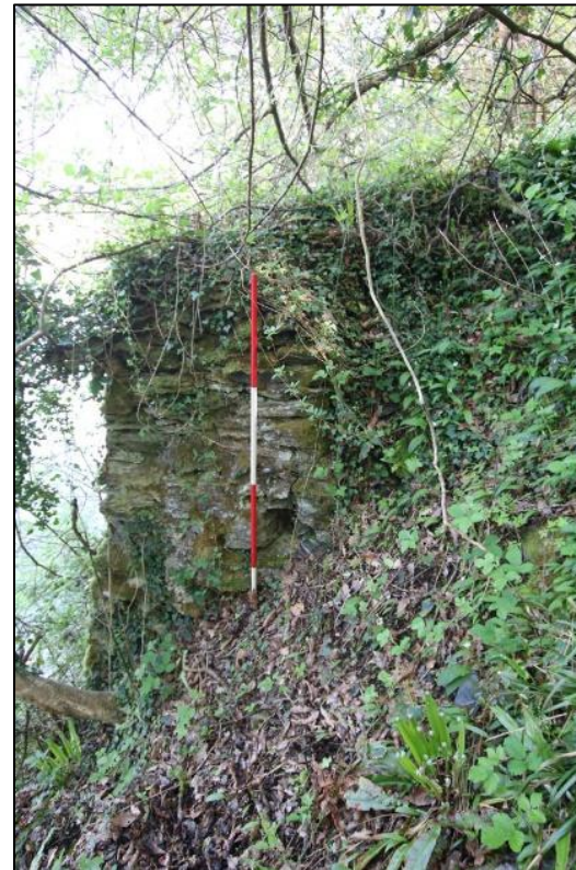
FIGURE 71: DETAIL OF THE SW CORNER OF THE STRUCTURE; FROM THE SOUTH (SCALE 2M).
