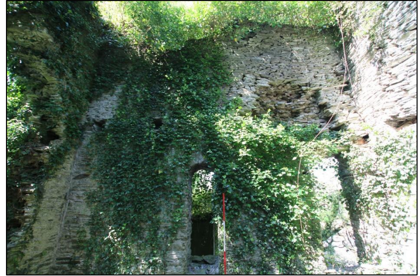
FIGURE 21: THE INTERNAL ELEVATION OF THE NORTH-WEST WALL; FROM THE SOUTH-EAST (SCALE 2M).
