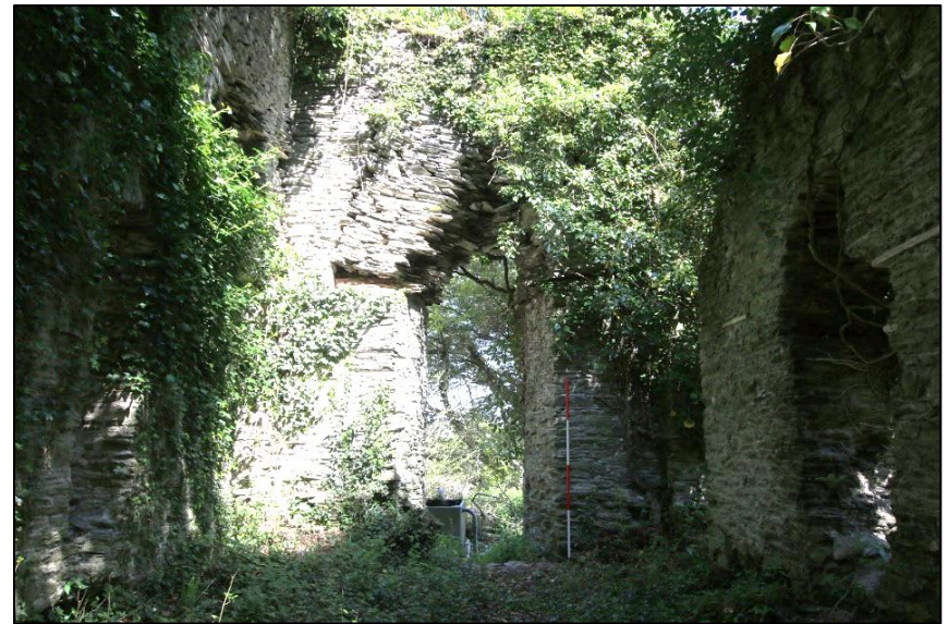
FIGURE 18: THE INTERNAL ELEVATION OF THE NORTH-EAST WALL; FROM THE SOUTH-WEST (SCALE 2M).
