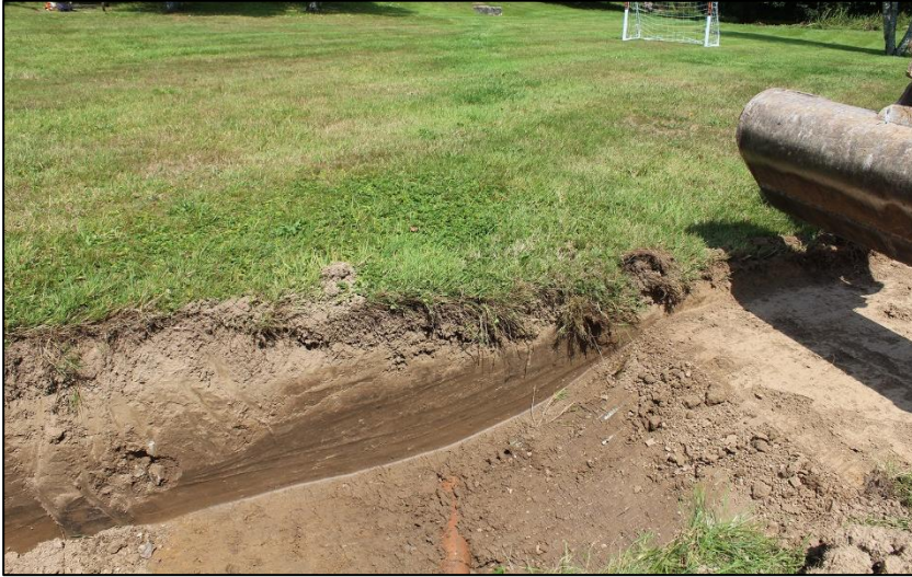
17. CLAY LAND DRAIN AT EAST END OF TRENCH #3; VIEWED FROM THE WEST-SOUTH-WEST.
