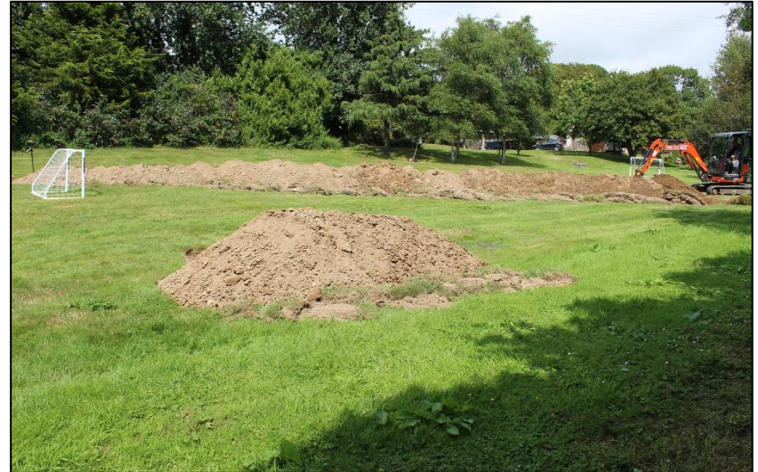
16. VIEW ACROSS TRENCH #2 ON LINE OF DRAINS; VIEWED FROM THE SOUTH-WEST (NO SCALE).
