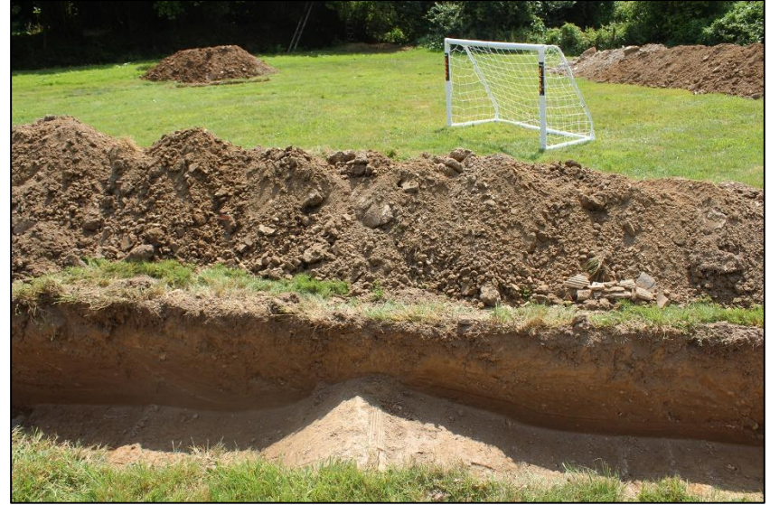
23. LINE OF TILE DRAIN IN TRENCH #3; VIEWED FROM THE NORTH-EAST (NO SCALE).
