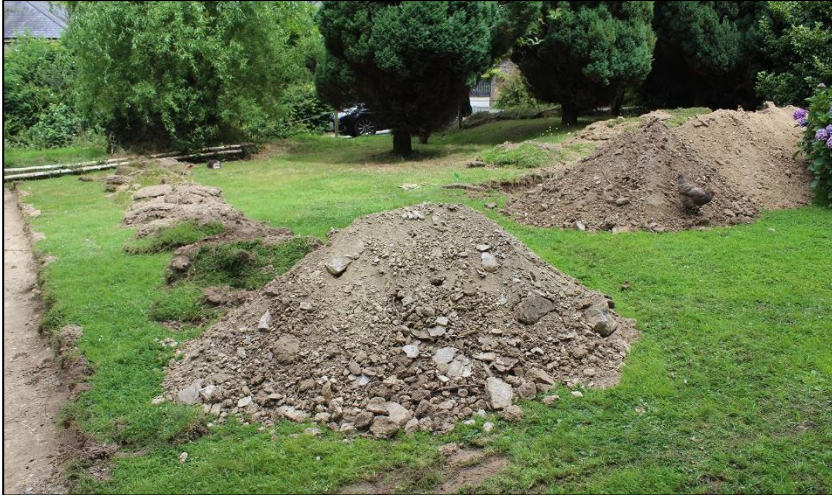
69. NORTHERN AREA FROM THE SOUTH-EAST END OF TRENCH #7; FROM THE SOUTH (NO SCALE).
