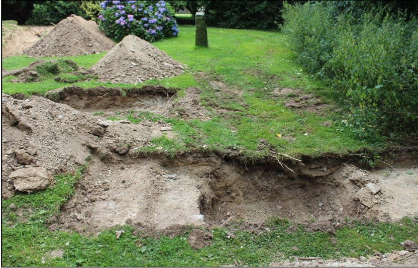
45. LINE OF SOUTH EDGE OF SLAB, TRENCH #6; VIEWED FROM THE SOUTH-WEST (NO SCALE).
