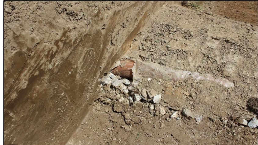
19. DETAIL OF PLASTIC PIPE IN TRENCH #3; VIEWED FROM THE WEST (NO SCALE).
