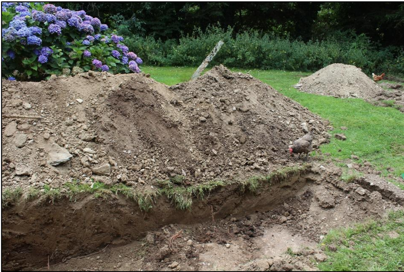
54. LINE OF STEP IN SLAB TOWARDS GRANITE POST; VIEWED FROM THE NORTH (NO SCALE).
