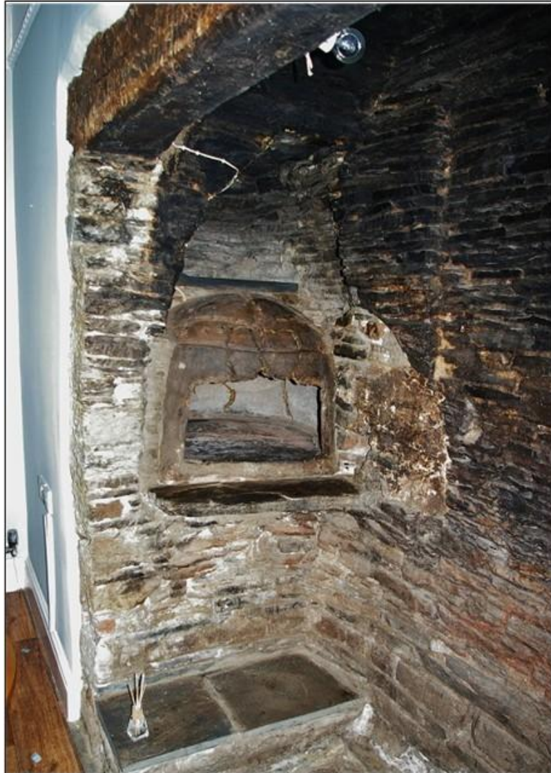
FIGURE 24: THE VICTORIAN CLOAM OVEN THAT HAS BEEN FORCED INTO THE SIDE OF THE 17 TH CENTURY STACK, REPLACING AN EARLIER OVEN; FROM THE NORTH-NORTH-EAST.
