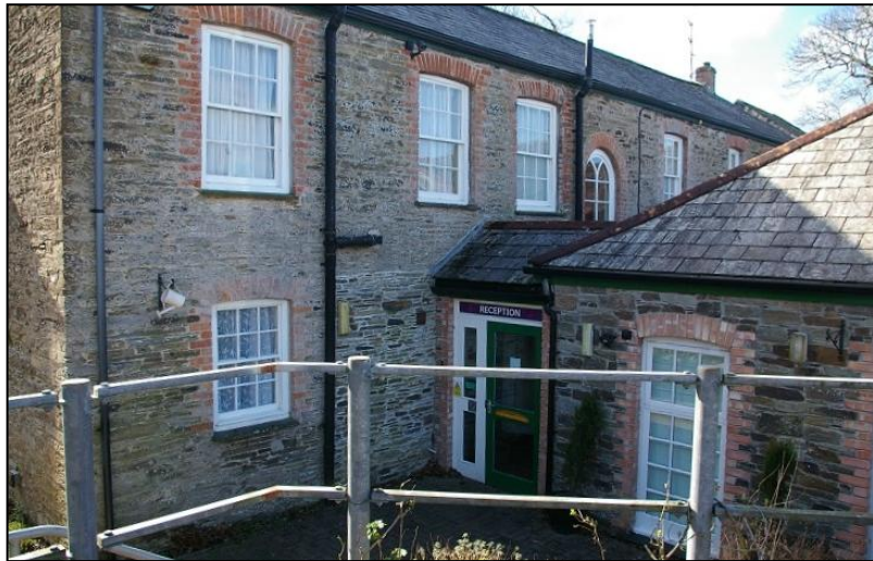
FIGURE 13: THE REAR ELEVATION OF THE PARALLEL RANGE, ABUTTED BY A NUMBER OF EXTENSIONS; FROM THE NORTH-EAST.
