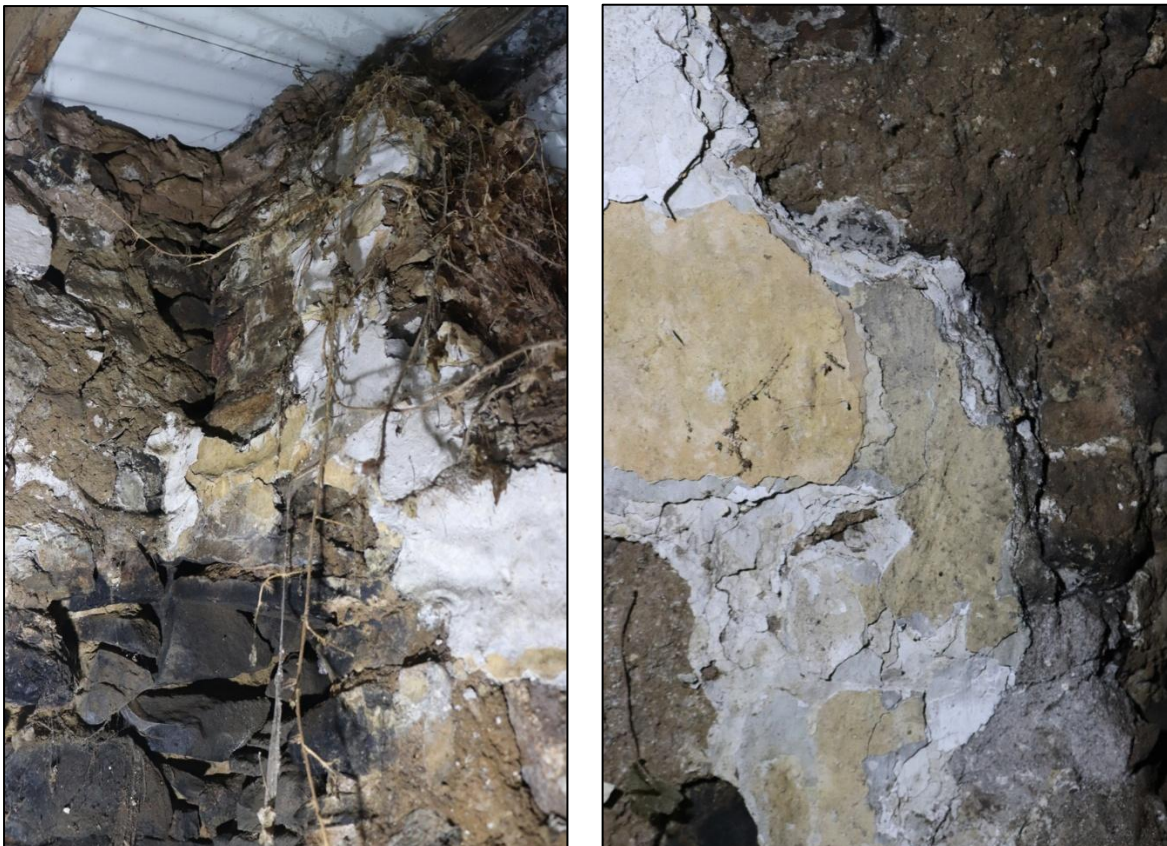
FIGURE 17: LEFT – STACK ADDED AGAINST THE SOUTHERN ELEVATION, VERY POORLY TIED. RIGHT- LAYERS OF LIMEWASH OVER EARTH PLASTER, WHICH INDICATES MORE VERNACULAR ORIGINS AND THE VALUE OF MAINTENANCE EVEN TO A SECONDARY SPACE.
