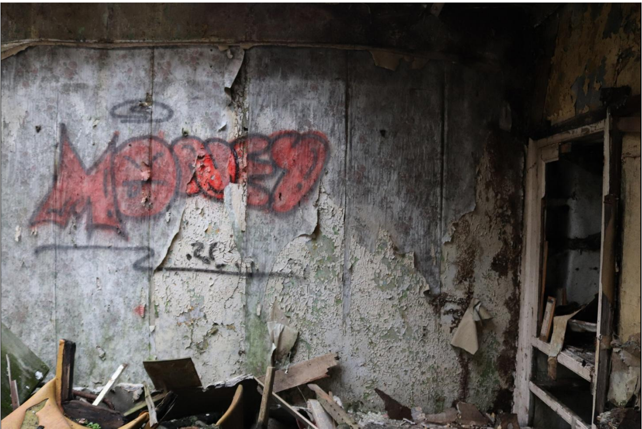
29. THE WEST ELEVATION OF R4 SHOWING LOST DECORATIVE SCHEMES, FROM THE EAST.
