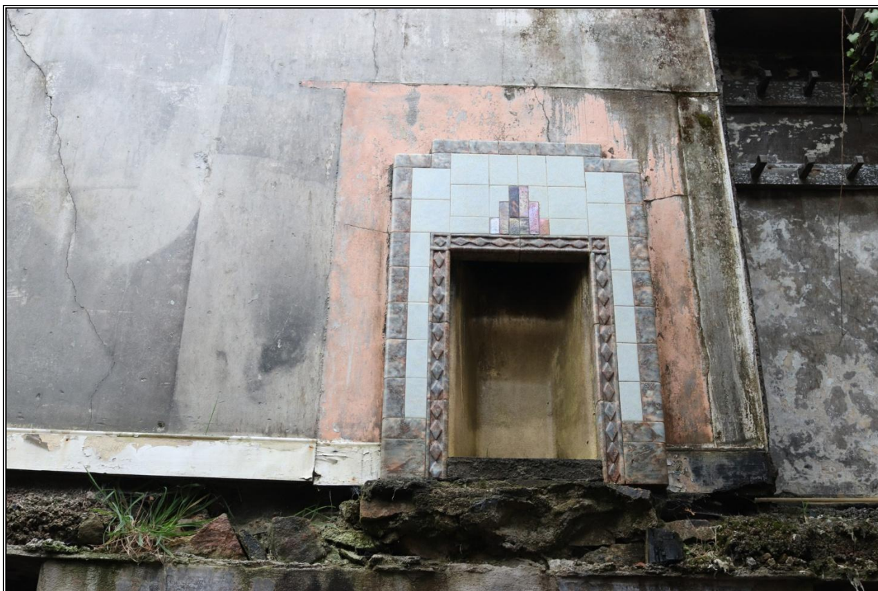
50. ALTERED FF FIREPLACE OVER R2.
