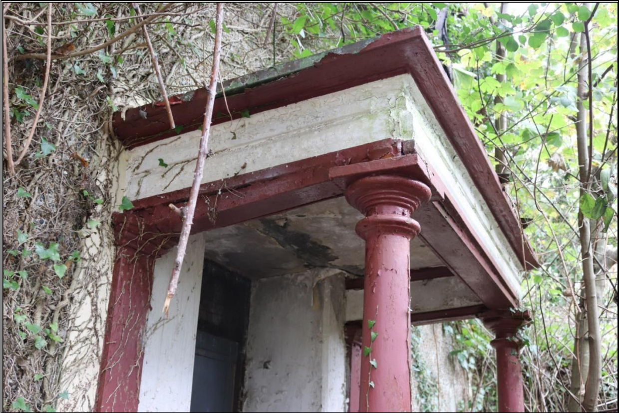
15. CANOPY OVER PORCH, AD HOC CAST IRON PADS BRACE BETWEEN COLUMN AND DETAILED HOOD.
