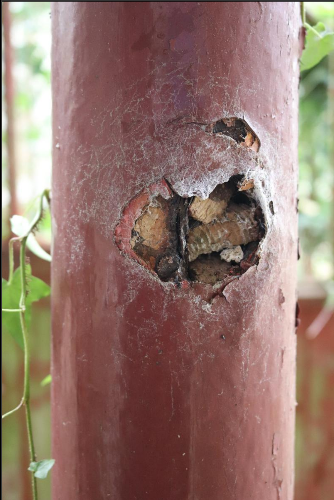
21. HOLES TO REAR OF EACH COLUMN SUGGESTING LOST RAILING, FURTHER INDICATION OF THE A RESET STRUCTURE.
