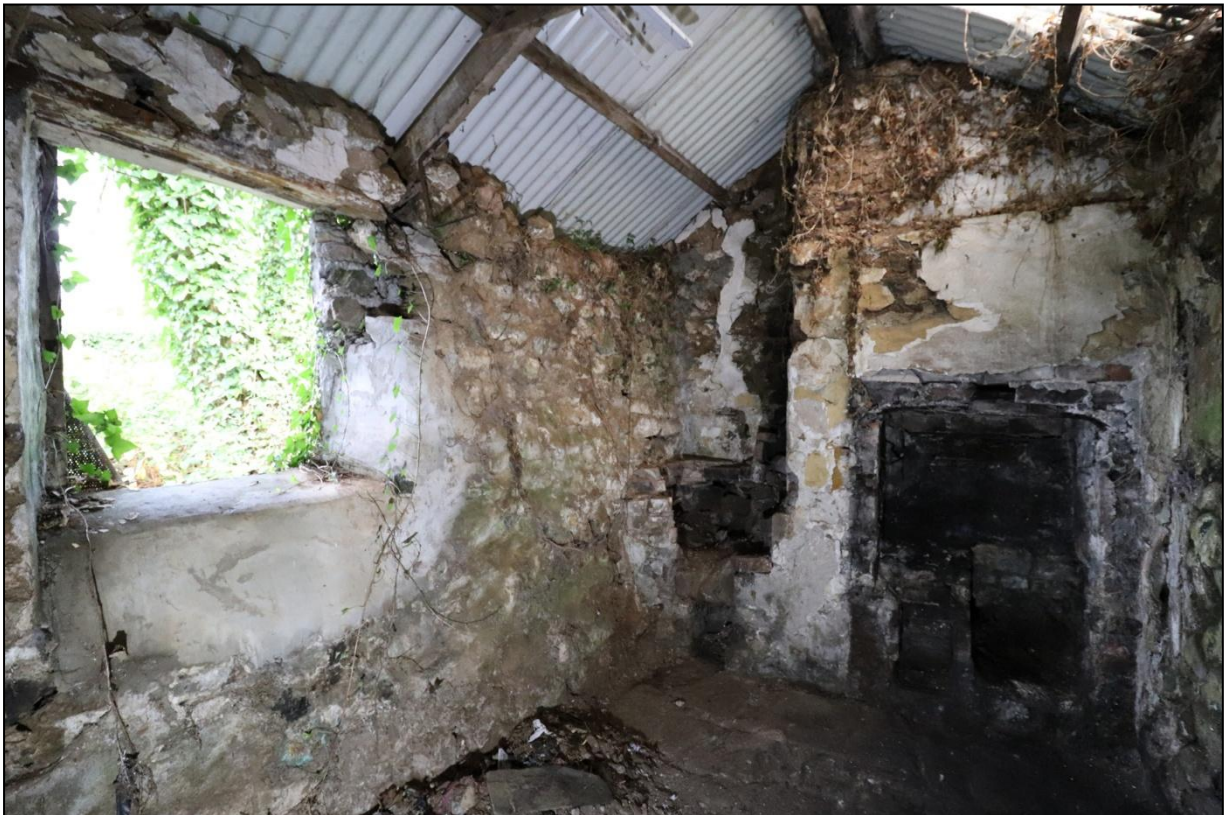
FIGURE 19: BATTERED EAST WALL, WITH FORCED AND ALTERED WINDOW TO THE EAST WALL, TAKEN WITH A WIDE-ANGLED LENS, FROM THE NORTH.
