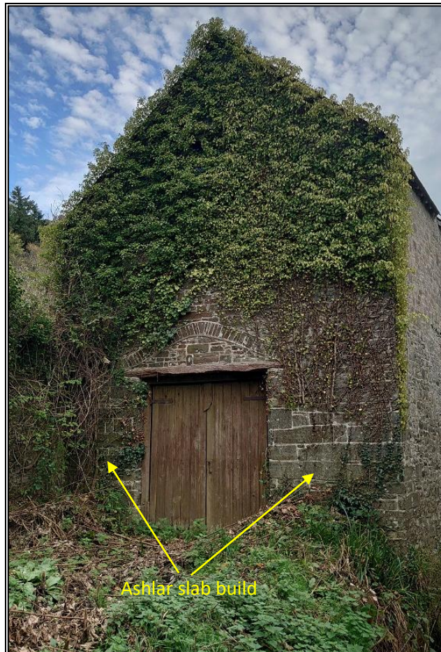
FIGURE 18: THE WEST WALL OF BUILDING 2, SHOWING DIFFERENCES IN BUILD, POSSIBLY USING RECYCLED ASHLAR AND LARGE DOUBLE DOORS TO THE INTERIOR, THE DATESTONE IS BELIEVED TO BE UNDER THE IVY; FROM THE WEST.
