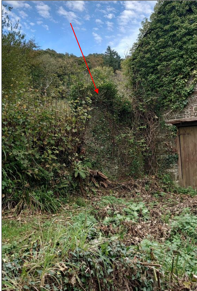
FIGURE 19: THE FRAGMENT OF BUILDING 3, ATTACHED TO THE END OF BUILDING 2; FROM THE SOUTH-WEST.
