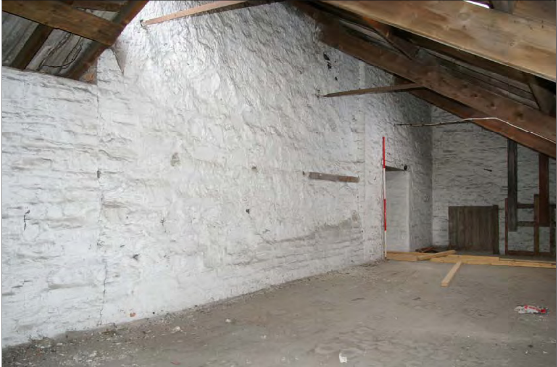
Figure 34: The south wall of Room 4, viewed from the north-east. The gable end of the Phase 2 building is clearly visible with its rough coating of render, abutted on both sides by later walls (scale 2m).
