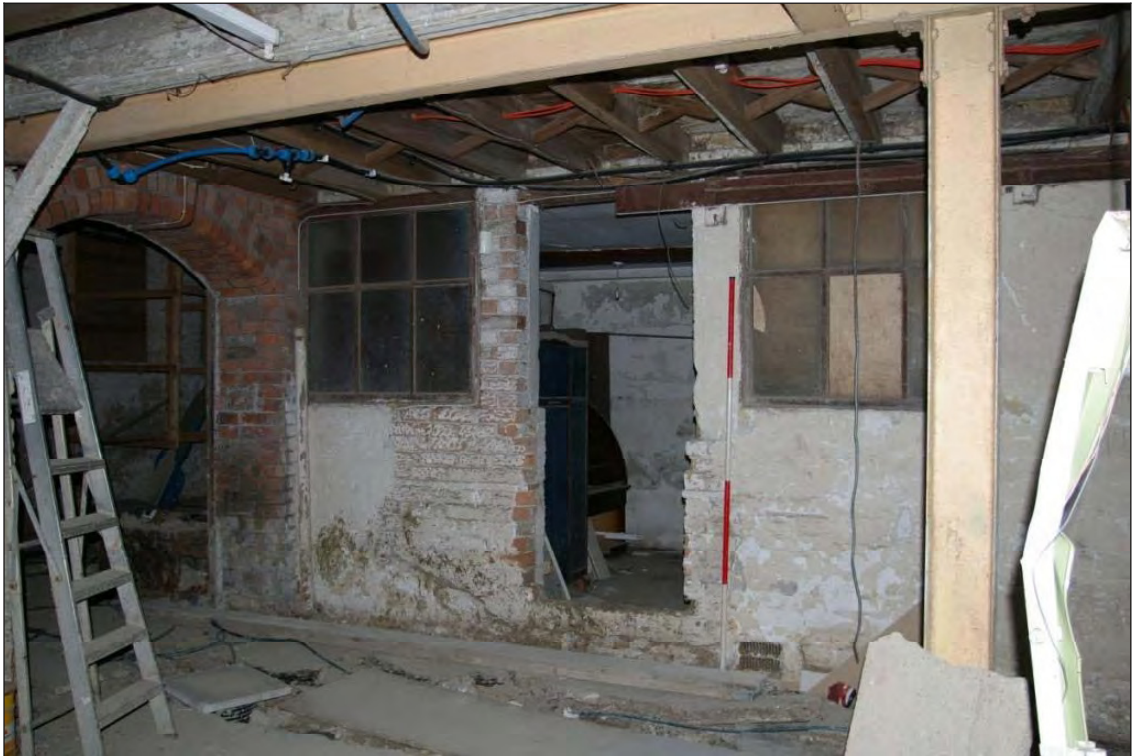
Figure 11: Door 5 viewed into Room 3a, viewed from Room 1 in the west (2m scale).
