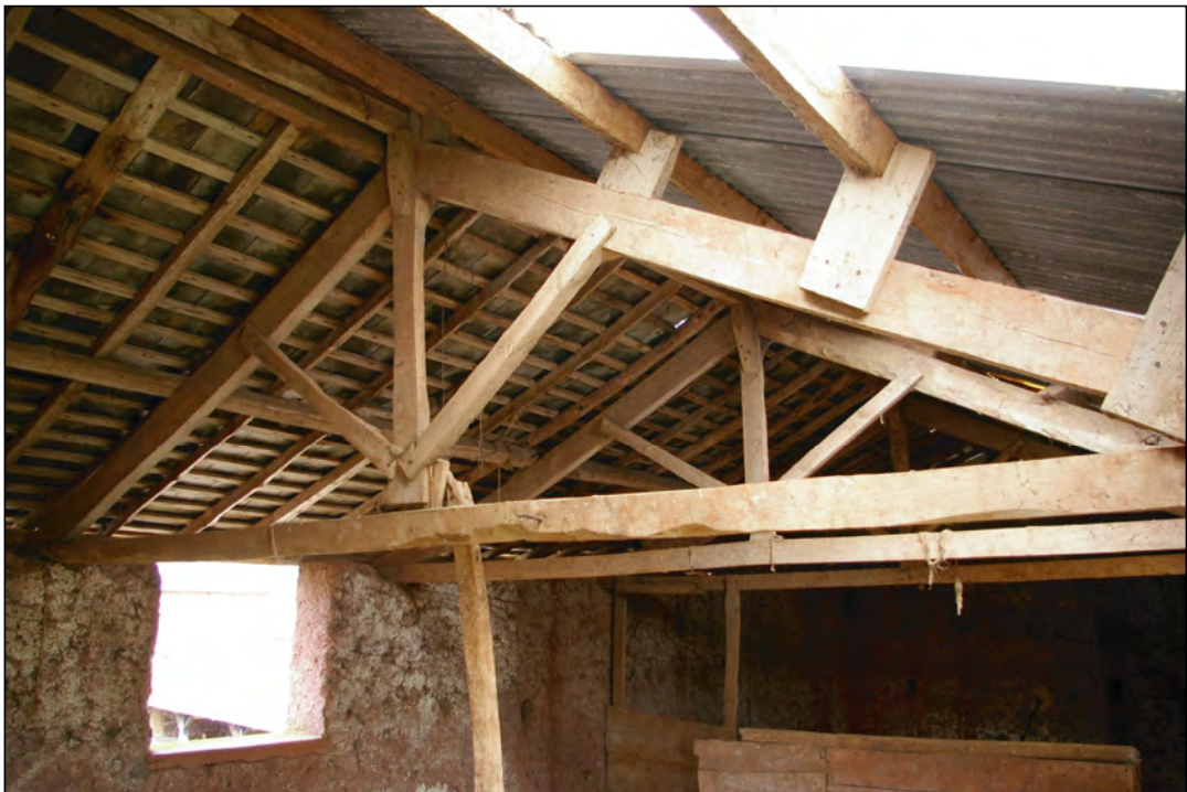
Plate 6: The roof structure of the Pound House, viewed from the south west.
