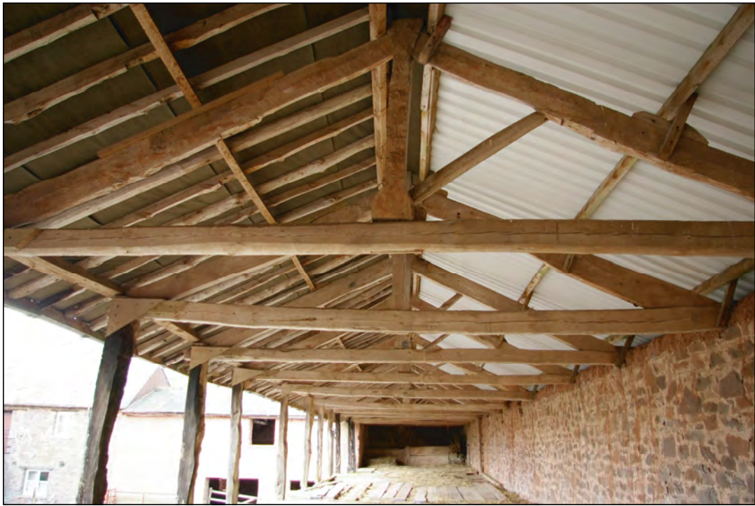
Plate 5: The first floor and roof structure of the Linhay, viewed from the north.
