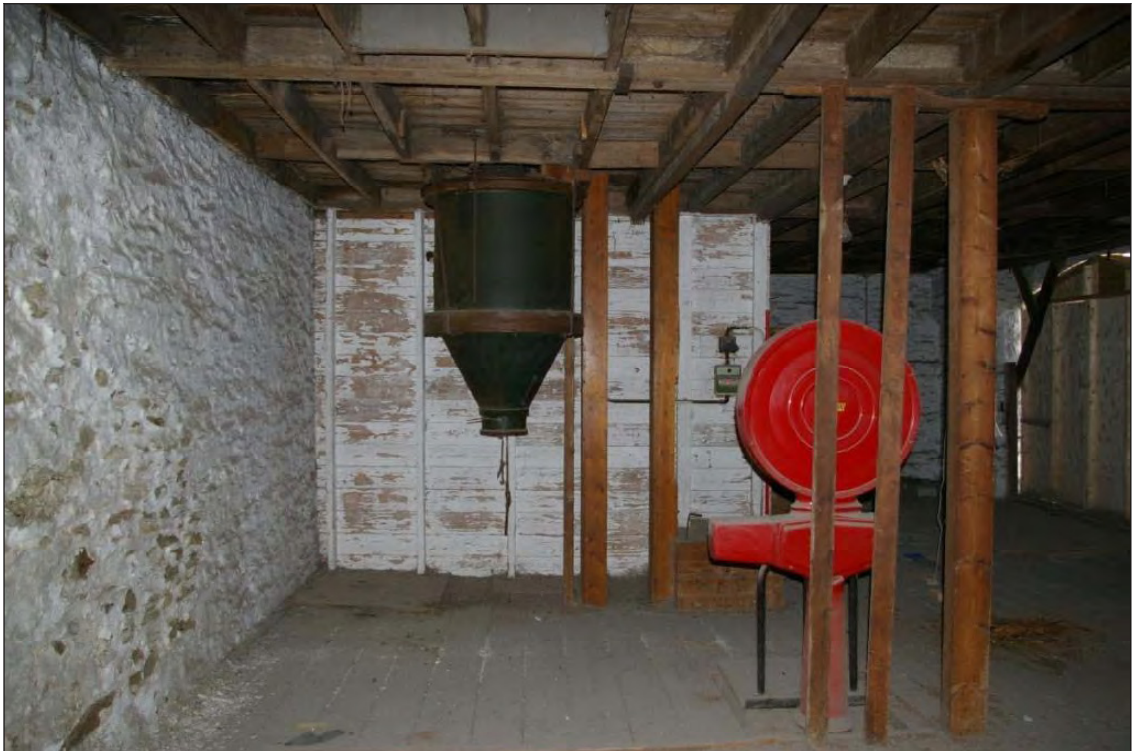
Figure 21: The grain hopper and scales in the south east corner of Room 13, viewed from the north.
