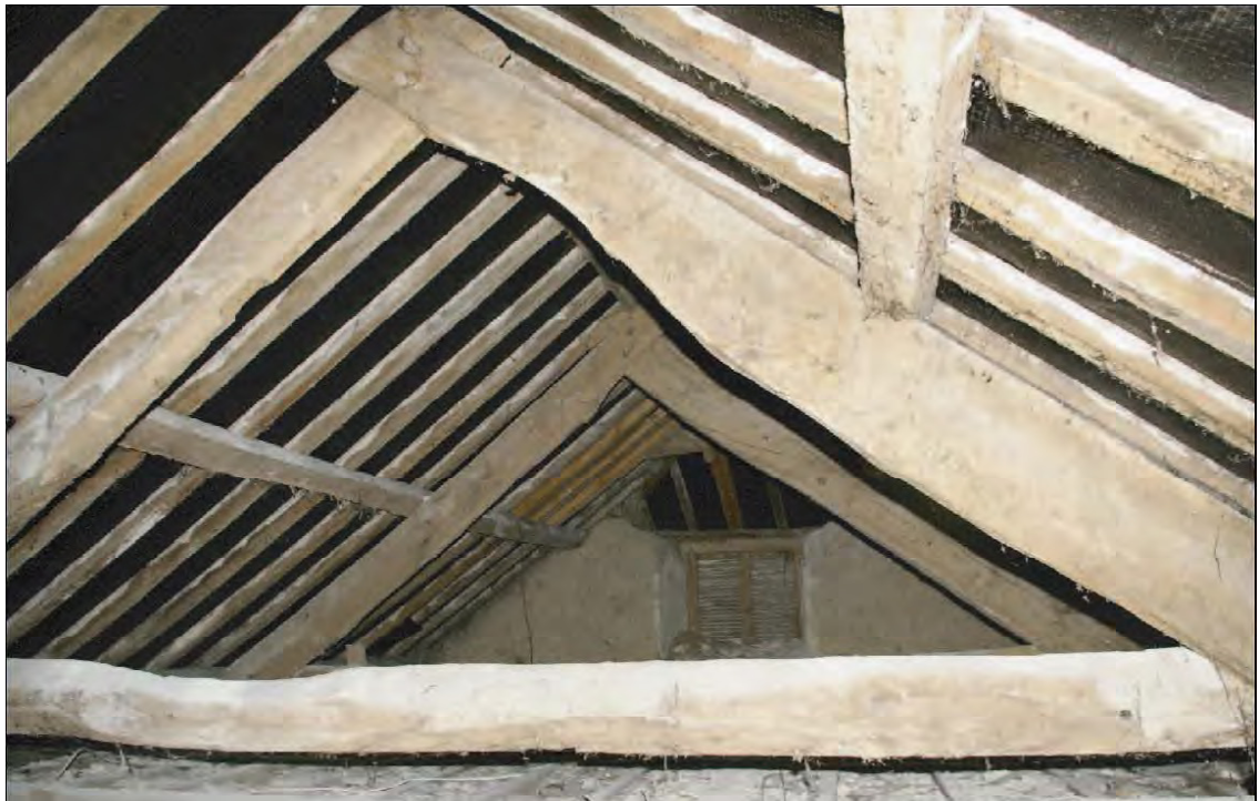
Figure 14: The roof structure over the main range, showing a blocked window in the north wall. Viewed from the south.
