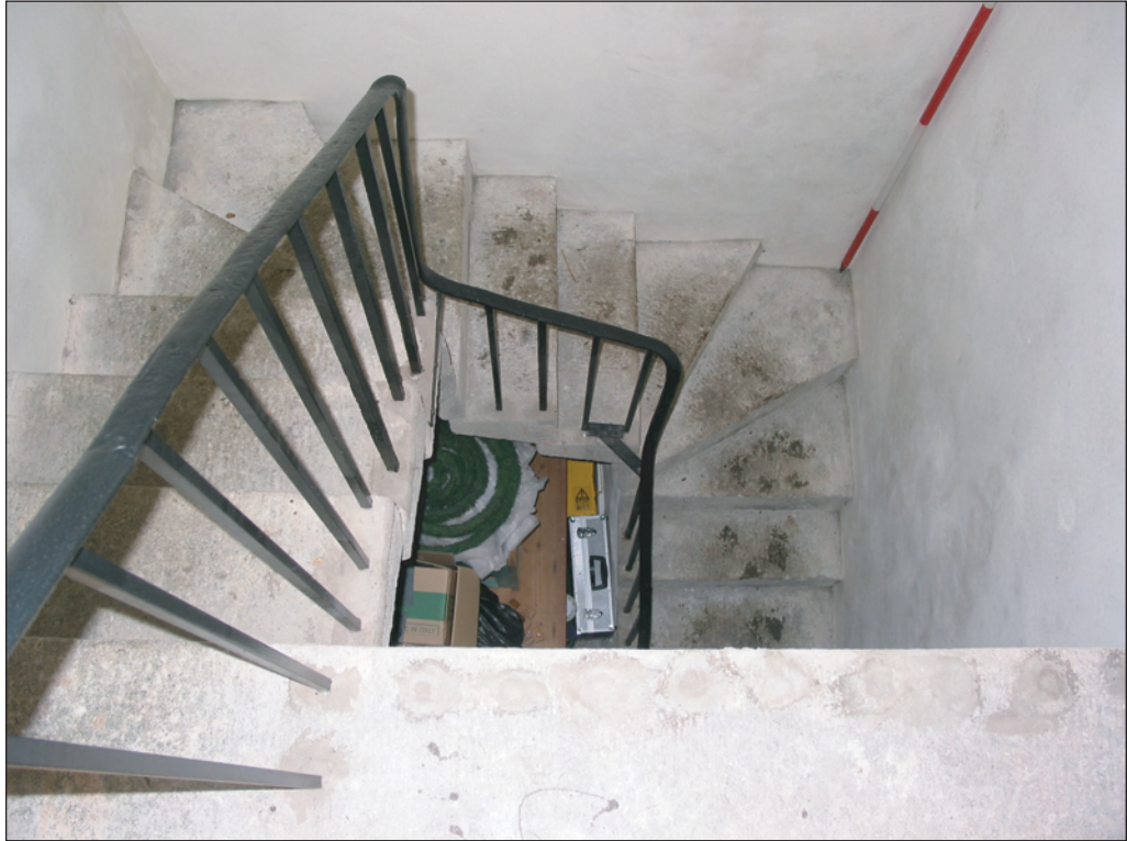
Plate 5: The stairs viewed from above. (Note the scars along the edge of the granite lintel).
