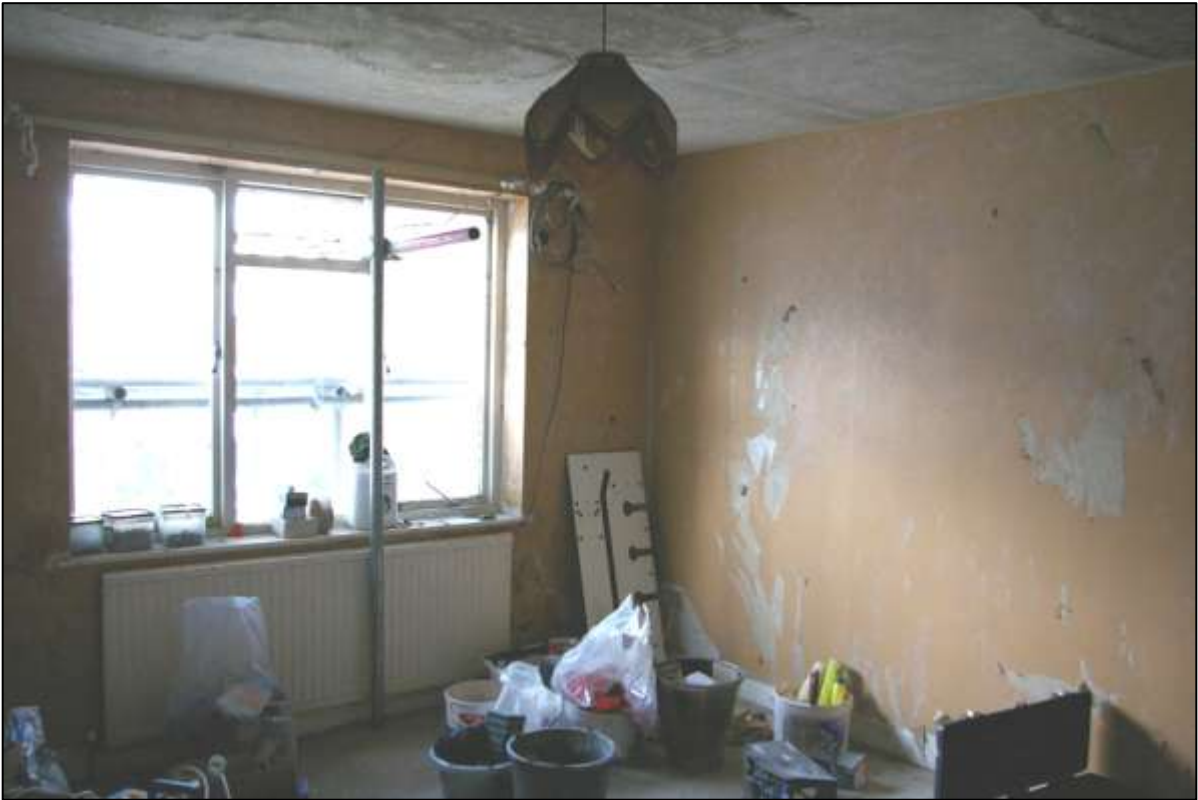
INTERNAL NORTH AND EAST WALLS OF FR4; VIEWED FROM THE SOUTH-WEST (NO SCALE).
