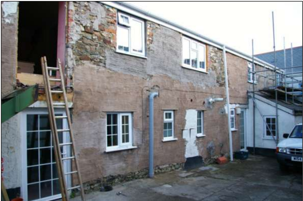
WEST ELEVATION OF EAST WING SHOWING BRICK REPAIRS AND RUBBLE STONE CONSTRUCTION BENEATH THE RENDER; VIEWED FROM THE NORTH-WEST.
