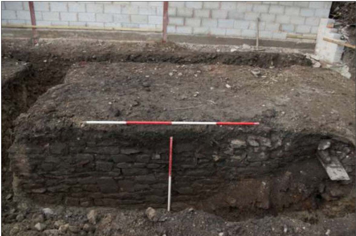
FIGURE 17: STONE WALL {018}, SOUTH FACING ELEVATION WITH KEYED WALL {019}; VIEWED FROM THE SOUTH (1M & 2M SCALES).
