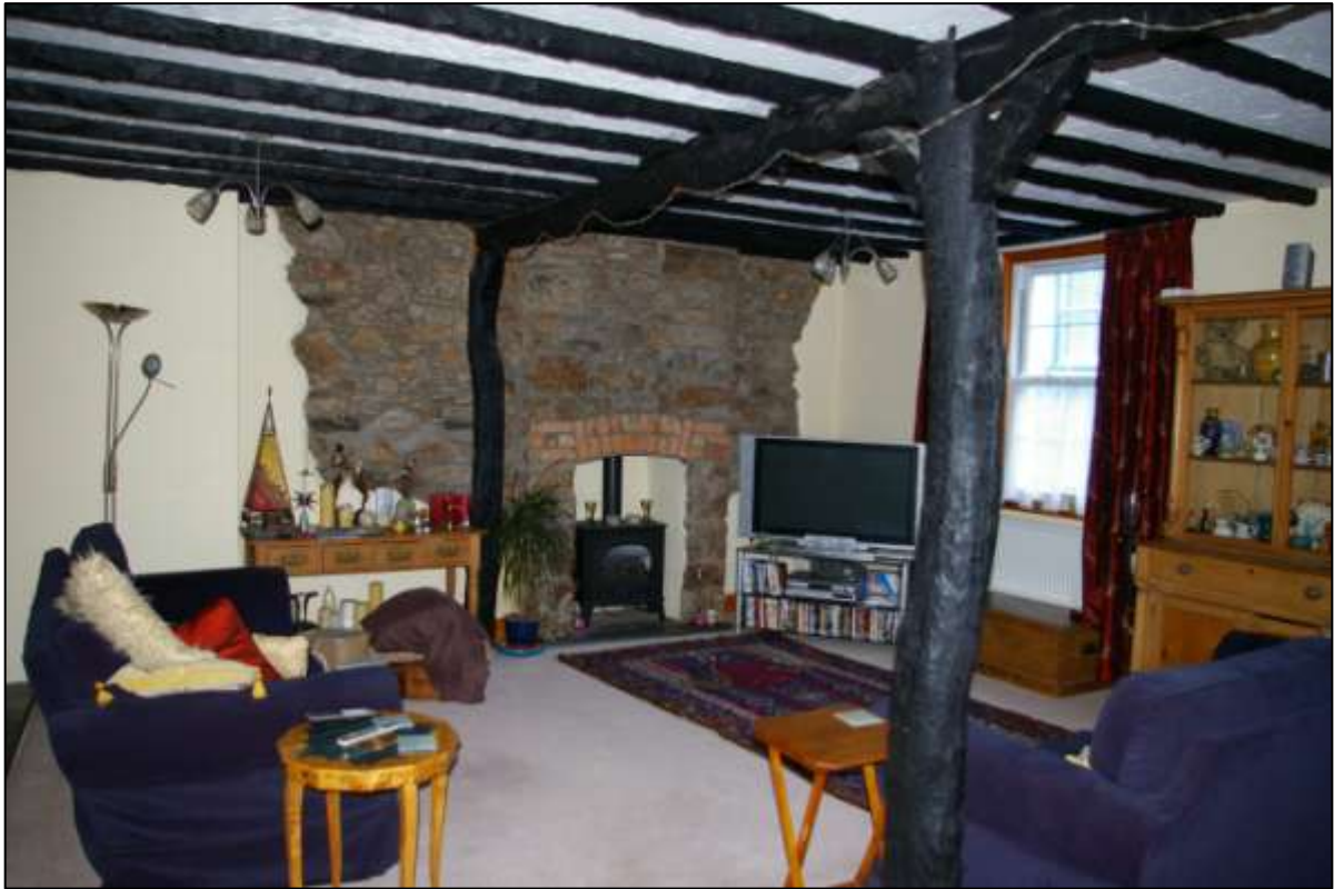
INTERNAL EAST WALL OF GR4 SHOWING TIMBER SUPPORTS; VIEWED FROM THE NORTH-WEST (NO SCALE).
