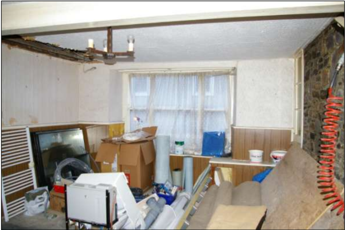
INTERNAL SOUTH WALL OF GR1 SHOWING SASH WINDOW; VIEWED FROM THE NORTH-WEST (NO SCALE).
