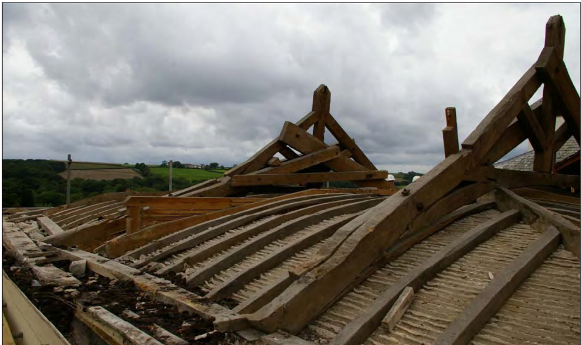
Figure 10: The ceiling and roof structure above Rooms 4 and 5, viewed from the south-west.
