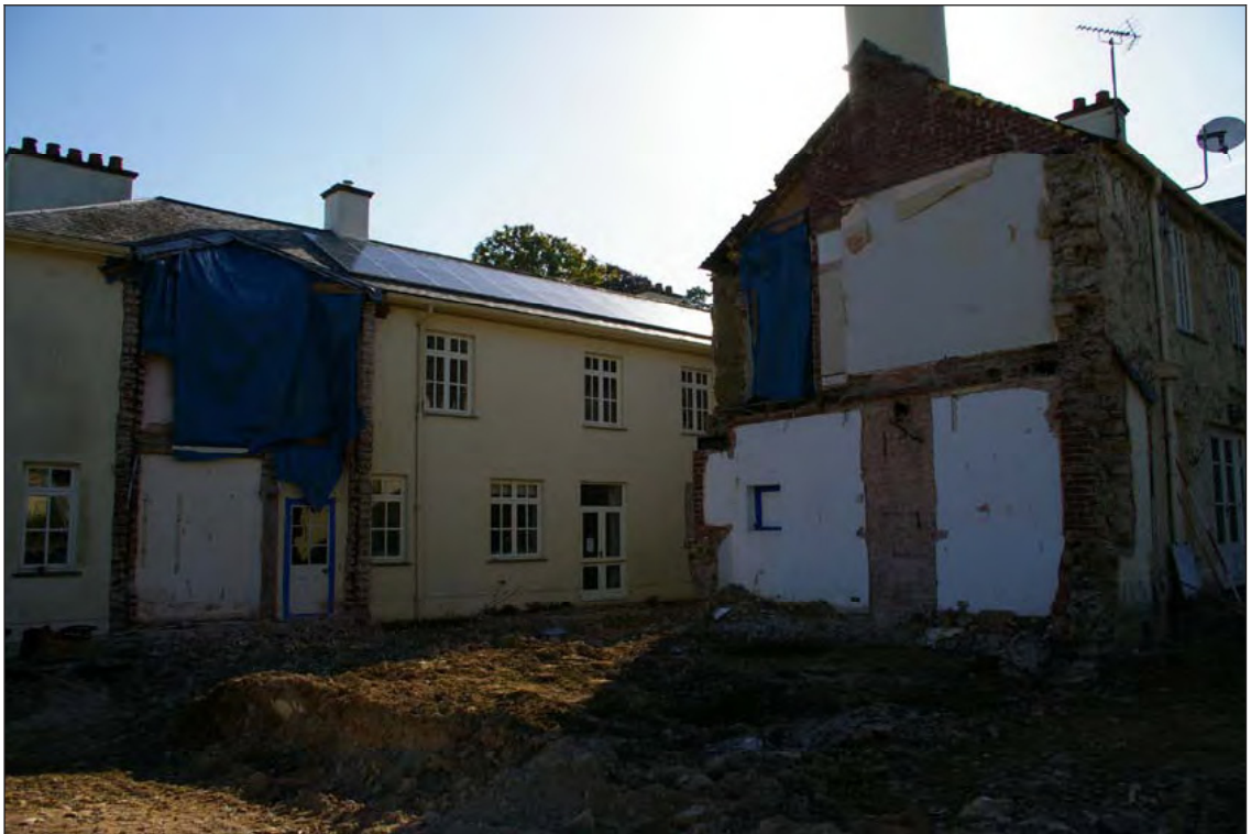
Figure 14: Fishleigh House, following the demolition of the wing and 20 th century extension, viewed from the north-west.
