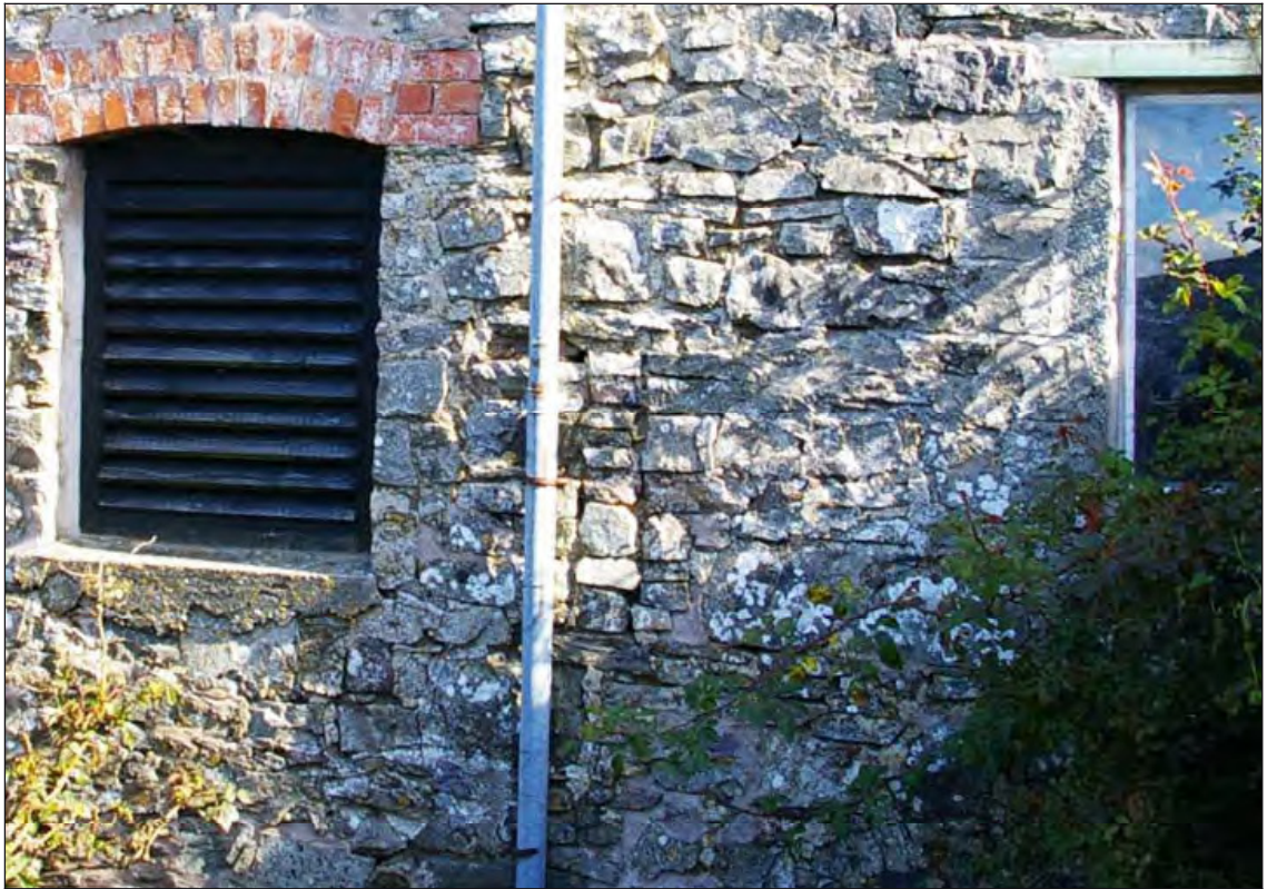
Figure 12: Detail of the slit air-vent in the west elevation of Shippon no. 2, viewed from the west.
