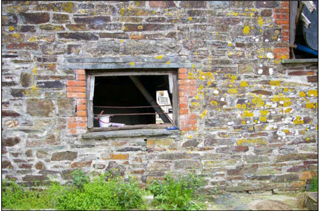
Figure 6: Ground-floor opening to the west of the south elevation, with a double slate slab lintel.
