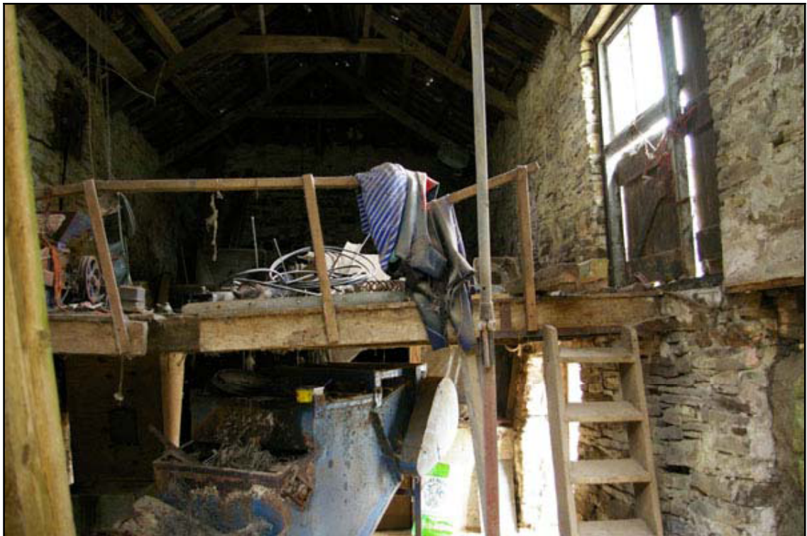
Figure 12: Internal view of barn from the east showing the floor and in situ machinery.
