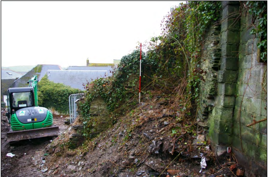
Figure 10: The eastern elevation of Building 5 prior to clearance and collapse (2m scale).
