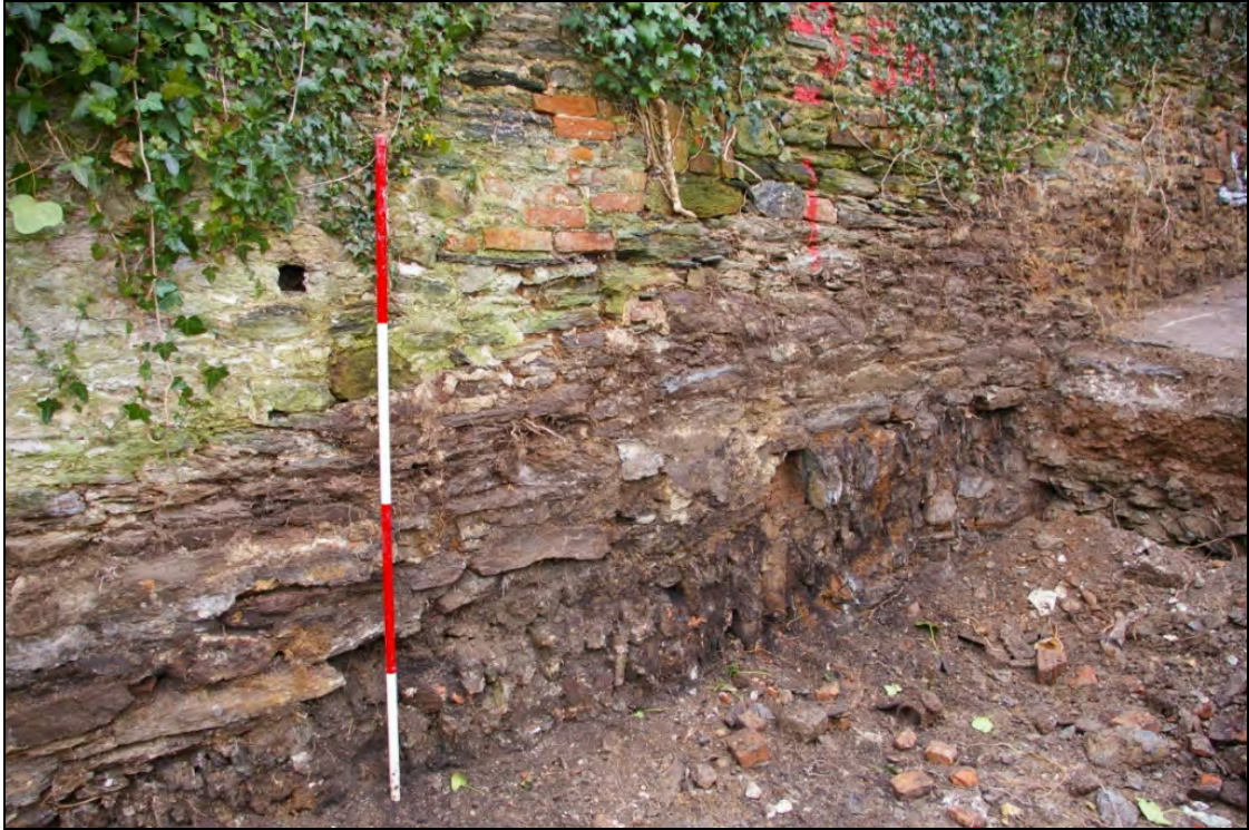
Figure 6: The blocked fireplace in the south elevation (Elevation 1) of Building 3, viewed from the north (2m scale).
