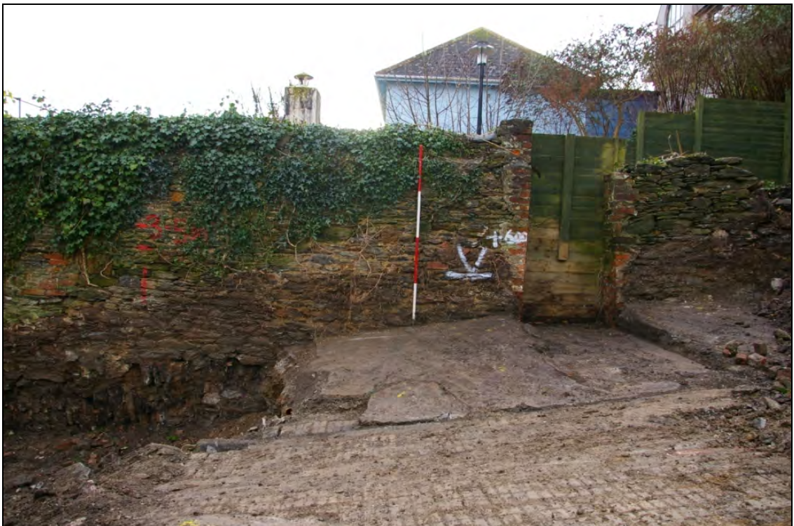
Figure 7: Forced entrance inserted in the south elevation (Elevation 1) of Building 3 leading onto Fountains Ope (formerly Allen's Yard), viewed from the north-west (2m scale).
