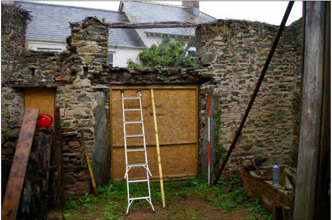
Figure 12: The internal elevation of the north wall, showing the two orthostats flanking the door (D2). Viewed from the south (scale 2m).
