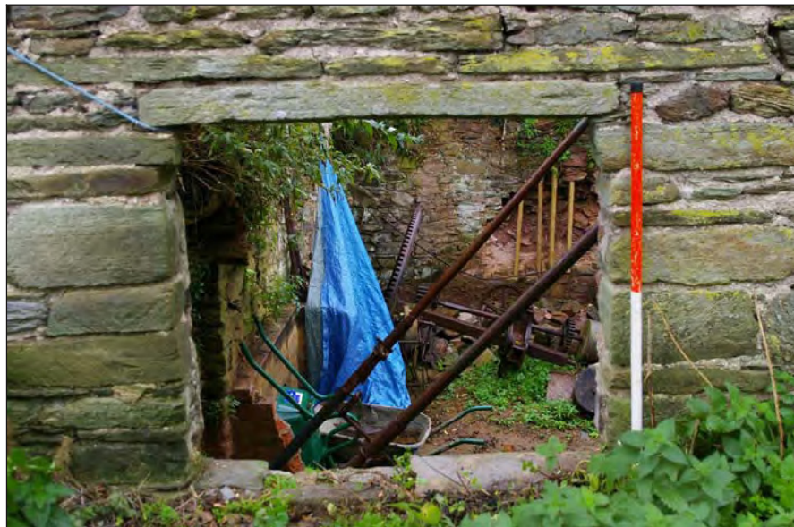
Figure 8: The window (W4) in the external east elevation, viewed from the east. Note the dressed stonework around the jambs and lintel (scale 1m).
