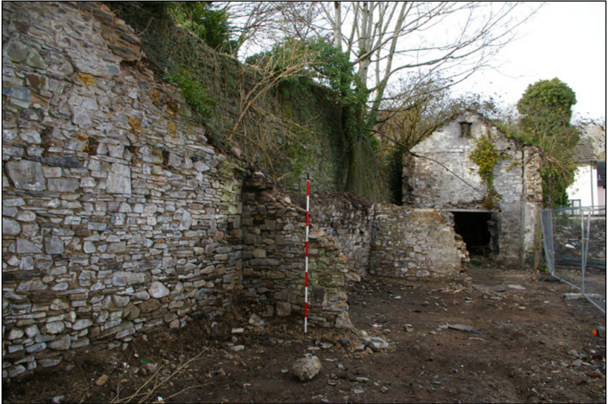
Figure 11: The remaining masonry of the rear (south-west) walls & dividing walls of B3, B4 & B5, with the north-west gable of B6 viewed from the east (2m scale).
