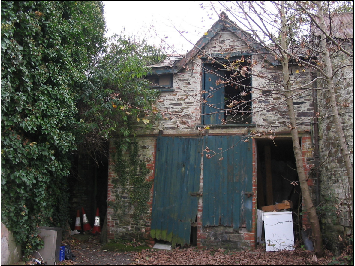
Figure 8: The Former stable at the south-east of the range (B2), viewed from the east. (Courtesy Bill Walton)
