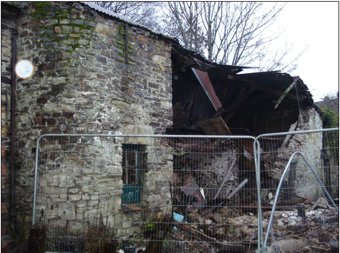
Figure 7: The buildings formerly in the centre of the range (B3 & B4), partially collapsed, viewed from the south-east. (Courtesy Bill Walton)
