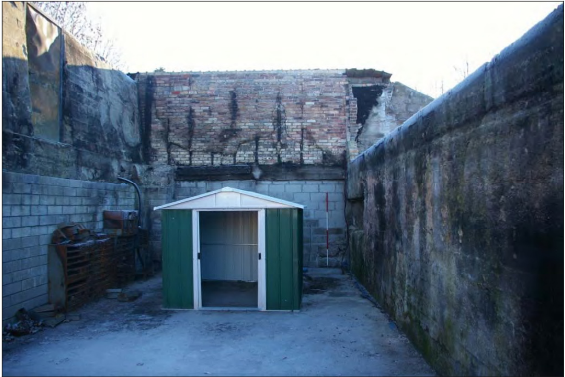
Figure 17: North-western exterior wall of the furnace house, viewed from the north-west (Scale: 2m).
