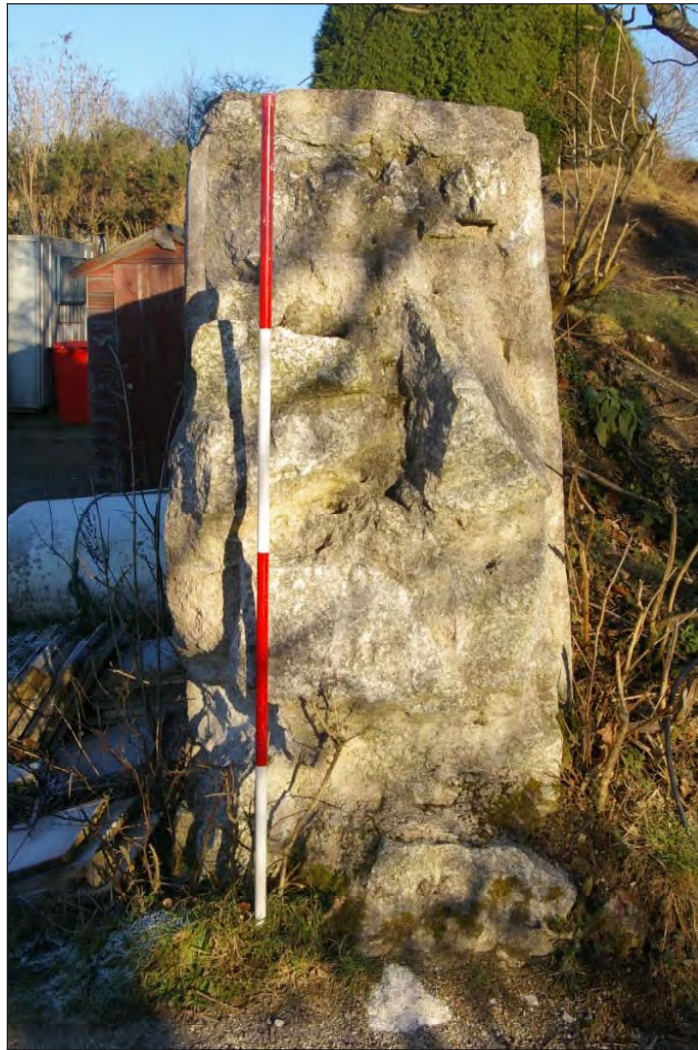
Figure 9: Section through the south-eastern wall of settling tank 8 (see Figure 2) showing the shuttered concrete and granite rubble construction (Scale 2m).
