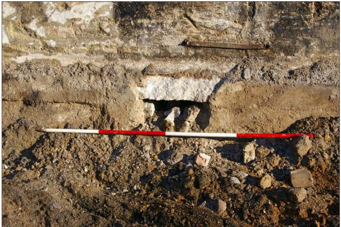
Figure 13: Culvert for carrying the waste water from the settling tanks under the linhay and drying pan, viewed from the south-west (Scale: 2m).
