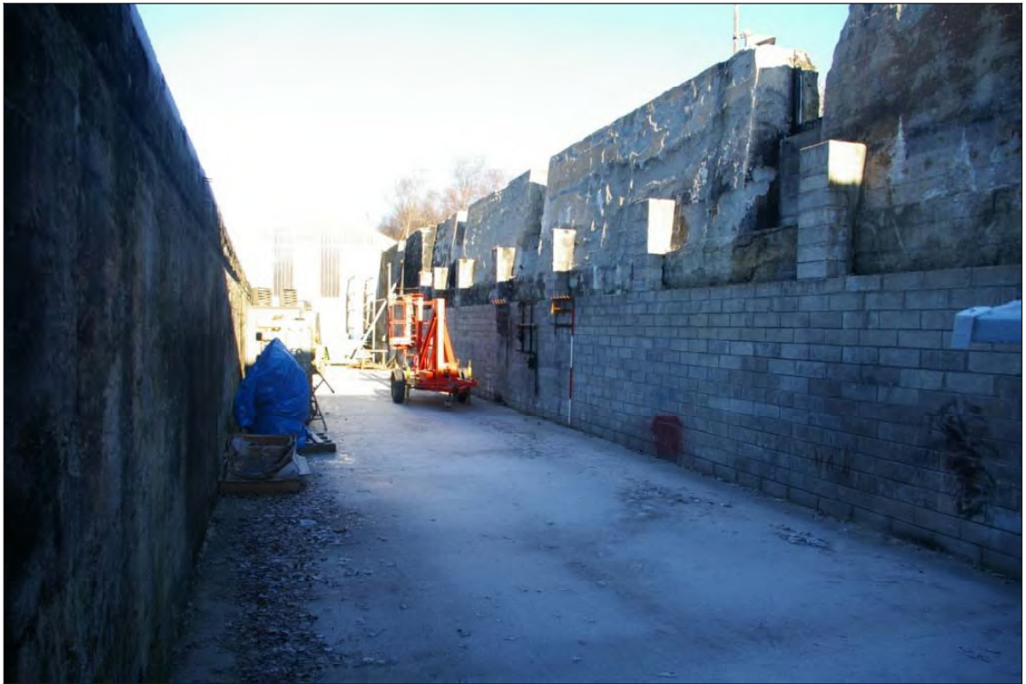
Figure 18: Junction between the Phase 1 and Phase 2 settling tanks, viewed from the south (Scale 2m).
