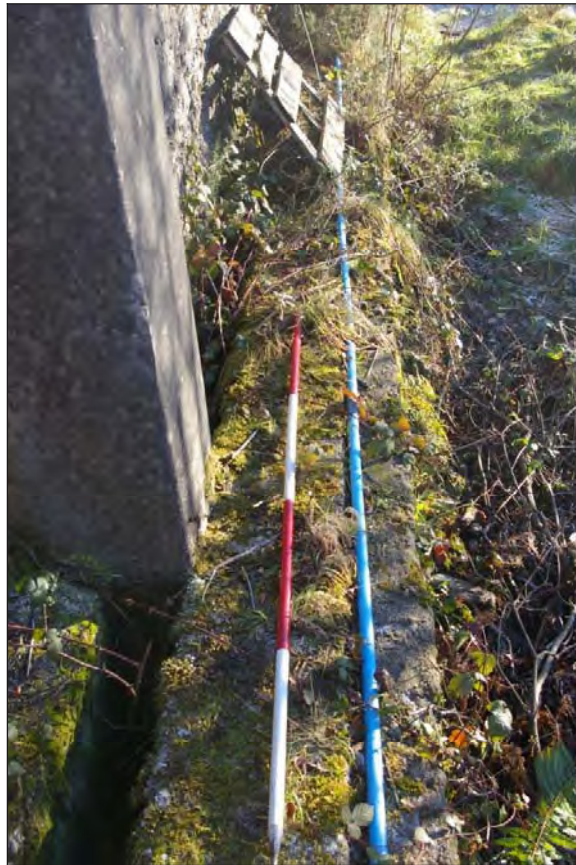
Figure 5: Dwarf wall in front of the entrance to settling tank 3 (see Fig. 2) carrying the waste water channel, viewed from the north-west (Scale: 2m).
